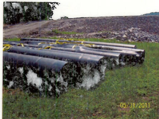
HDPE Liner On-Site for Ash Pond No. 4 Conformance Samples Taken While Stockpiled and All Materials were Approved
