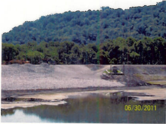
Placing 18" of Class 2 Channel Lining Ontop of #11 Stone at Ash Pond No. 4
