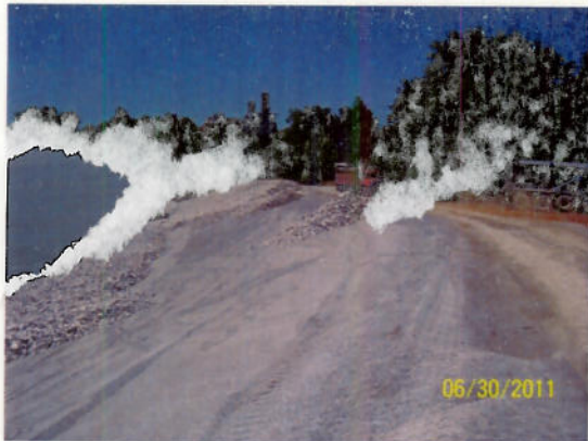
Placing 18" of Class 2 Channel Lining Ontop of #11 Stone at Ash Pond No. 4
