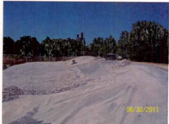
Placing 18" of Class 2 Channel Lining Ontop of #11 Stone at Ash Pond No. 4
