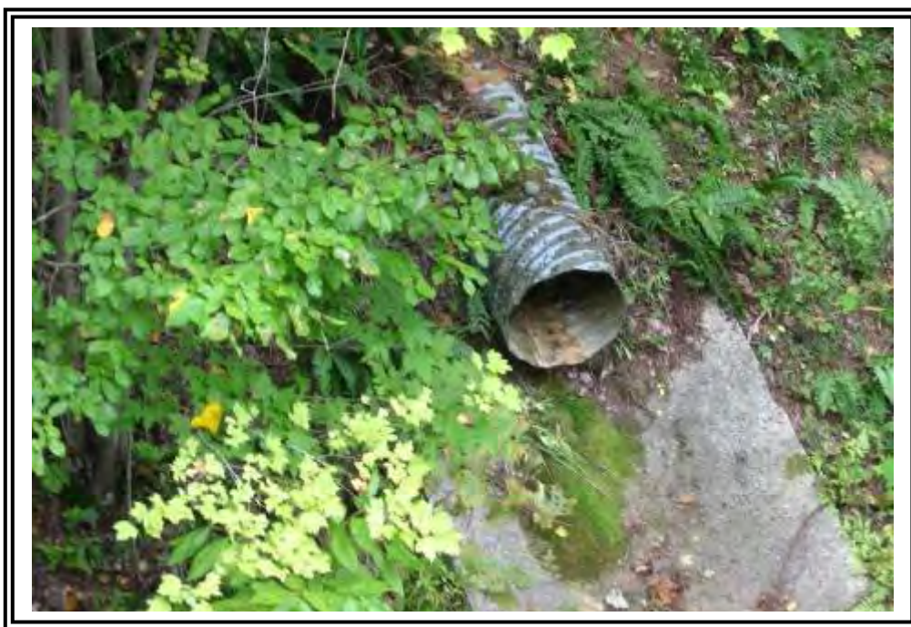
Abandoned outfall pipe.
