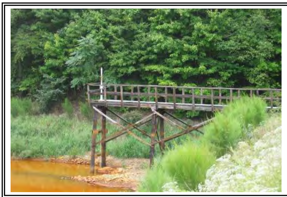
Chemical washdown dike gauge station.
