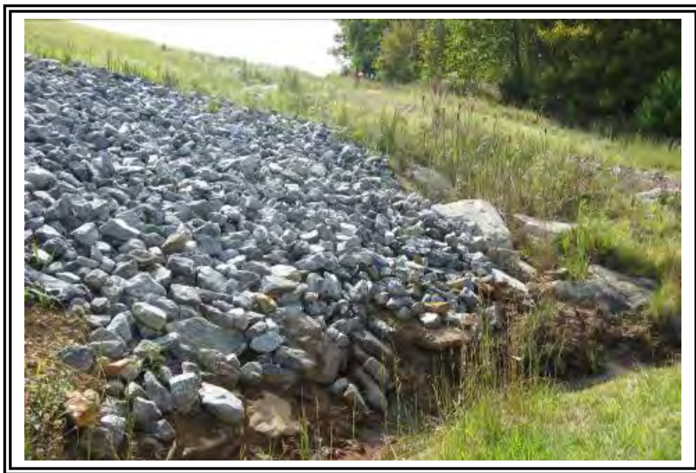
Rip rap repair and seepage area.
