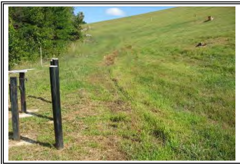
Wet rutted area.
