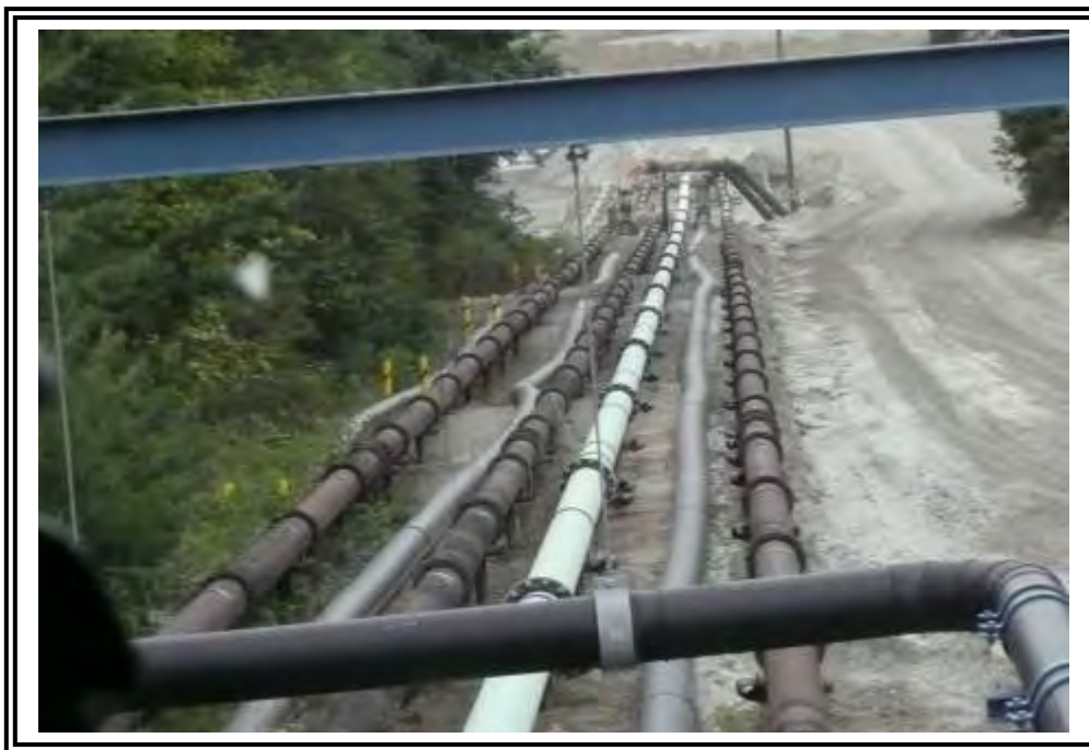
Sluice pipe lines to Ash Pond.
