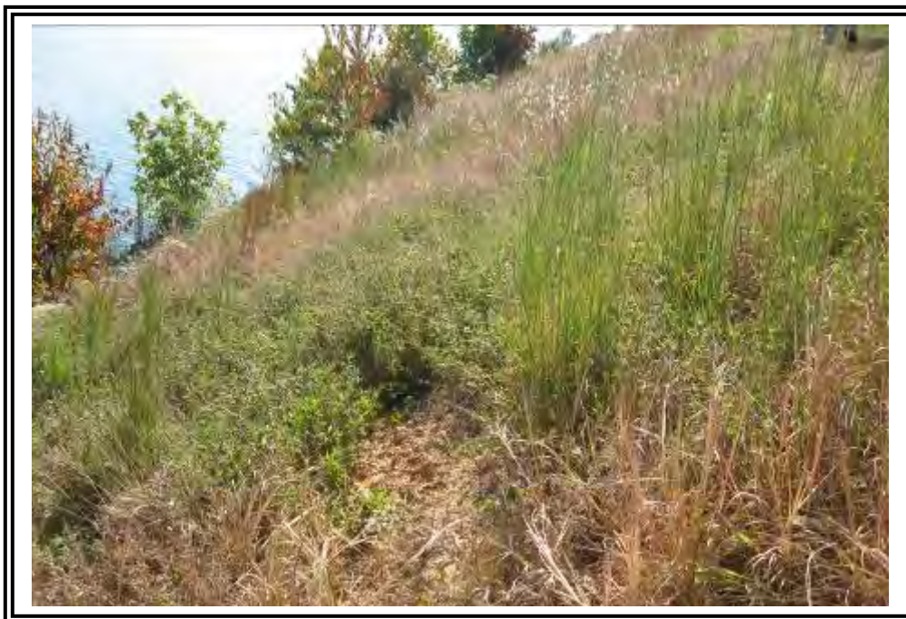
Upstream face erosion on ash dike.
