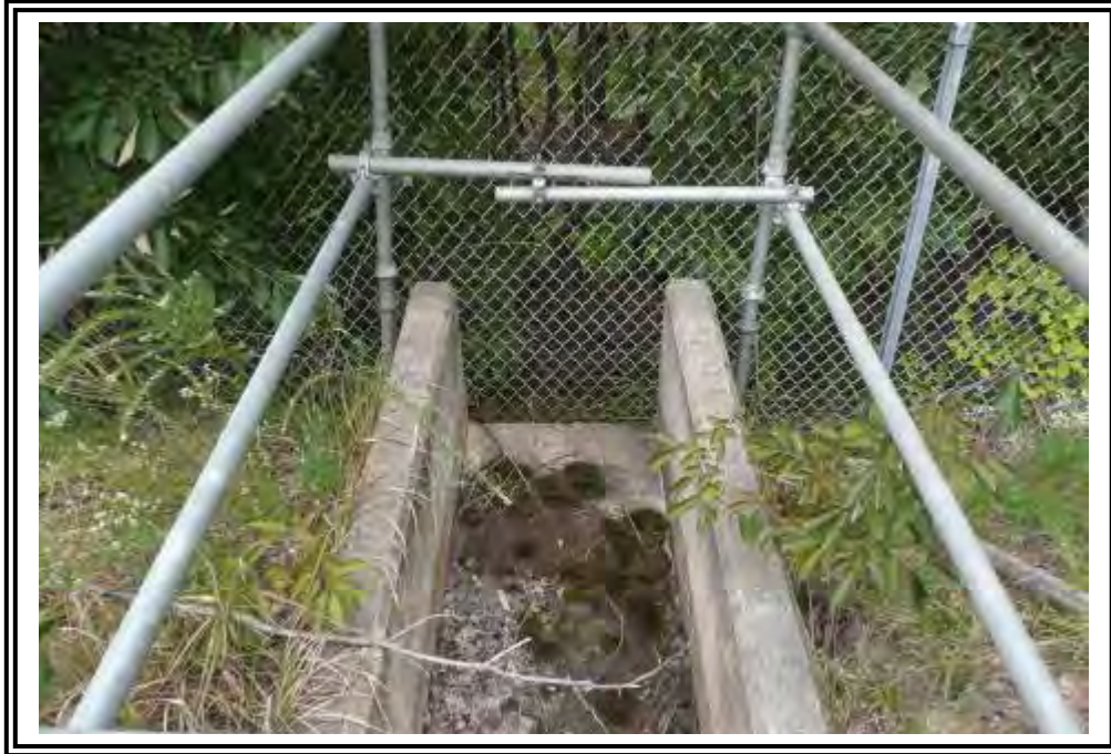
Chemical washdown pond overflow structure.
