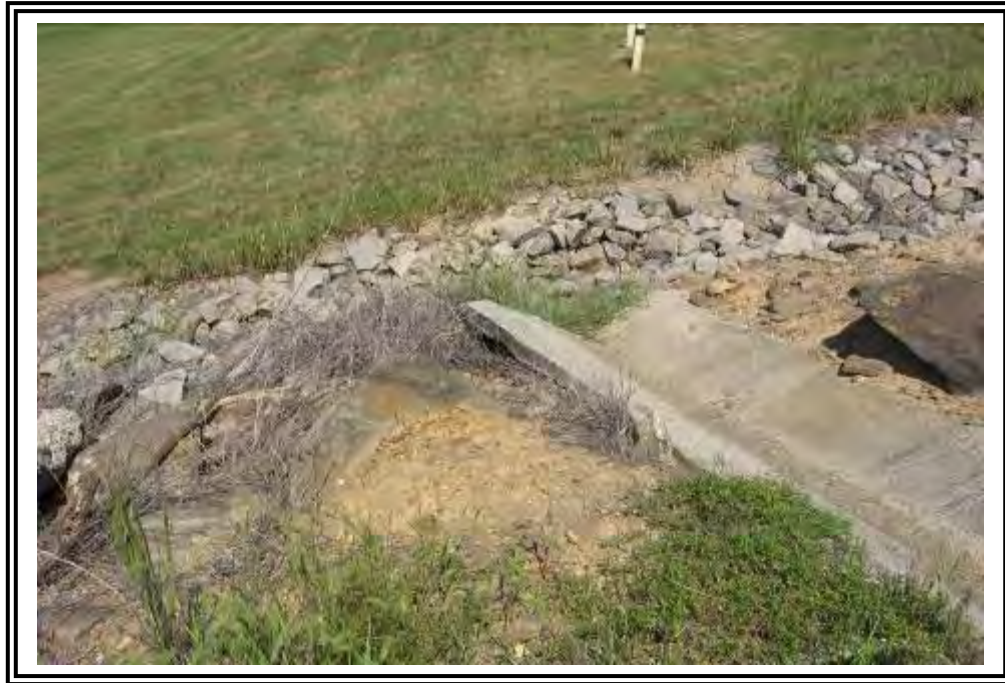
Drainage structure at east groin, undermined of chute.
