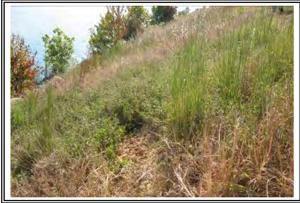
Upstream face erosion on ash dike.
