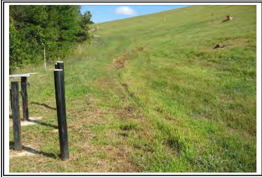
Wet rutted area.
