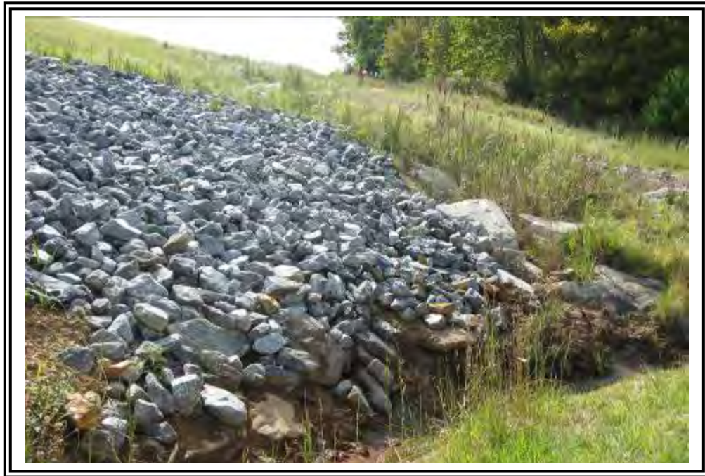
Rip rap repair and seepage area.
