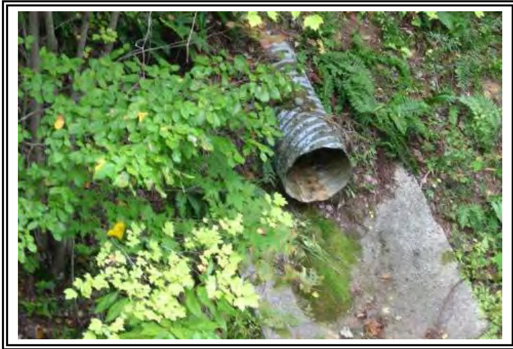
Abandoned outfall pipe.
