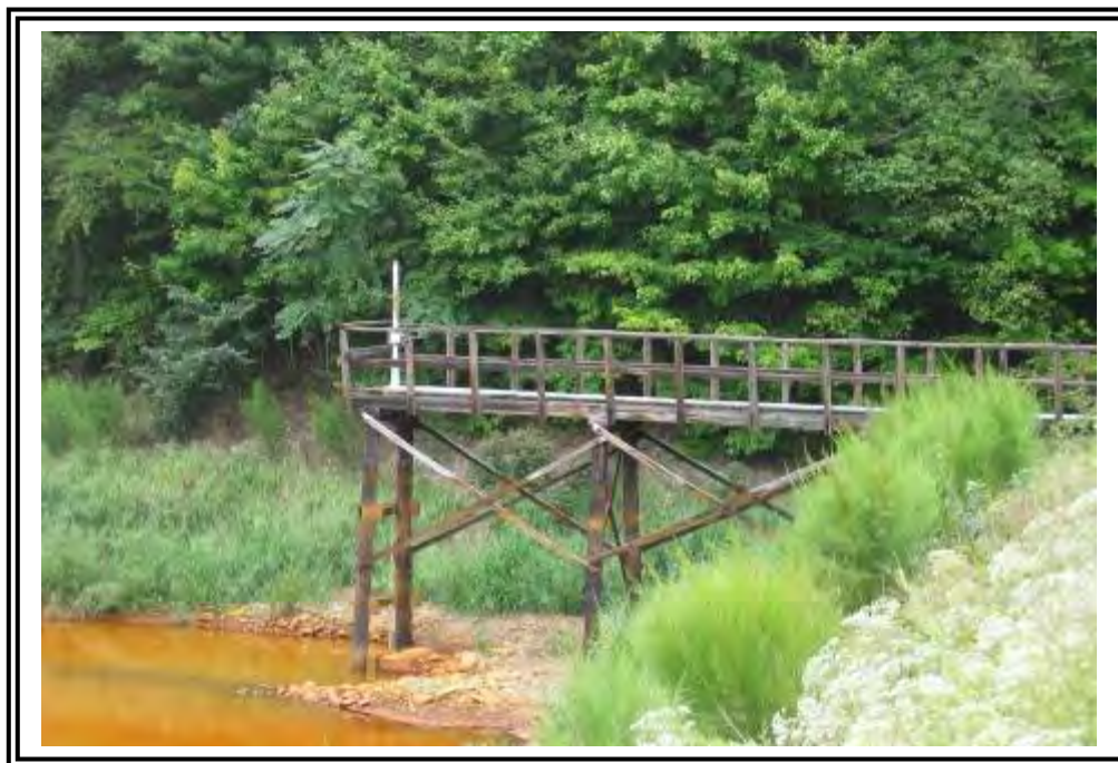
Chemical washdown dike gauge station.
