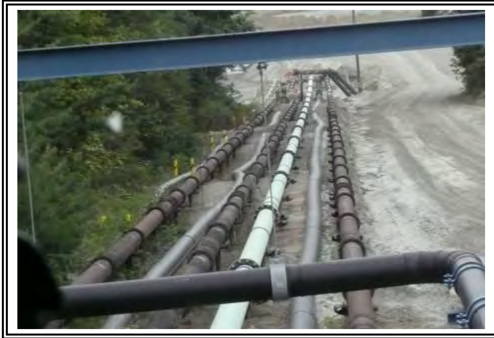
Sluice pipe lines to Ash Pond.
