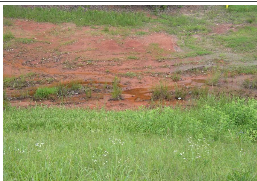
#67 Erosion at Downstream Slope of North Dike
