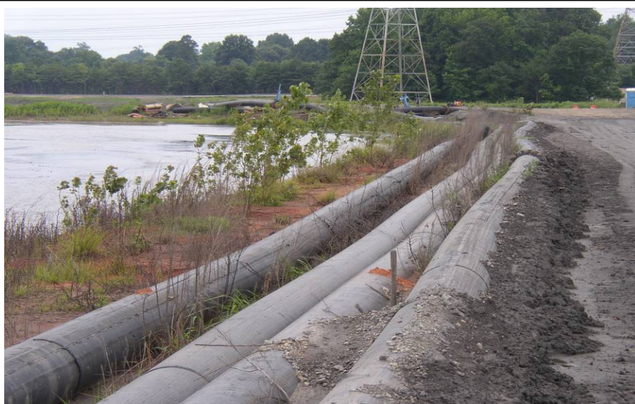
#50 Pipes Used for Sluicing
