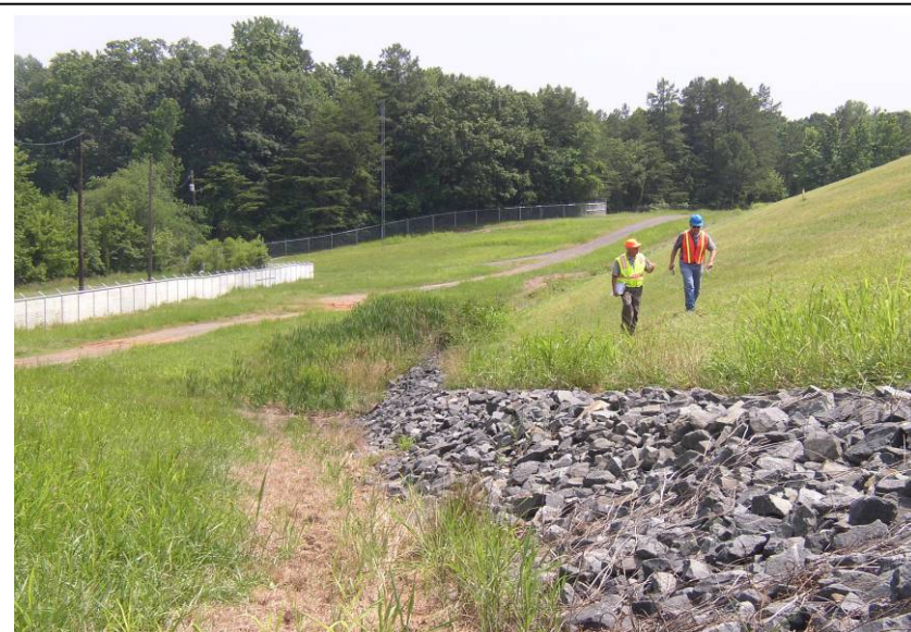
#37 Seepage Area Near Maximum Section of East Dike
