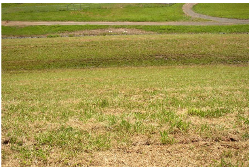
#8 Pooled Water on Bench of Downstream Stability Berm of East Dike
