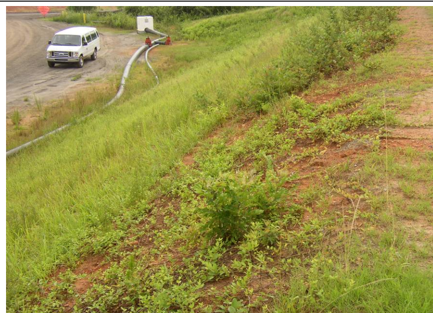
#66 Local Erosion Near Crest of North Dike
