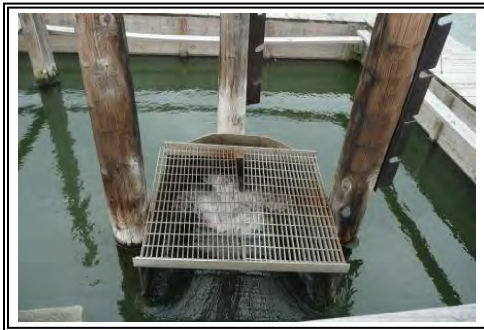
Ash Pond B overflow.
