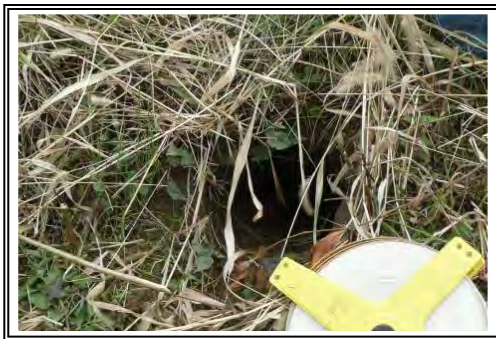
Rodent hole (typical).
