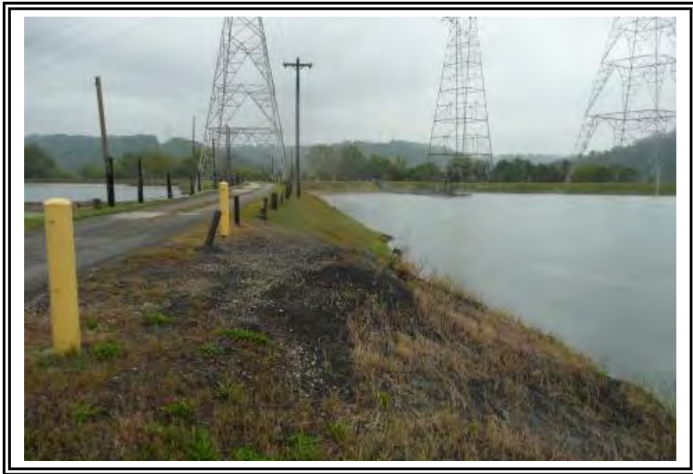
Loss of vegetation and erosion on Interior Dike.
