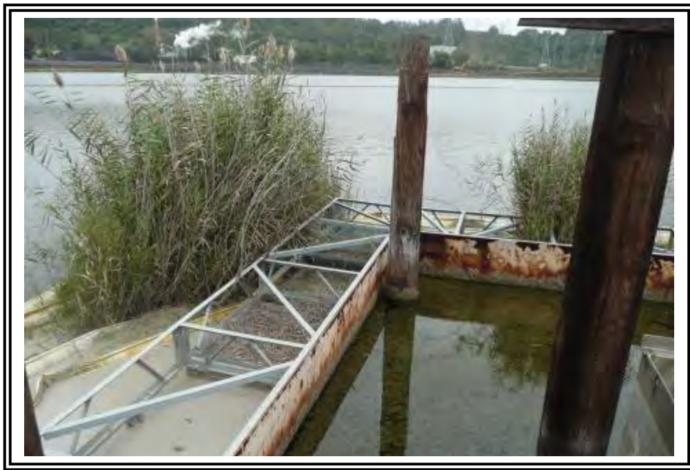
Vegetation build-up at Ash Pond A overflow structure.
