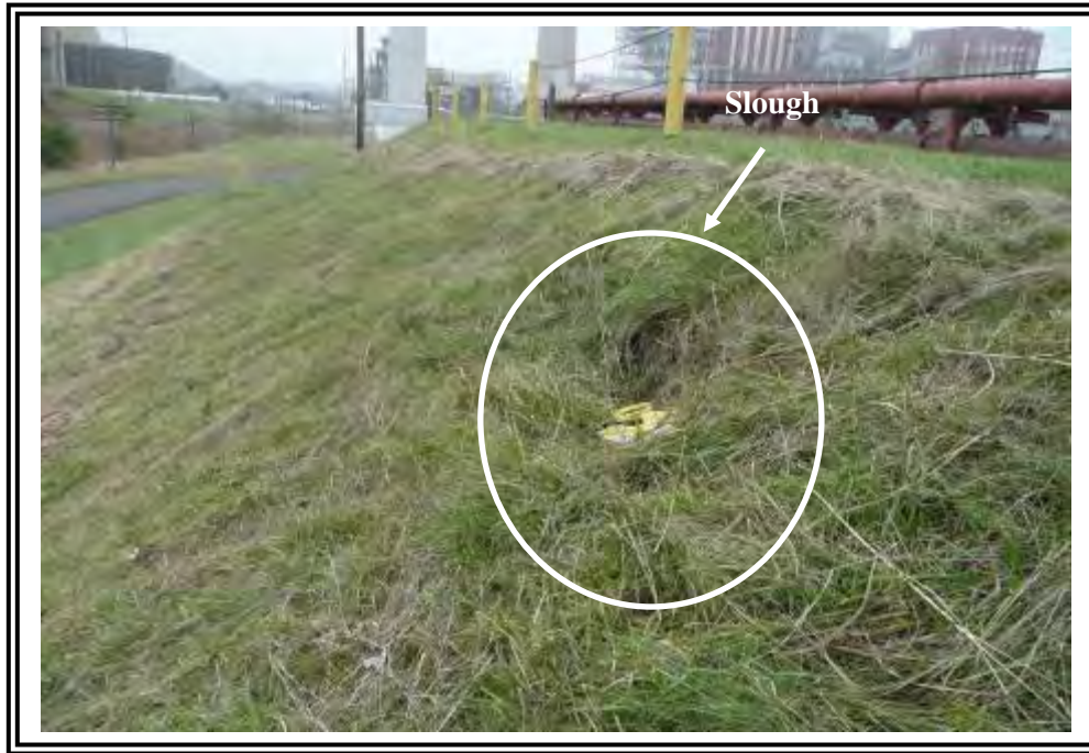
Ash Pond A slope slough, north slope.
