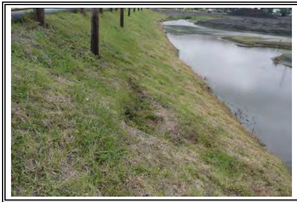
Sloughing along Interior Dike, Ash Pond A.
