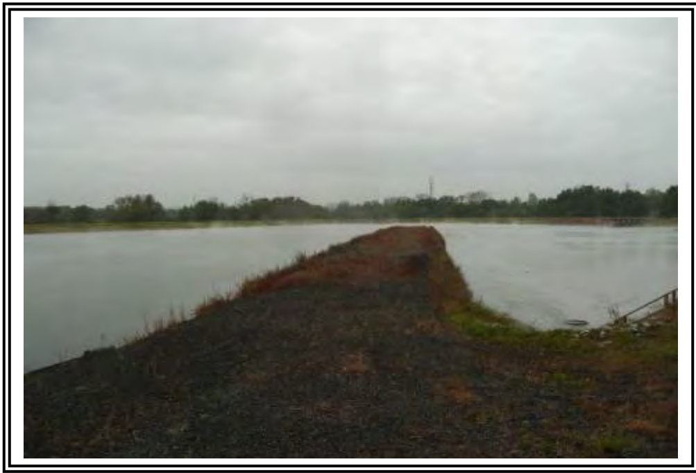
Interior groin in Ash Dike B. Feature not shown on plans.
