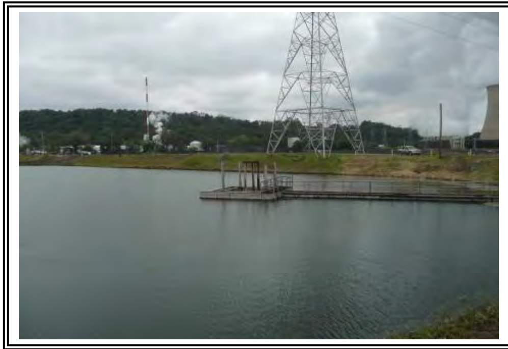
Ash Pond B overflow.
