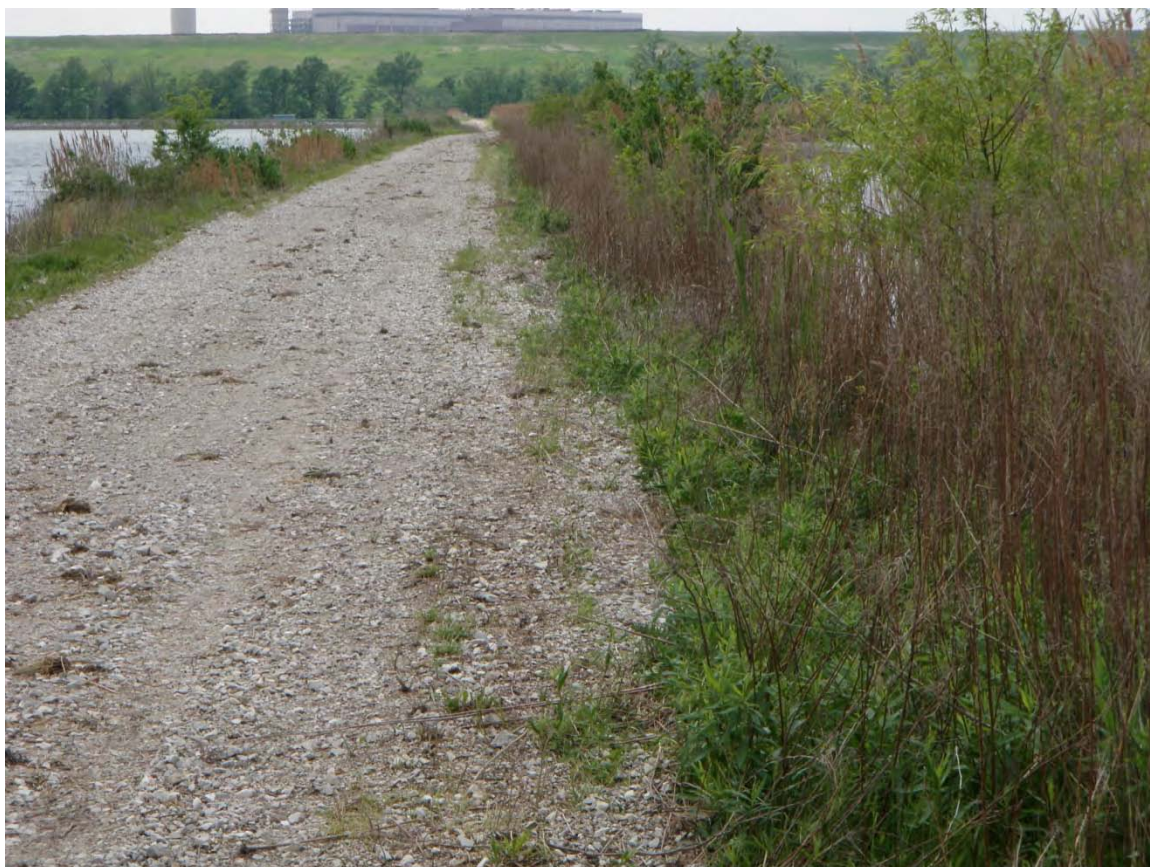
Photo 12: East Ash Pond #1 – Interior dike crest between EAP #1 and Settling Basin, looking west, notice several small trees.
