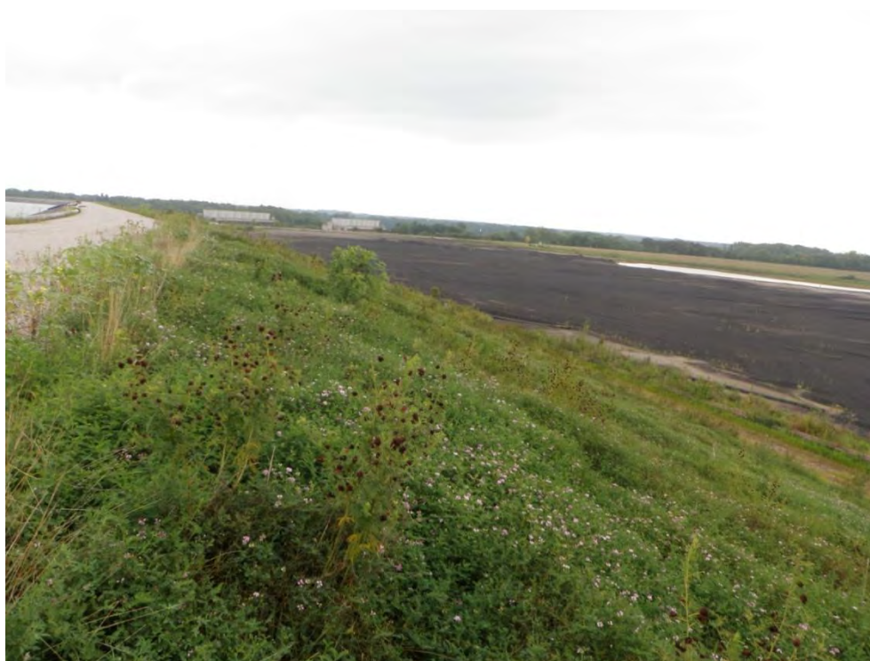
Photo 11: Ash Disposal Area #1 – West dike upstream slope (divider dike with Lined Ash Disposal Pond – Cell #1), looking north
