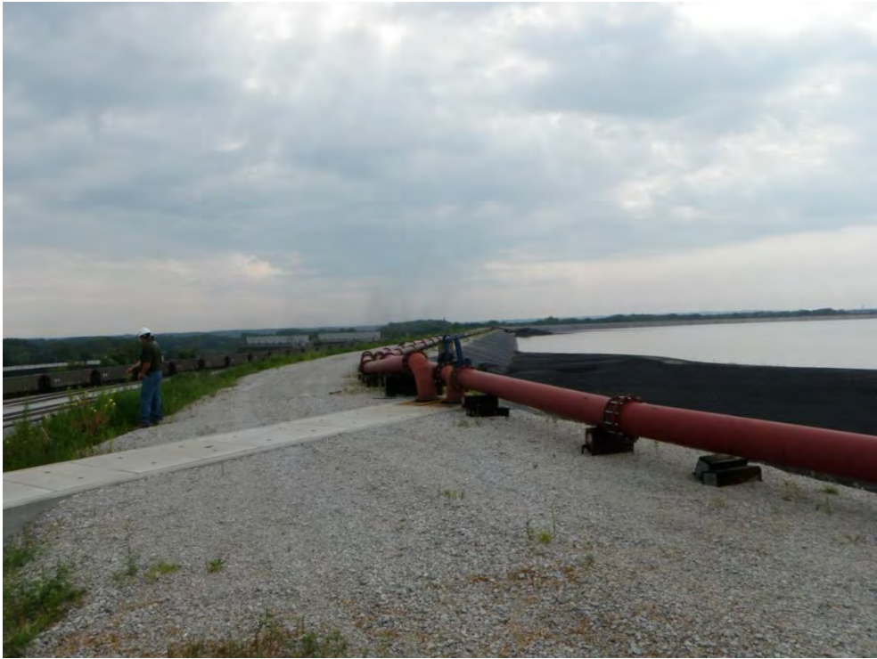
Photo 1: Lined Ash Disposal Pond – Cell #1 - North dike upstream slope and crest, looking east
