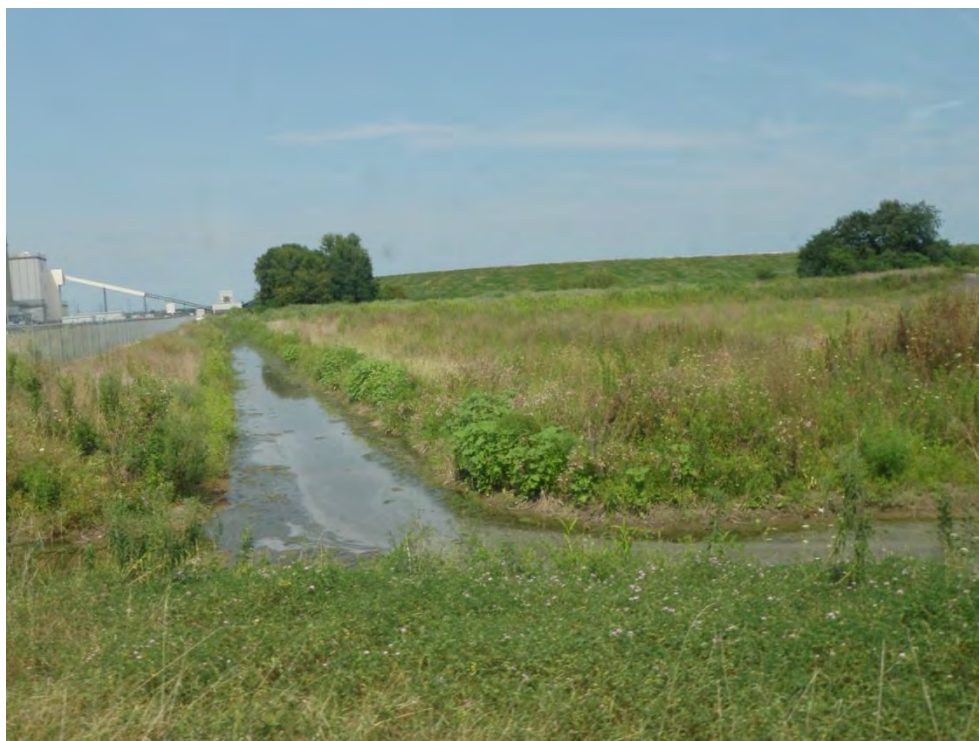
Photo 42: Lined Ash Disposal Pond – Cell #1 – South dike downstream slope and drainage ditch, looking north
