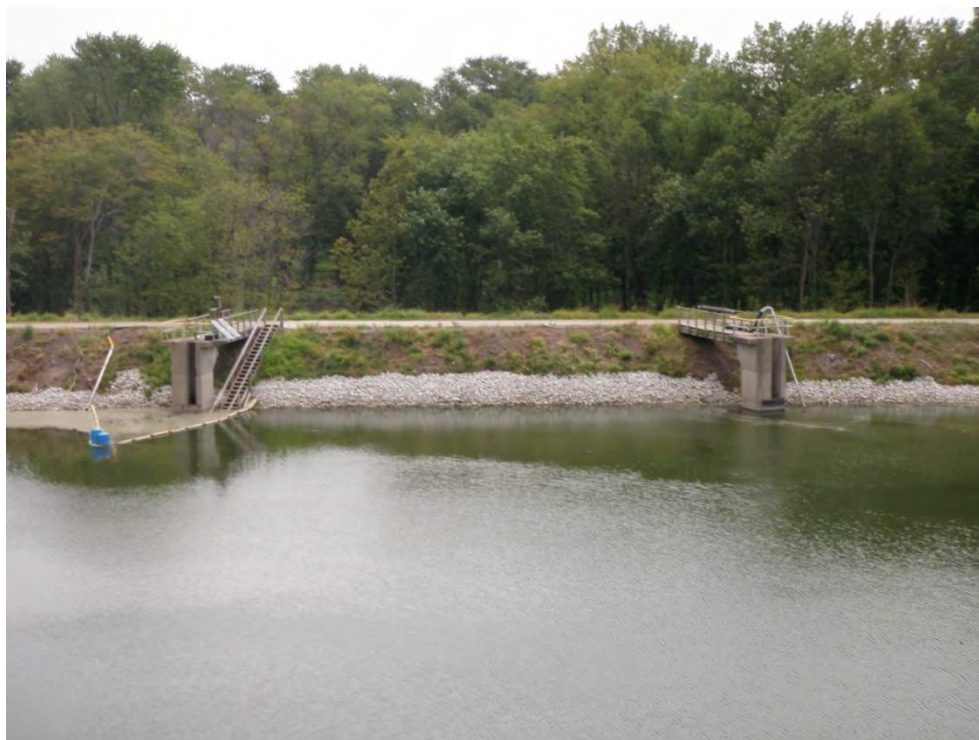
Photo 31: Secondary Ash Settling Pond – East dike upstream slope, Intake structure weir #3 and #4, looking east
