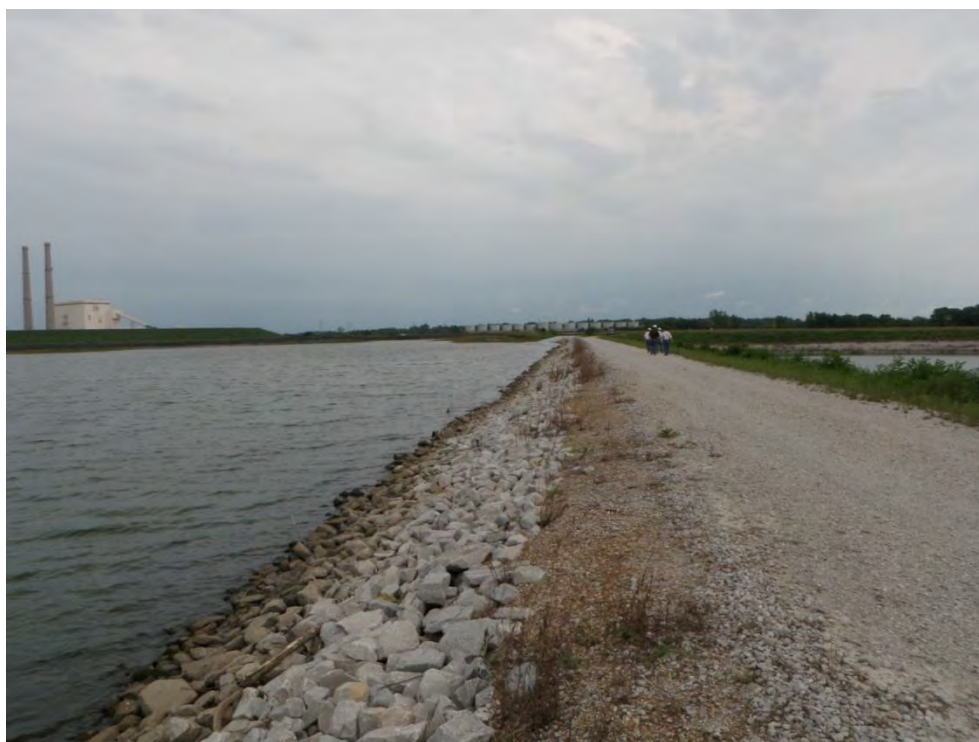
Photo 22: Ash Disposal Area #1 – East dike upstream slope (divider dike with Primary Ash Settling Pond), looking north
