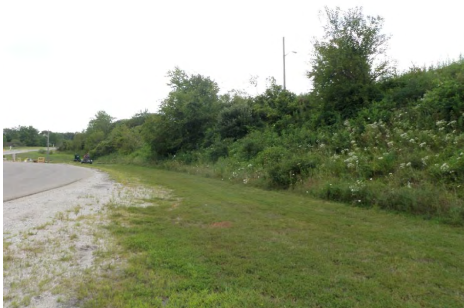
Photo 40: Original Ash Pond – North dike downstream slope, note trees, looking east
