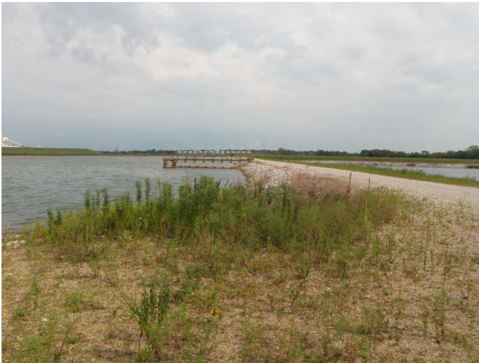
Photo 16: Ash Disposal Area #1 – East dike upstream slope (divider dike with Primary Ash Settling Pond), looking north
