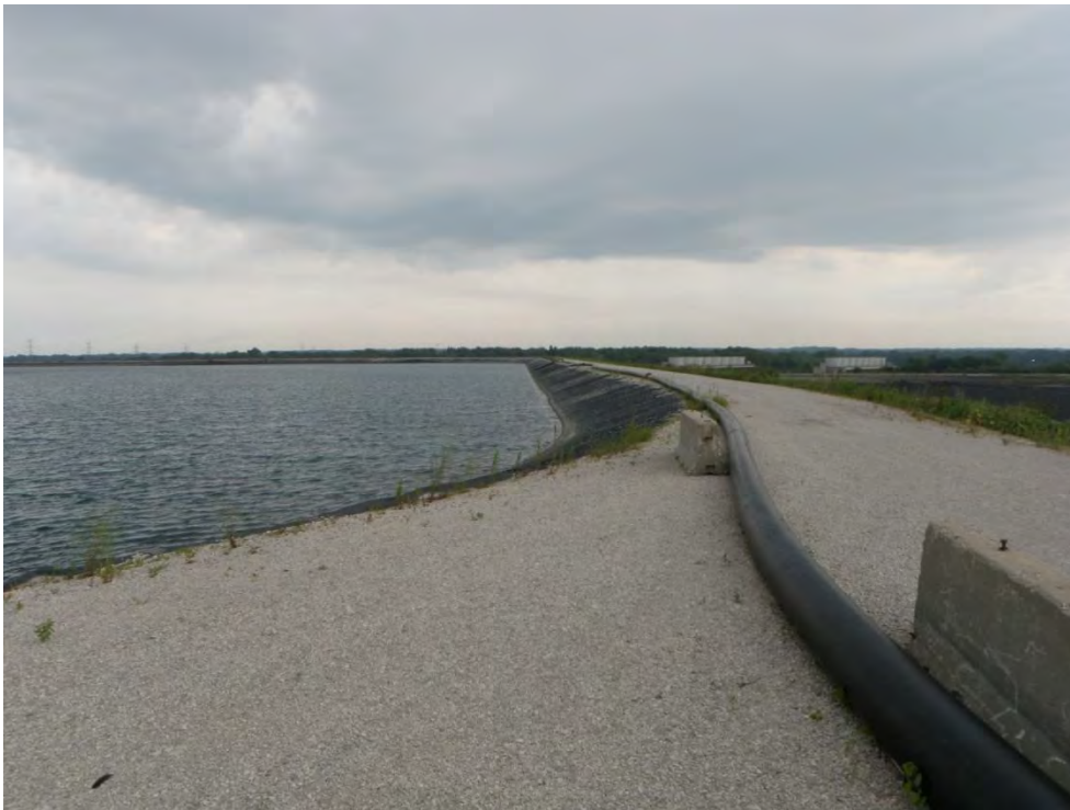
Photo 10: Lined Ash Disposal Pond – Cell #1 – East dike upstream slope (divider dike with Ash Disposal Area #1), looking north
