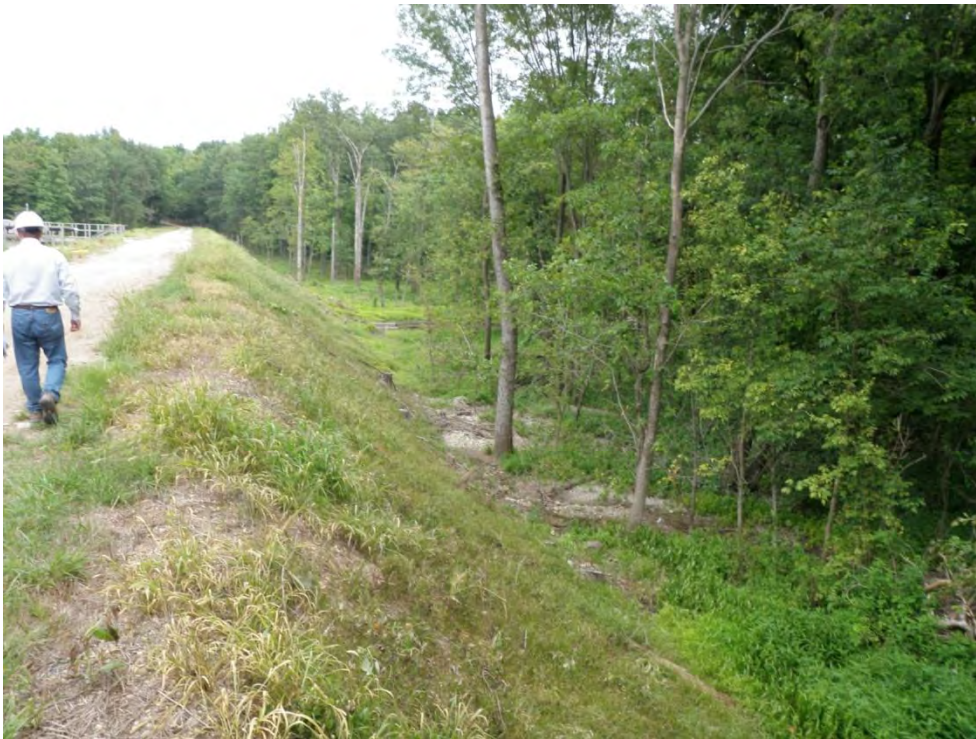
Photo 34: Secondary Ash Settling Basin – East dike downstream slope, note trees within 25' of dam toe, looking north
