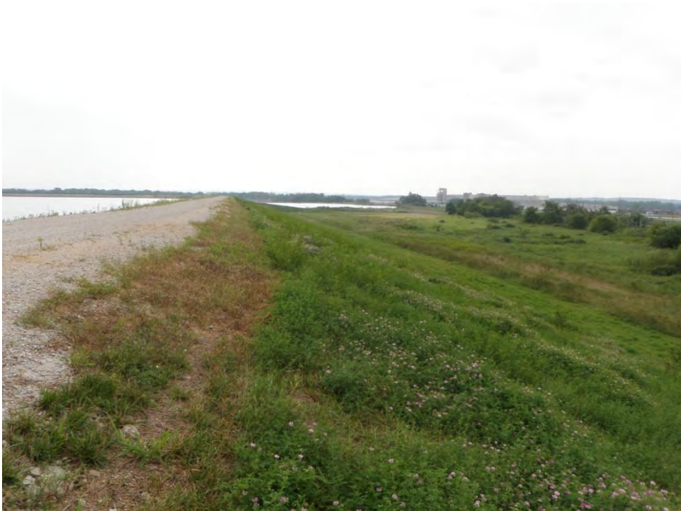
Photo 8: Lined Ash Disposal Pond – Cell #1 – South dike downstream slope and crest, looking east
