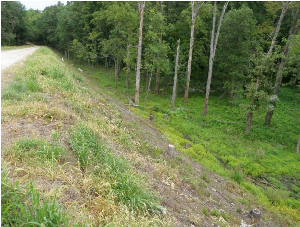
Photo 38: Secondary Ash Settling Basin – East dike downstream slope, note trees within 25' of dam toe, looking north
