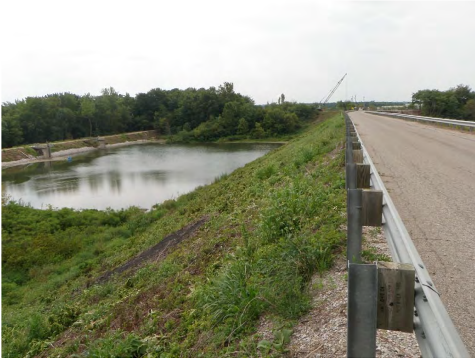
Photo 29: Secondary Ash Settling Pond – West dike upstream slope (divider dike with Primary Ash Settling Pond), note erosion, looking south
