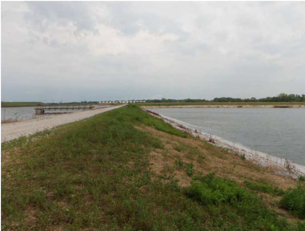
Photo 17: Primary Ash Settling Pond – West dike upstream slope (divider dike with Ash Disposal Area #1), looking north
