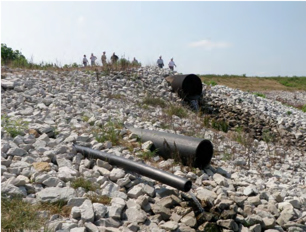
Photo 43: Primary Ash Settling Basin – Southwest corner, inlet pipes from drainage ditch, looking west
