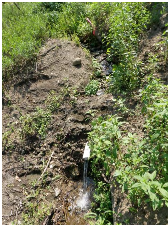
Photo 48: Ash Disposal Area #1 – Downstream of northeast dike downstream toe, note seeps / natural springs, looking southeast
