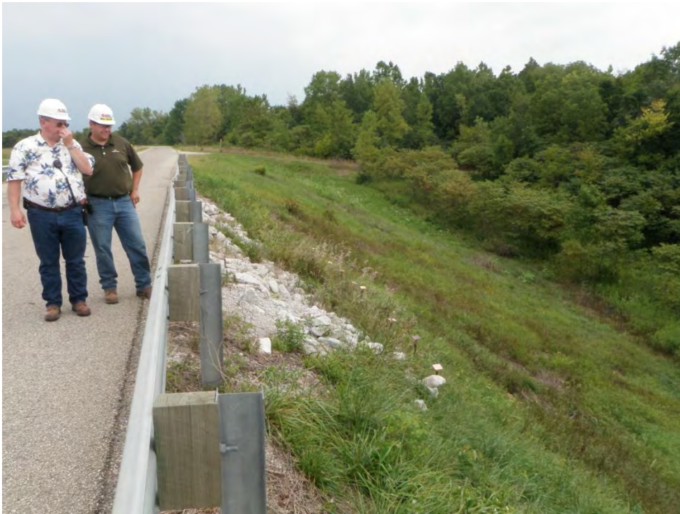
Photo 30: Secondary Ash Settling Basin – West dike upstream slope (divider dike with Primary Ash Settling Basin), note erosion, looking north
