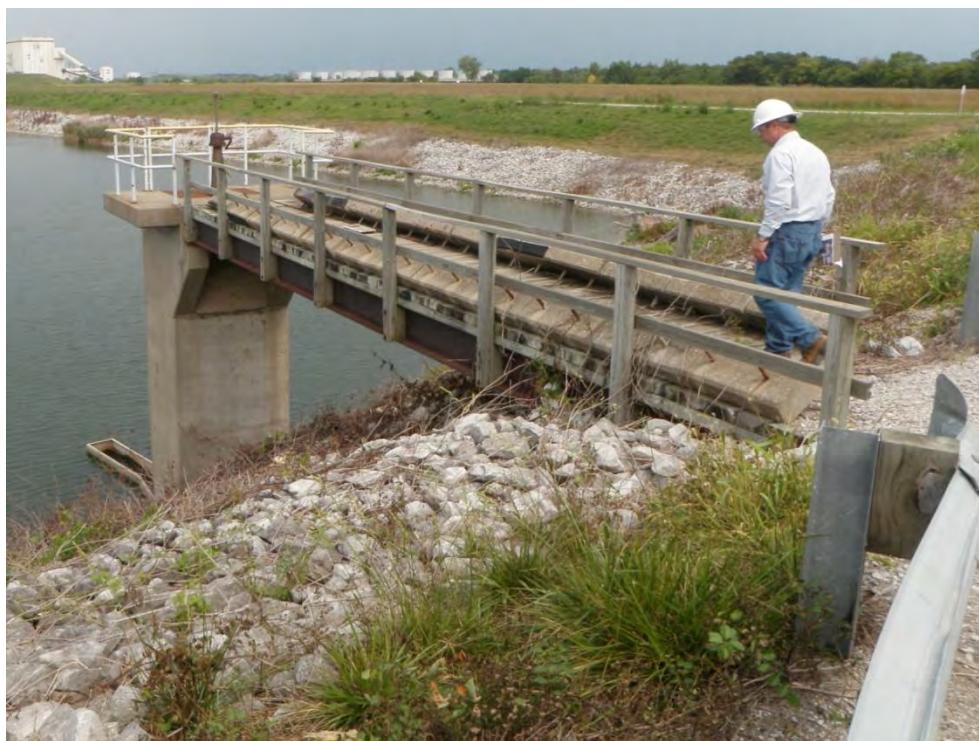
Photo 24: Primary Ash Settling Pond – Intake structure on west dike, concrete weir #2, looking northwest
