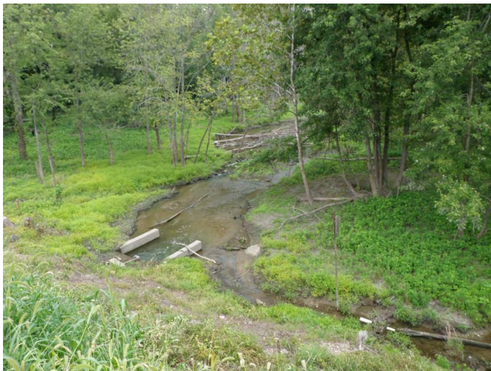
Photo 35: Secondary Ash Settling Basin – East dike downstream toe, outlet and outlet structure to Wabash River, note seepage along downstream toe of dike at right side of photo, looking northeast
