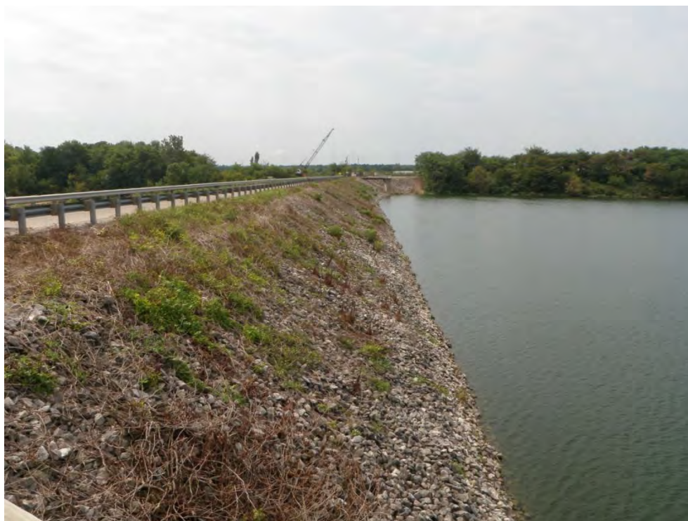
Photo 26: Primary Ash Settling Pond – East dike upstream slope (divider dike with Secondary Ash Settling Pond), looking south
