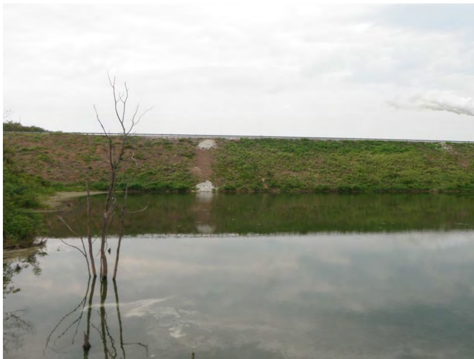
Photo 32: Secondary Ash Settling Basin – West dike upstream slope, note rip rap covering animal holes, looking west
