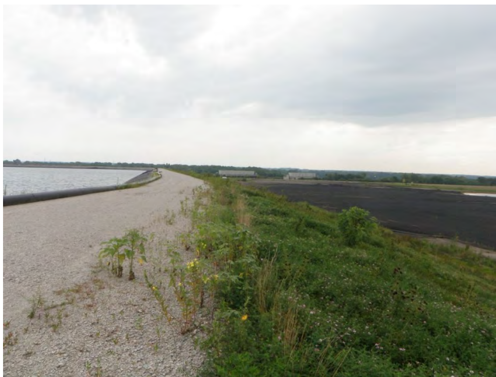
Photo 12: Divider dike between Lined Ash Disposal Pond – Cell #1 and Ash Disposal Area #1, crest, looking north
