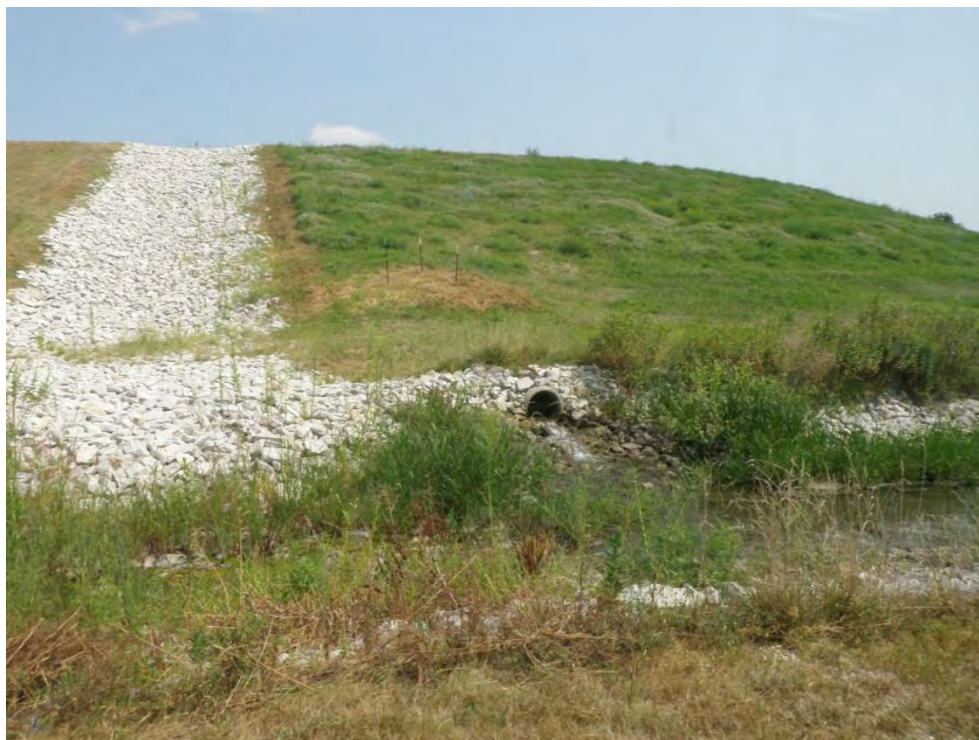
Photo 41: Lined Ash Disposal Pond – Cell #1 – Emergency spillway and outlet pipe, looking east
