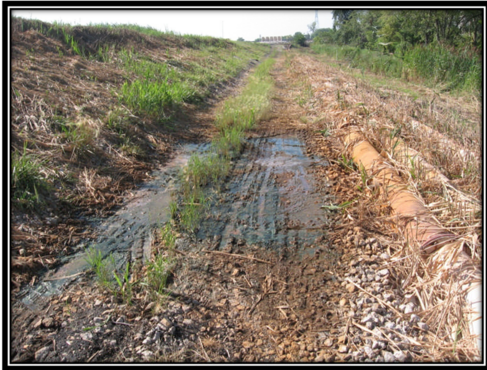
Photo 25 – Seepage Area Looking South
