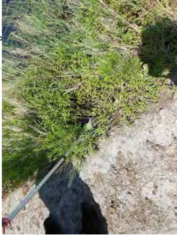
Photo 23: NP/SP - Erosion of ash material on common embankment north slope.
