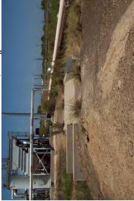
Photo 75: SP - Spillway between SRH Pond and South Bottom Ash Pond at west embankment crest, looking north.
