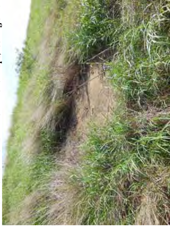
Photo 117: Exposed soil at south embankment exterior slope, looking north.
