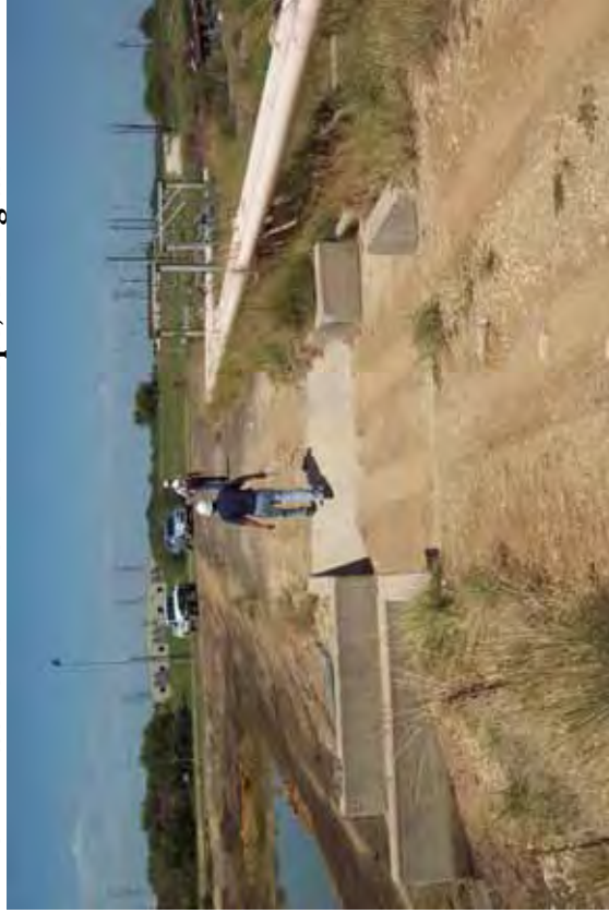
Photo 79: SP - Spillway between SRH Pond and South Bottom Ash Pond at west embankment crest, looking north.
