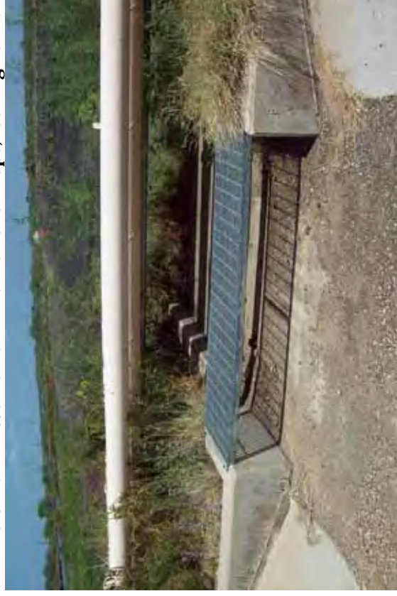
Photo 76: SP - Spillway between SRH Pond and South Bottom Ash Pond at west embankment interior slope, looking east.
