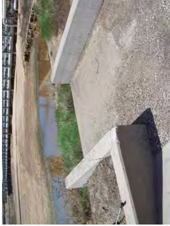
Photo 77: SP - Spillway between SRH Pond and South Bottom Ash Pond at west embankment exterior slope, looking west.
