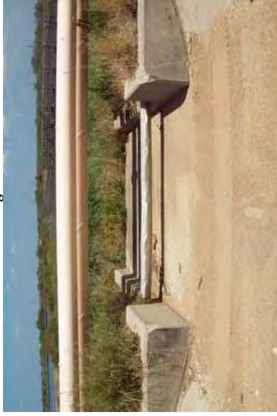
Photo 80: SP - Spillway between SRH Pond and South Bottom Ash Pond at west embankment interior slope, looking east.
