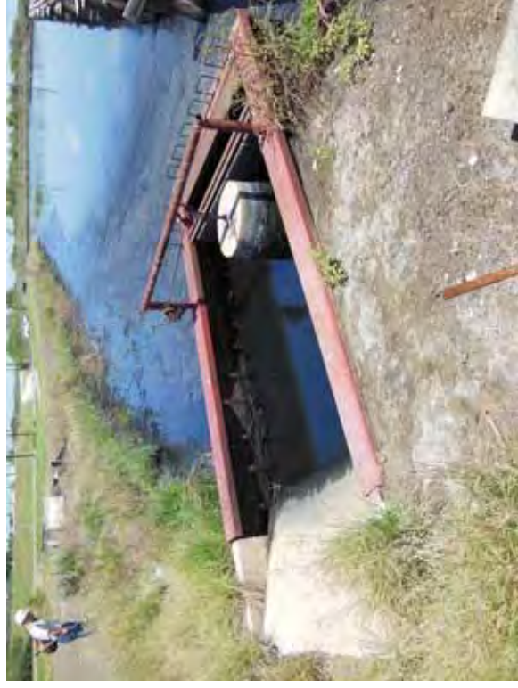
Photo 34: NP - 24-inch-diameter Plant return outlet, looking north.
