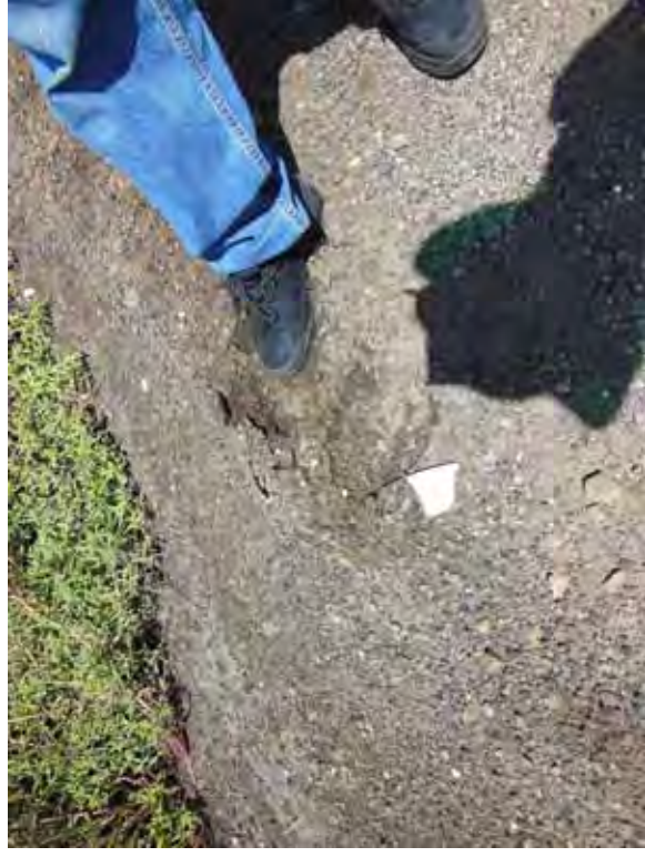
Photo 14: NP - Loose ash material at east embankment interior slope.
