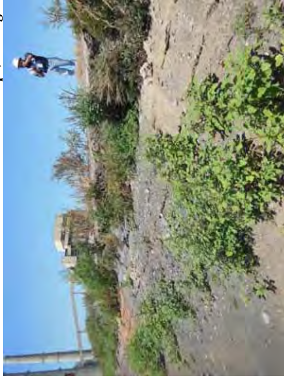
Photo 24: NP/SP - Erosion of ash material on common embankment south slope, looking northwest.
