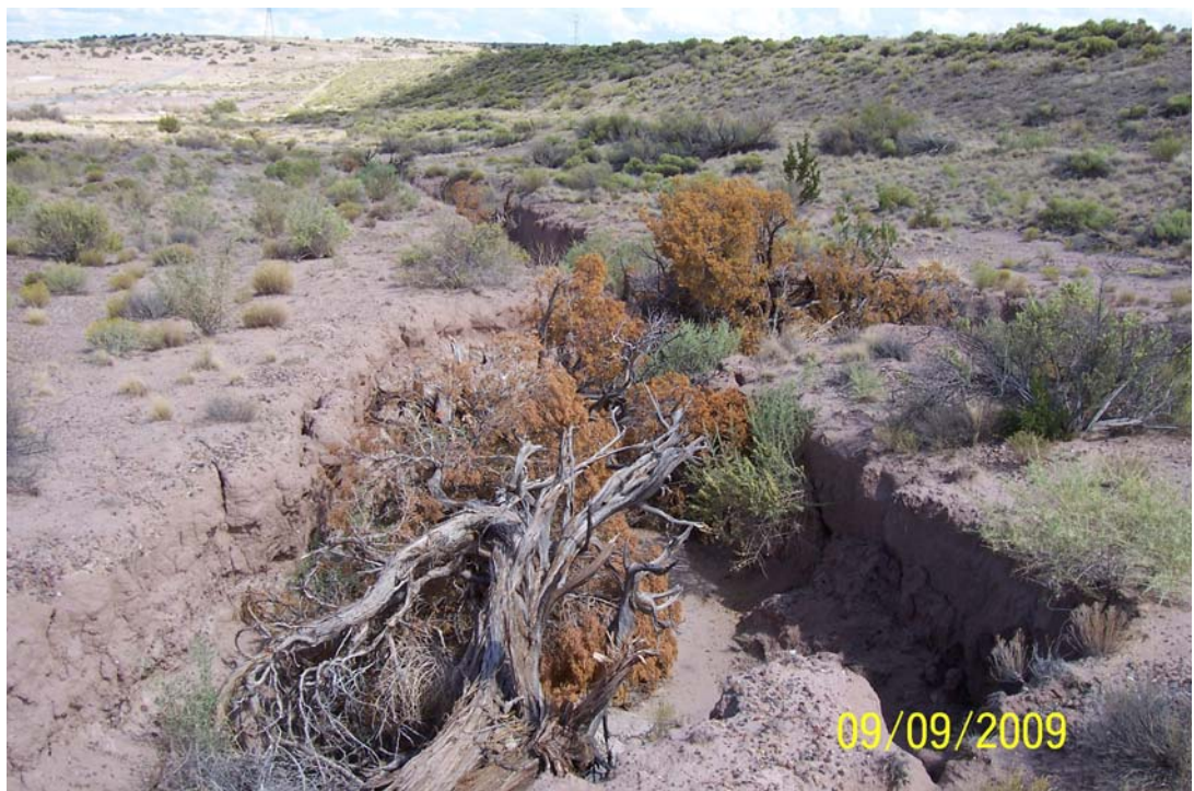
Photo 20: View of erosion gulley near left downstream toe of dam. Note woody debris placed in channel by SRP/CGS to control erosion.
