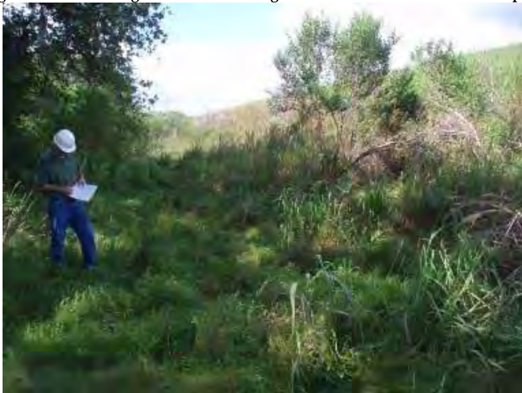
Photo No. 108: Primary Ash Pond - East embankment exterior slope, looking south at end of approximately 400-foot-long seepage area.
