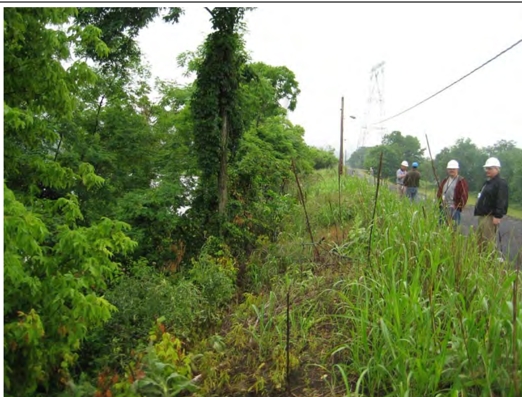
#12 - Typical Vegetative Growth on Upstream Face of Embankment
