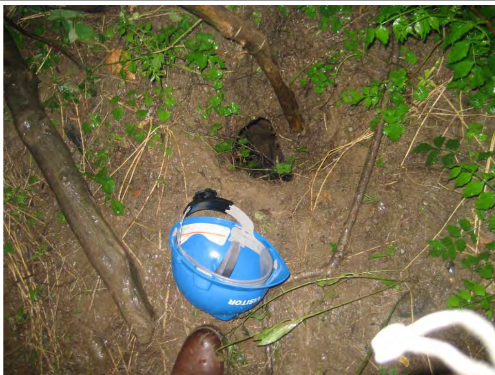
#7 - Sinkhole Above Downstream End of 36" Outlet Pipe
