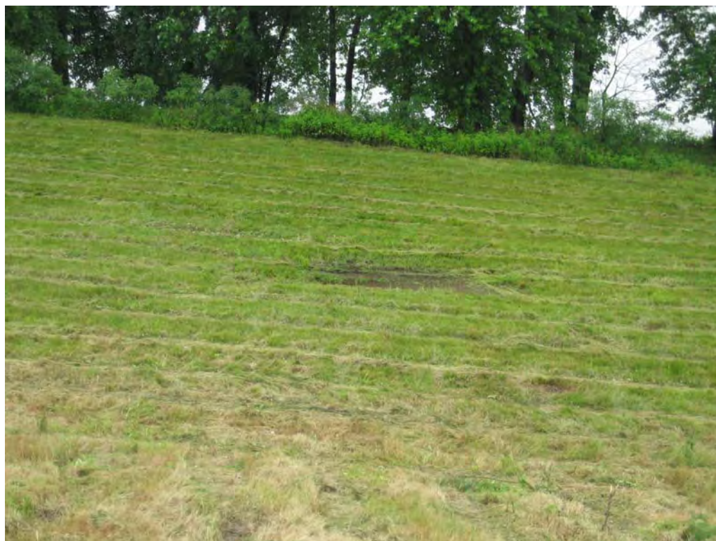
#13 - Downstream Face Along Horizontal Berm; Note Wet Area in Middle of Frame
