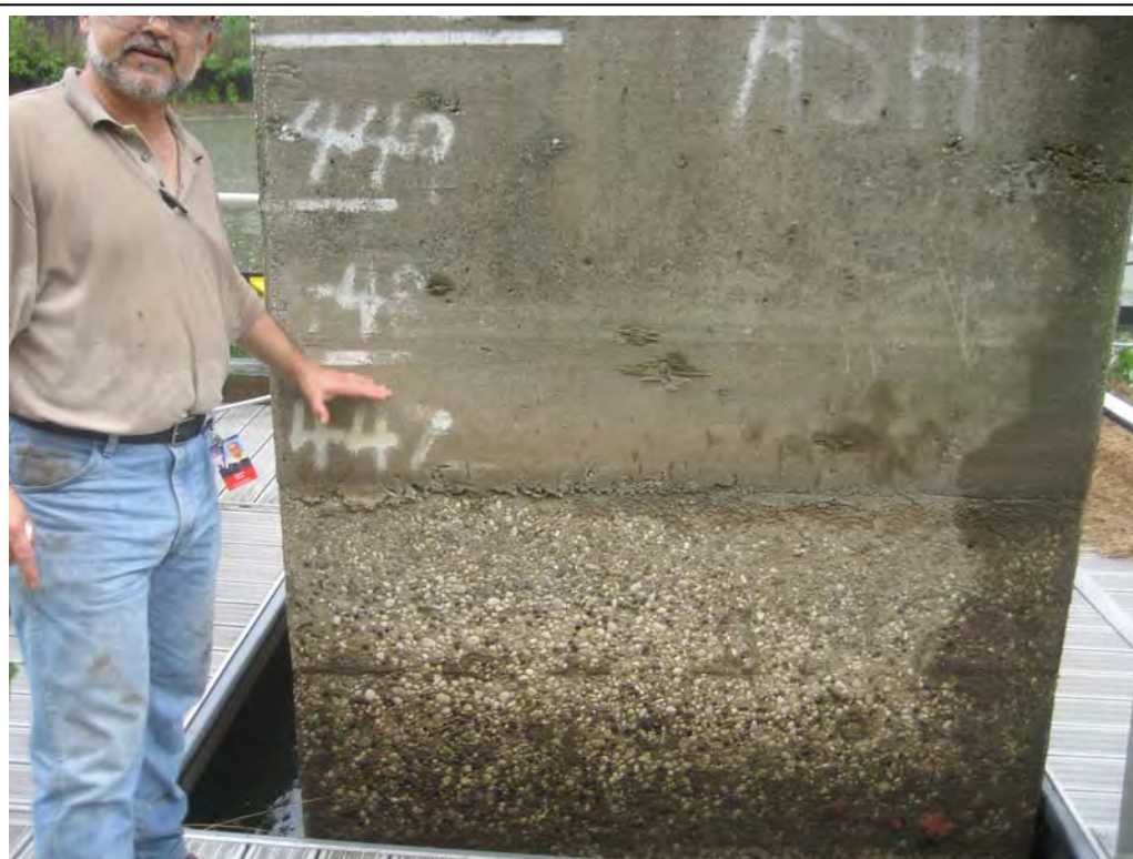
#10 - Surface Wear of Concrete Spillway Riser. EL 447 was Former Normal Pool Level.
