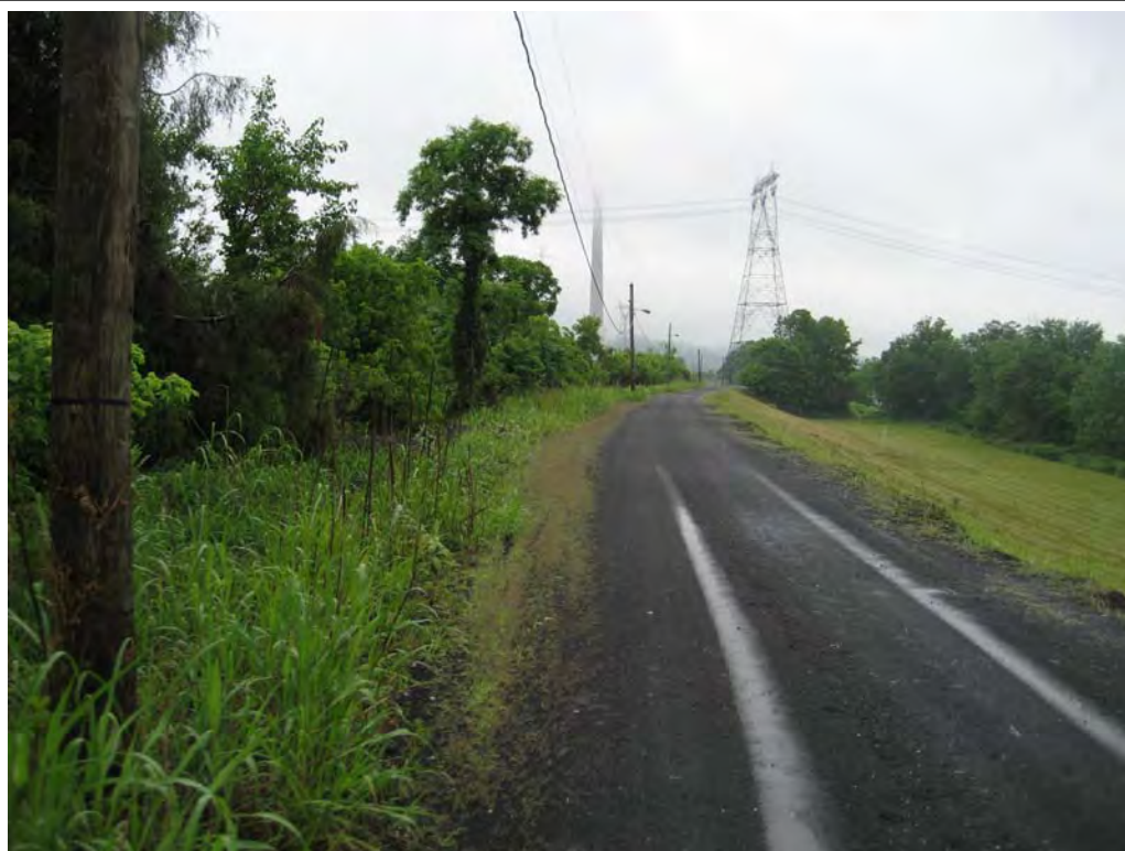
#11 - Access Road on Crest with Shallow Ponding in Tire Ruts looking eastward toward left abutment
