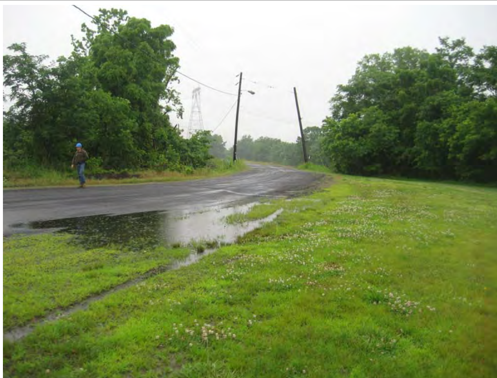
#5 - Standing Water on Crest Near Right Abutment
