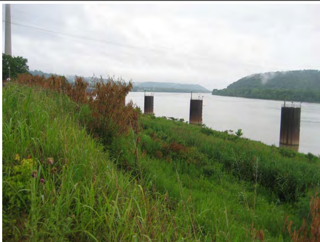
#14 - Lower Slope of Downstream Face at Location of Wet Areas
