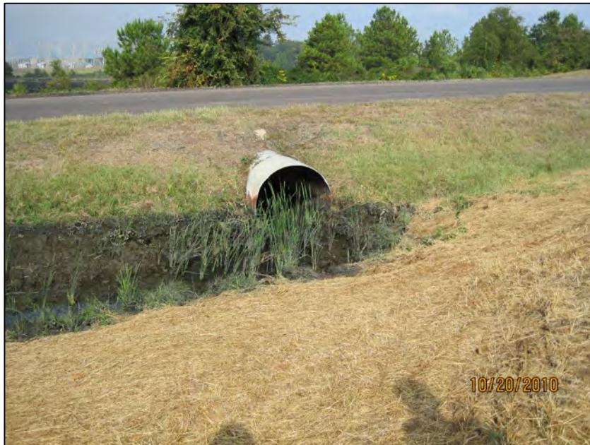
12 SECONDARY ASH POND-LOOKING WEST AT LPDES OUTFALL 002 CHANNEL AND PIPE CULVERT UNDER ROADWAY
