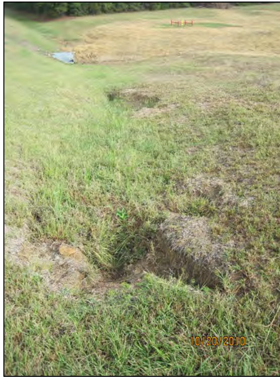
37 ASH POND 2-EROSION ON DRAINAGE SWALE OUTSIDE AND AWAY FROM DOWNSTREAM EMBANKMENT TOE
