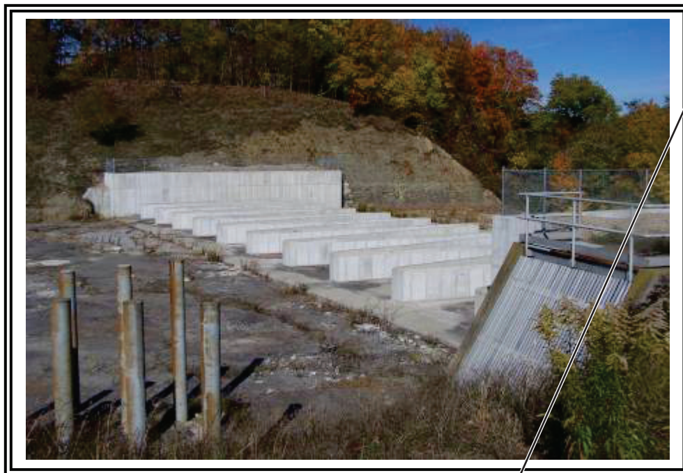
Service spillway and emergency spillway.
