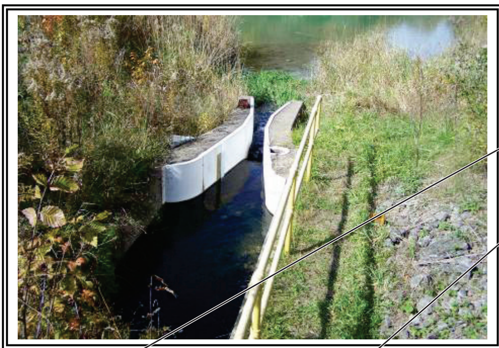
Parshall flume monitoring point for blanket drain seepage.
