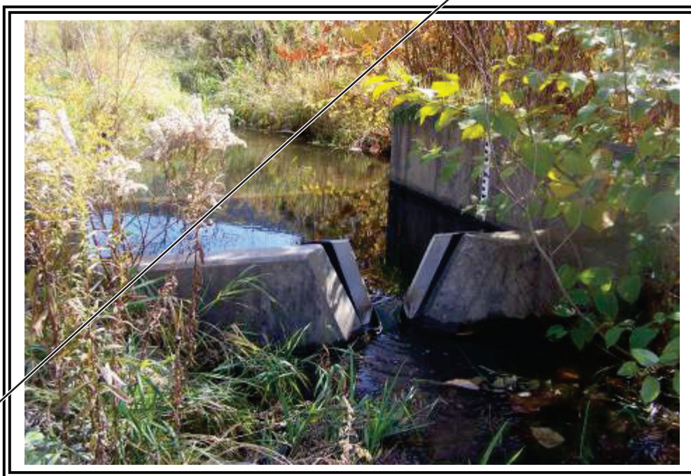
V-notch monitoring weir for west abutment seepage monitoring. Clogged culvert was causing back flow during our site visit.
