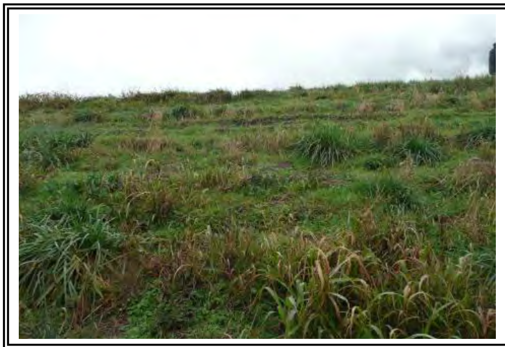
Mowing ruts on west dike outboard slope.
