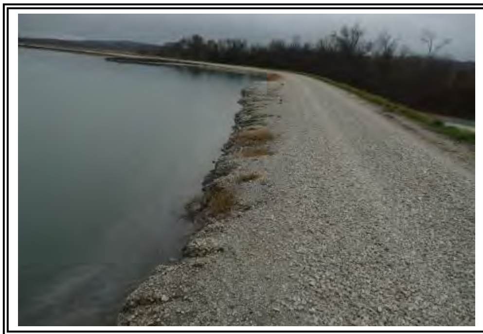
North dike inboard slope. Note beaching erosion and erosion rills.
