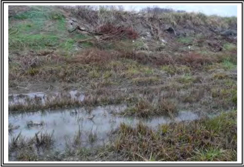
Poor drainage at toe of north dike where culvert under road has been blocked.
