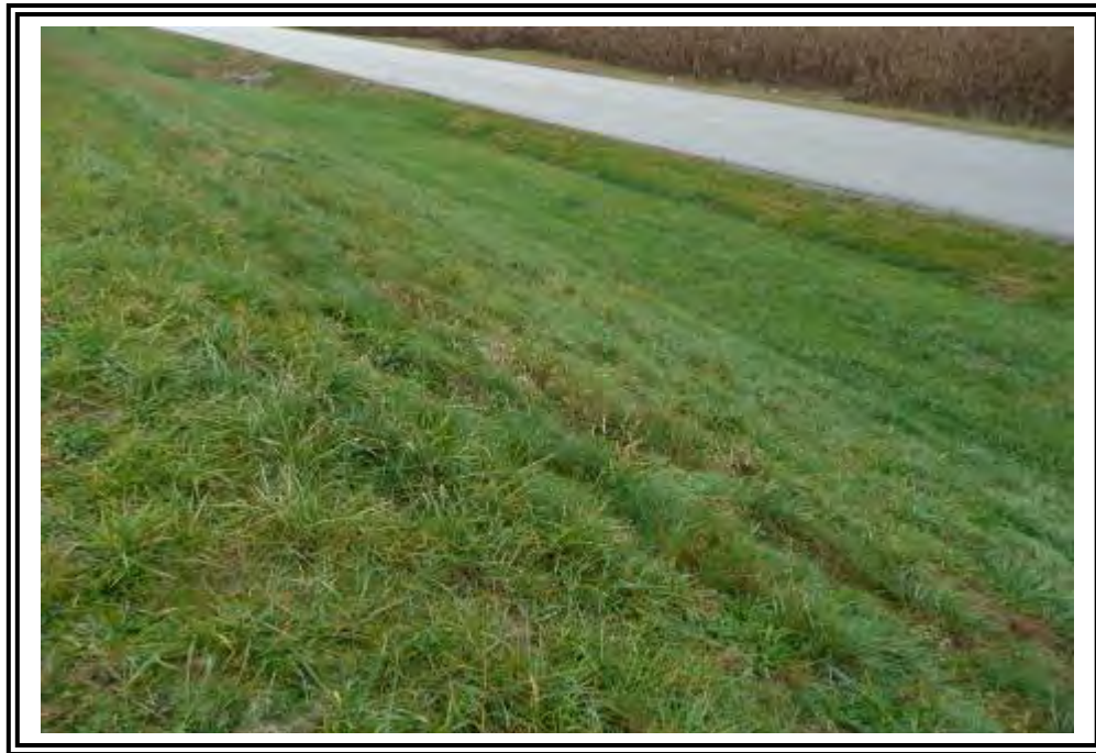
Mowing ruts in surface on west dike outboard slope.
