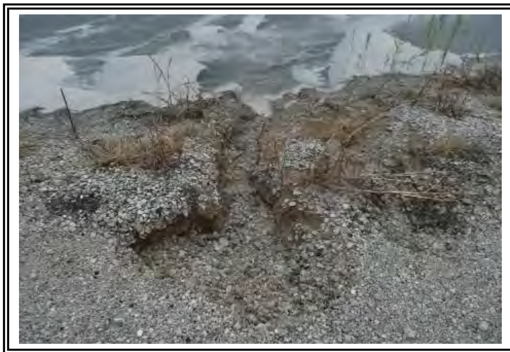
Erosion rills on inboard slope of south dike.
