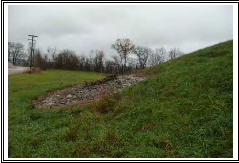
Rock toe drain at northeast corner of Ash Pond A, outboard slope.
