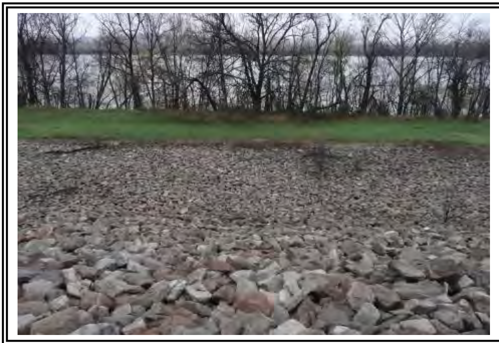
East dike emergency spillway, looking east toward the Ohio River. Note isolated dying woody vegetation.
