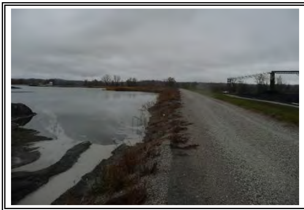
South dike, inboard slope looking east at open pond beyond ash processing area.
