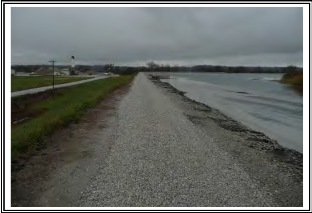
North dike crest looking east. Note wet area at toe of dike to left of photo.
