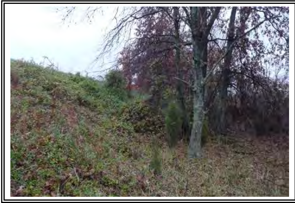
South dike outboard slope, looking east. Note trees and brush vegetation on slope and at slope toe.
