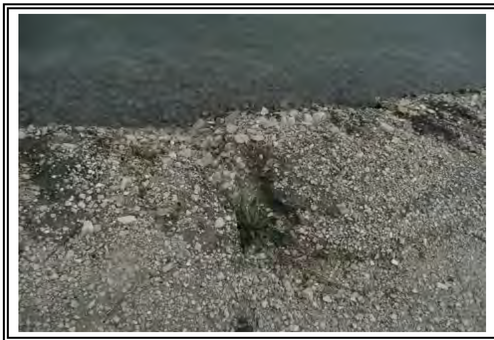
Close up of slight beaching on inboard slope of north dike.
