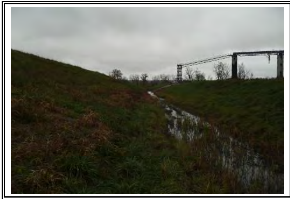
Standing water in drainage swale at toe of south dike.
