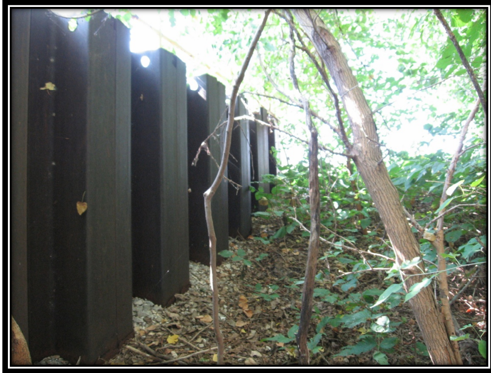
Photo 13 – South Side of the Oil Delivery Sheet Pile Platform (Note Penetration into Embankment)
