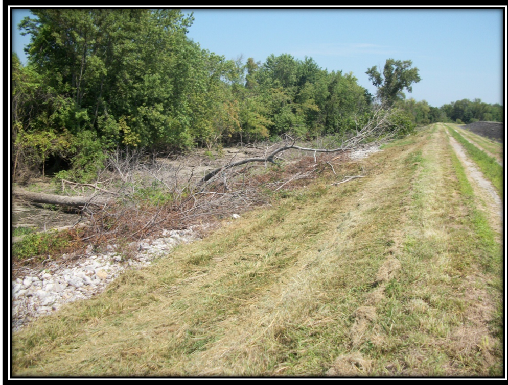
Photo 31 – Fly Ash Pond Embankment (Note Riprap and Felled Tree Debris near Toe)
