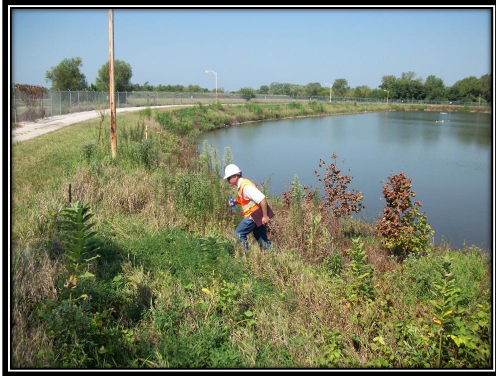
Photo 23 – Upstream Slope of the Bottom Ash Pond (Note Steep Slopes and Light Pole Penetrations)
