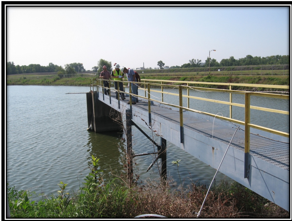
Photo 14 – Outlet Works for the Bottom Ash Pond (Note Broken Support of Walkway)
