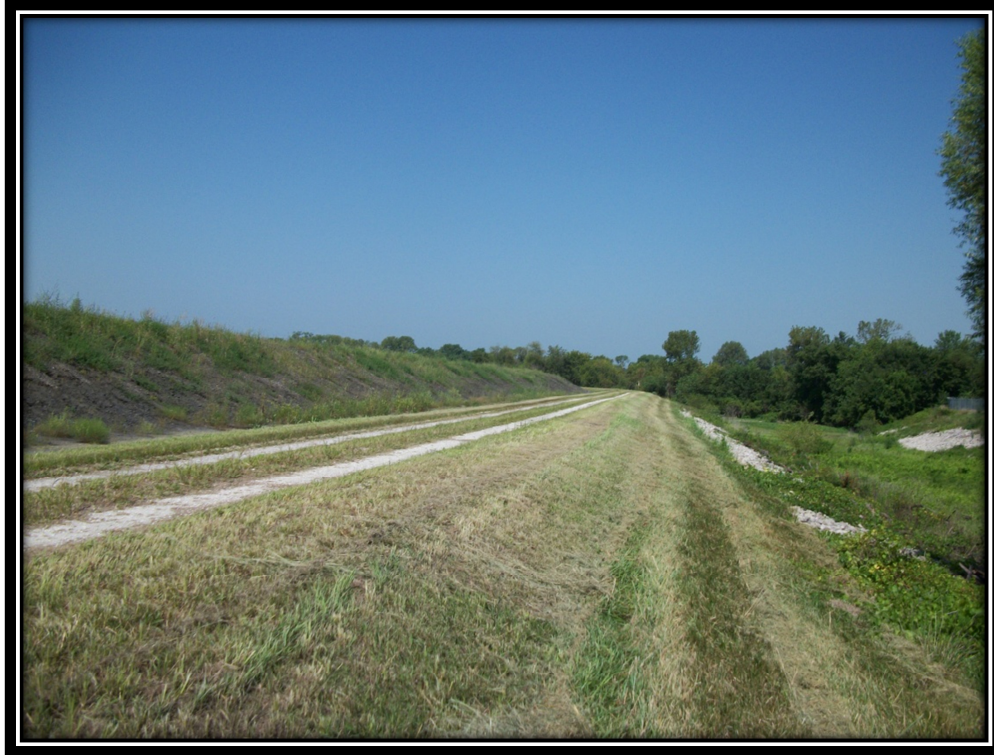
Photo 29 – Typical Embankment of Fly Ash Pond (Note Fly Ash Cell Divider Embankment to Left in Photo)
