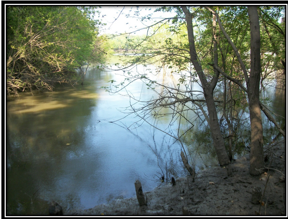
Photo 16 – Bottom Ash Pond Outlet Pipe Discharge Bay (Note Illinois River in Background)
