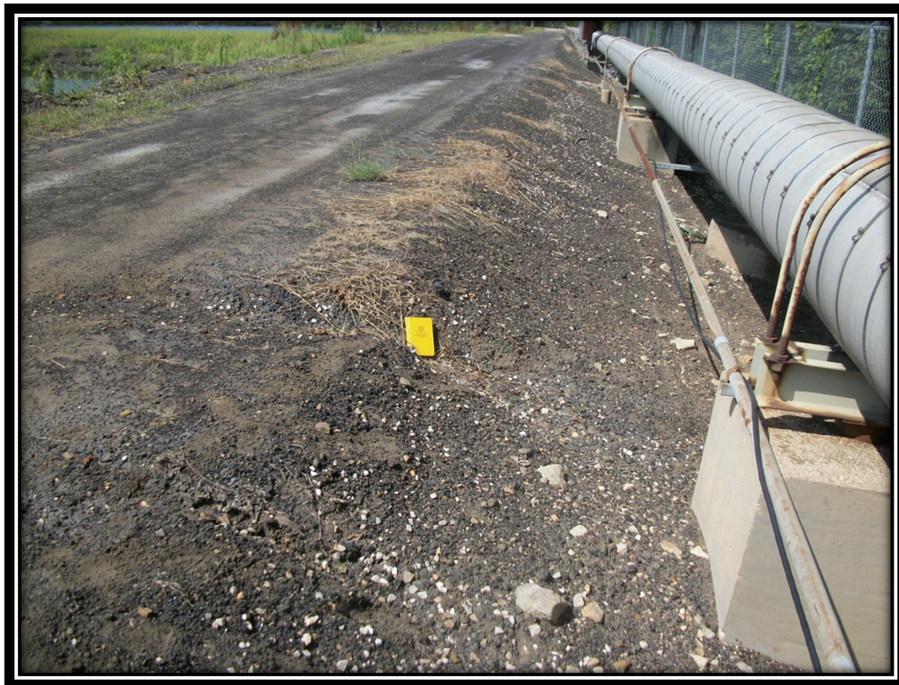
Photo 2 – Minor Surface Erosion of Bottom Ash Pond Crest (Note Typical Crest Condition and Pipeline)
