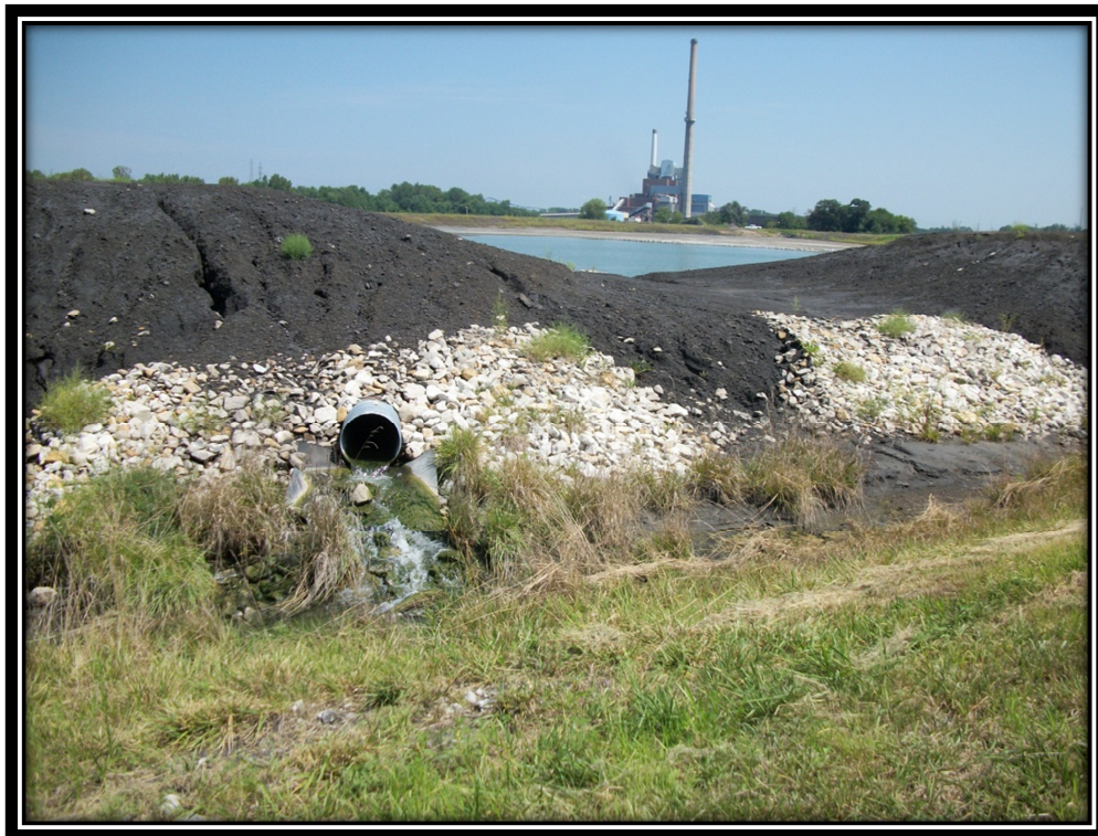
Photo 36 – Fly Ash Pond Culvert Pipe between cells 1 and 4 (Note Emergency Spillway Cut)
