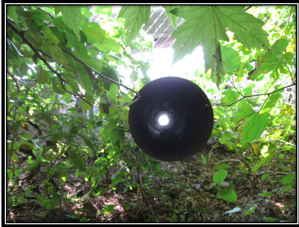
Photo 11 – Emergency Spillway Pipe for the Bottom Ash Pond without any Noticeable Obstructions
