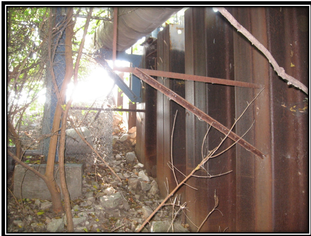
Photo 12 – North Side of the Oil Delivery Sheet Pile Platform (Note Penetration into Embankment)
