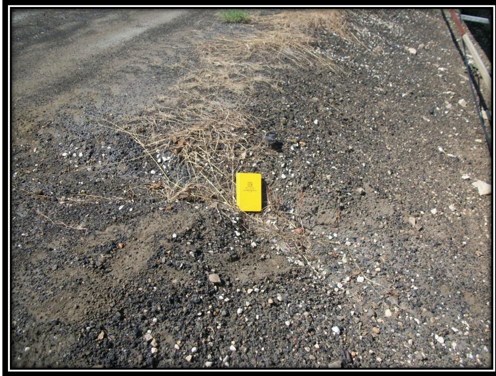
Photo 3 – Minor Surface Erosion of Crest and Downstream Slope of the Bottom Ash Pond (Typical)
