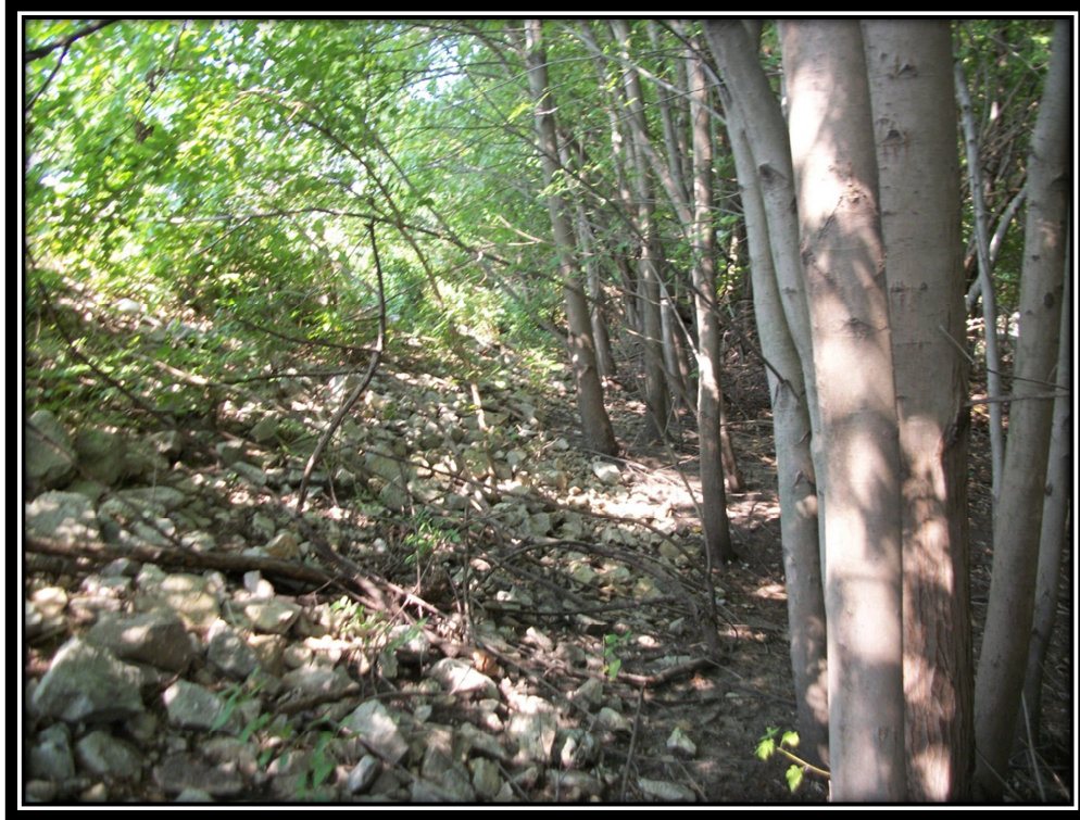
Photo 7 – Riprap and Mature Trees on the Downstream Slope of the Bottom Ash Pond (Typical)
