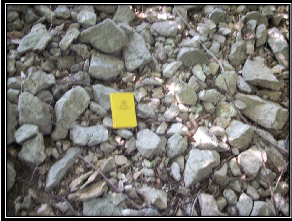
Photo 9 – Undersized Riprap on Downstream Embankment of the Bottom Ash Pond
