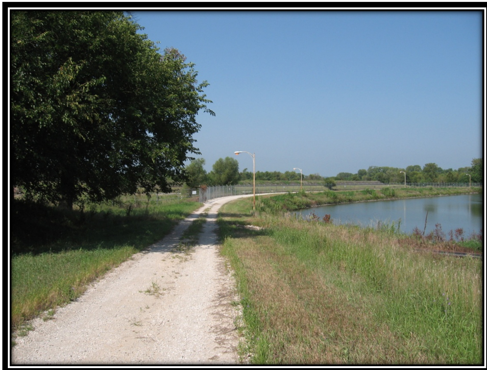
Photo 28 – Typical Crest Condition of the Bottom Ash Pond (Note Light Pole Penetrations in Crest)
