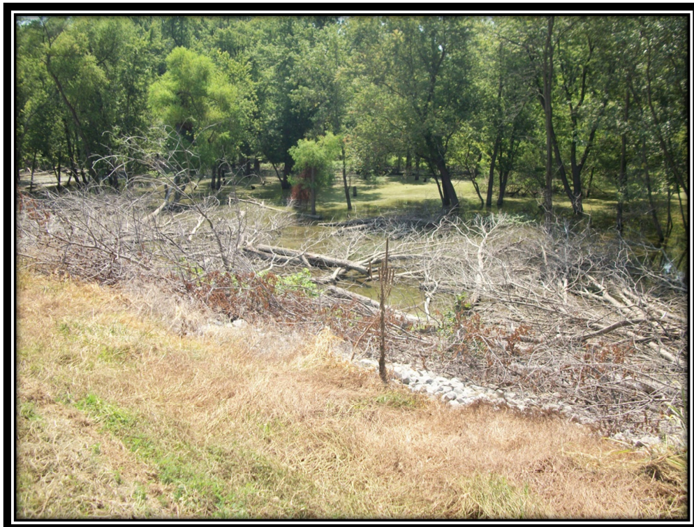
Photo 34 – Flooded Timber and Felled Tree Debris at the Toe of the Fly Ash Pond
