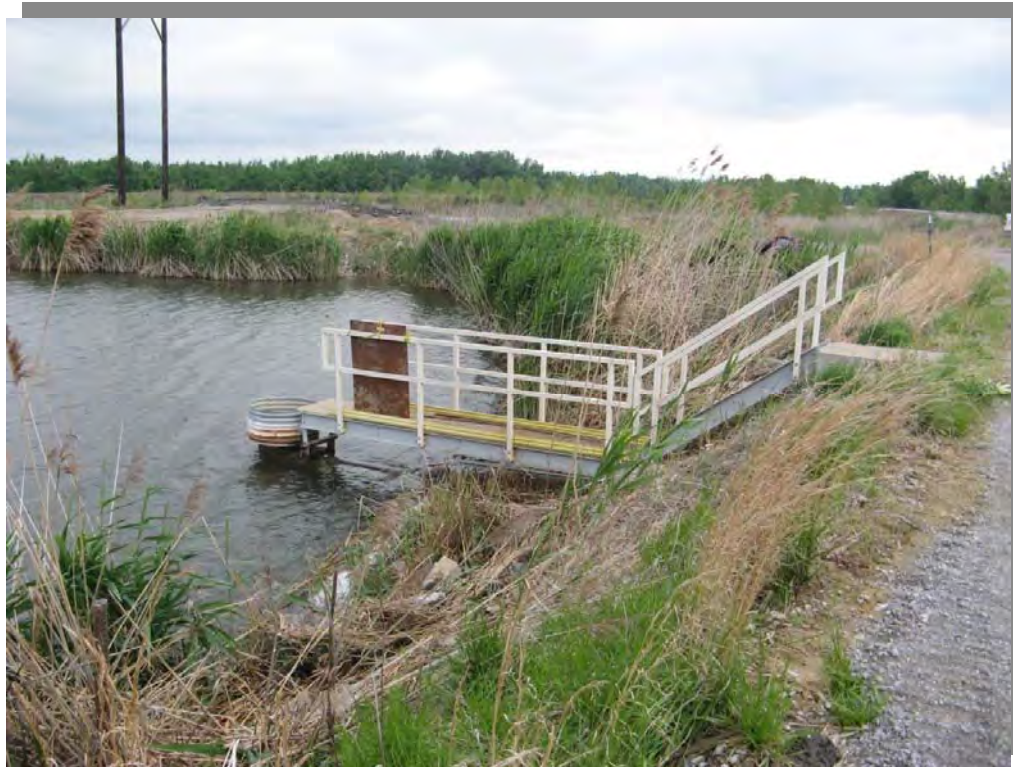
Photo 15 – Southern Pond primary outlet structure.
