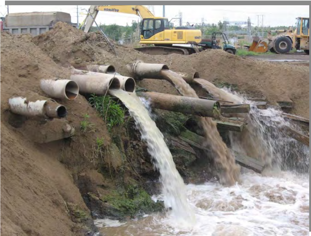
Photo 13 – CCW discharge from Joppa Plant into Ash Pond at southwestern corner of Southern Pond..
