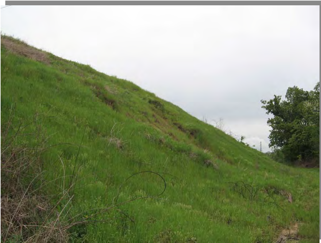
Photo 22 – Slides and sloughs on east embankment of Southern Pond, approximately 200 feet south of power lines.
