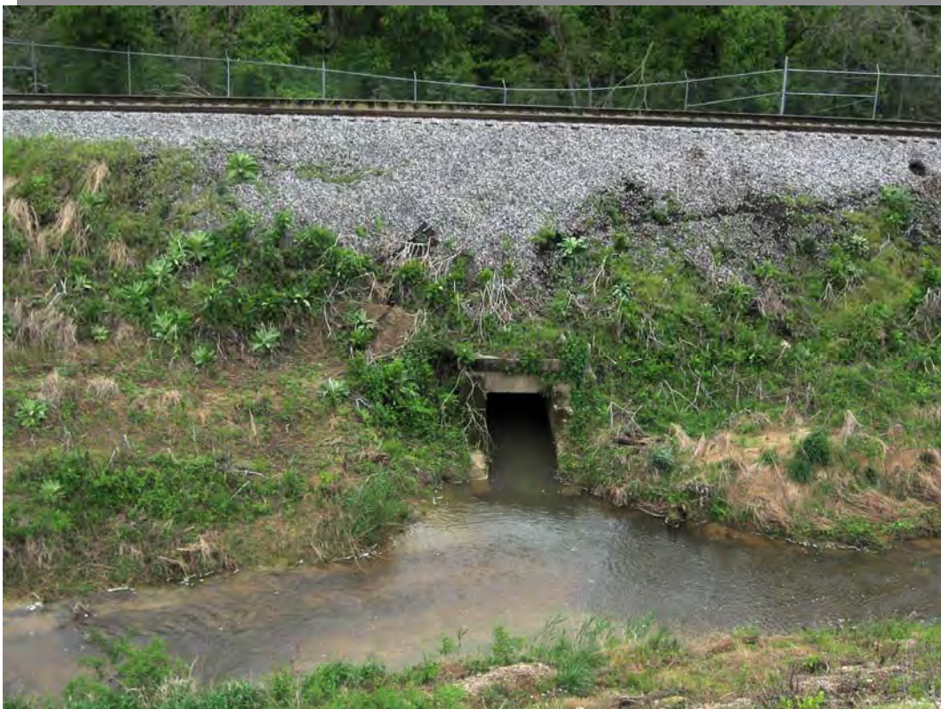
Photo 10 – Runoff from drainage area east of Ash Pond merging with Pond effluent..
