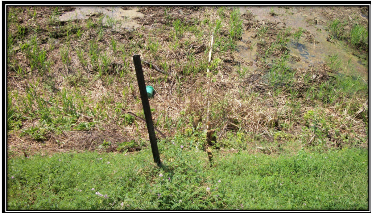
Photo 9 – Abandoned pump crossing
