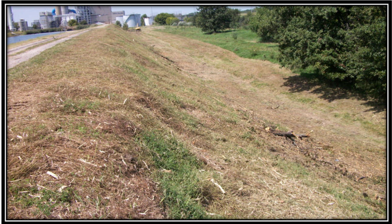
Photo 19 – Slope failure along downstream slope
