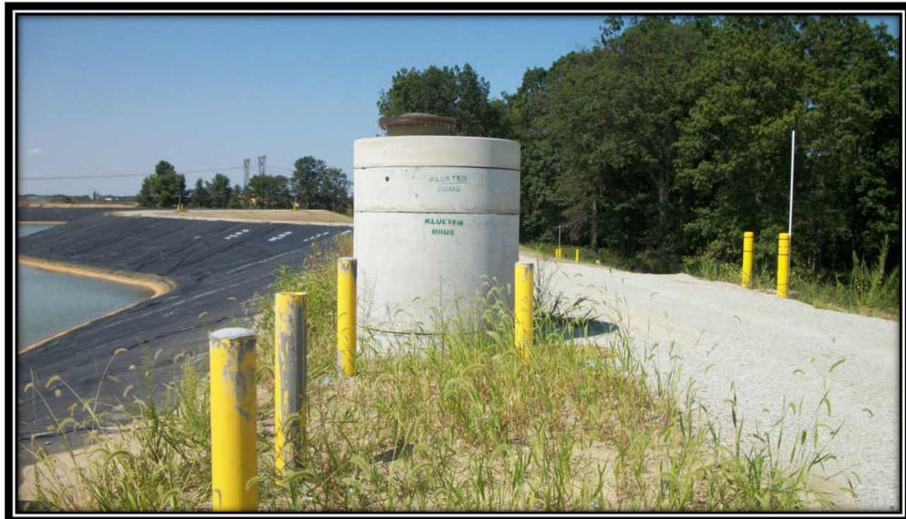
Photo 47 – Inlet of recirculation system
