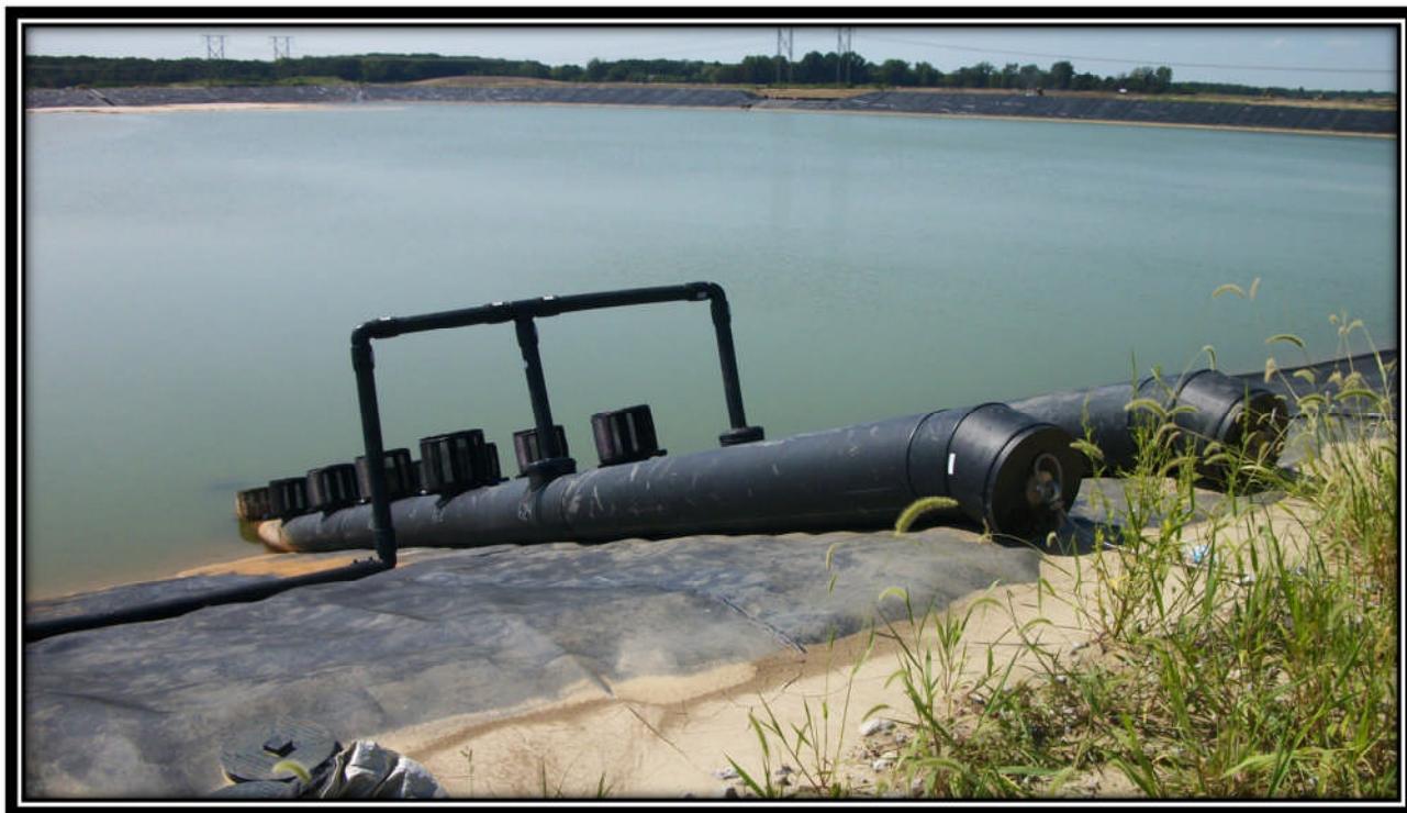
Photo 46 – Inlet of recirculation system
