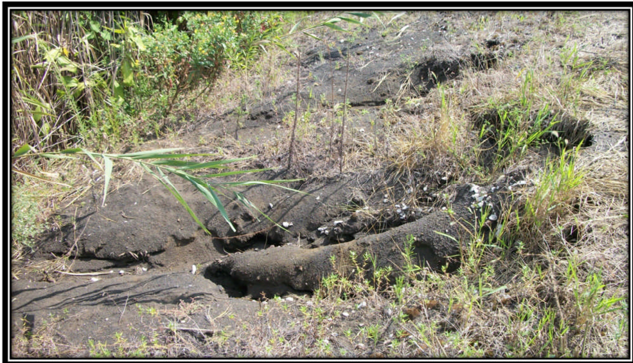
Photo 3 – Gulleys on upstream slope of South embankment
