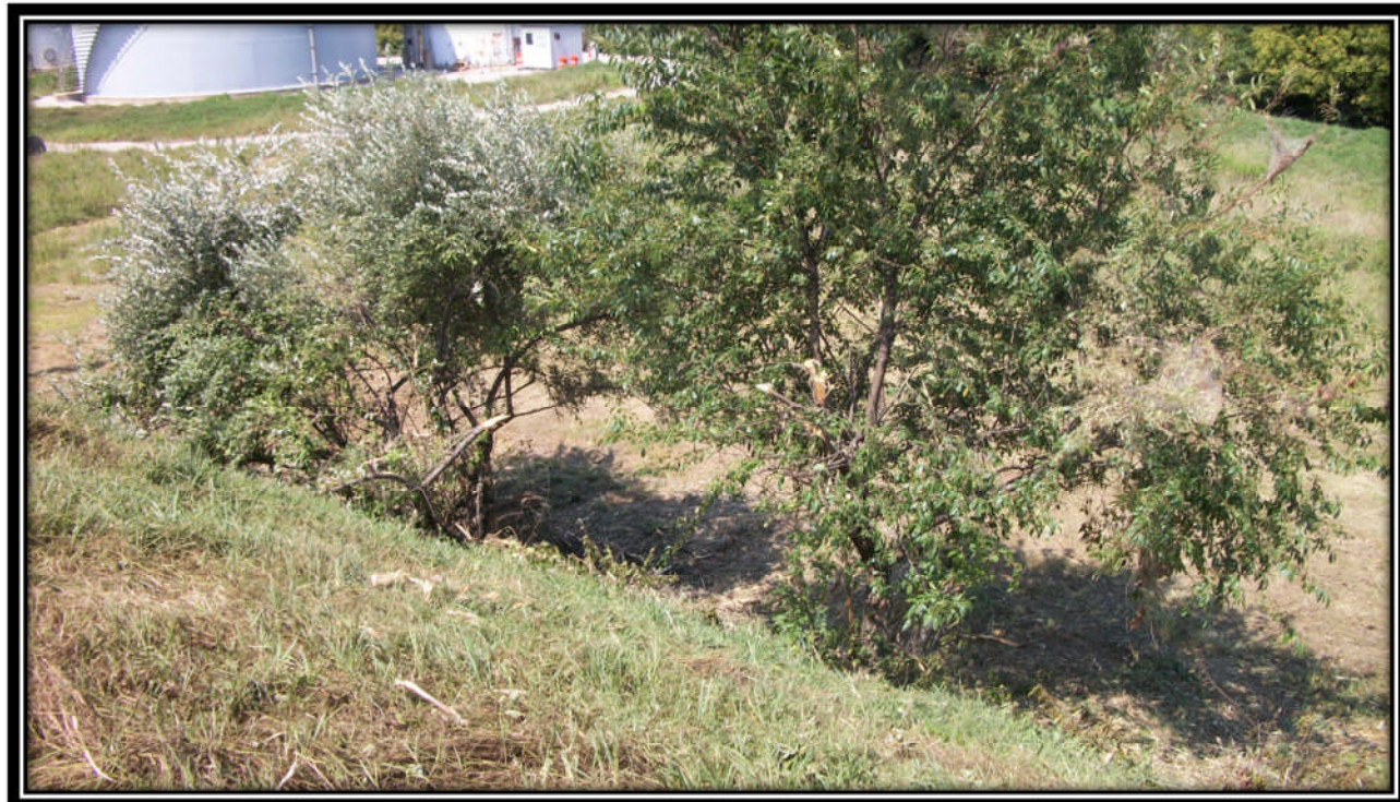
Photo 23 – Trees on downstream slope
