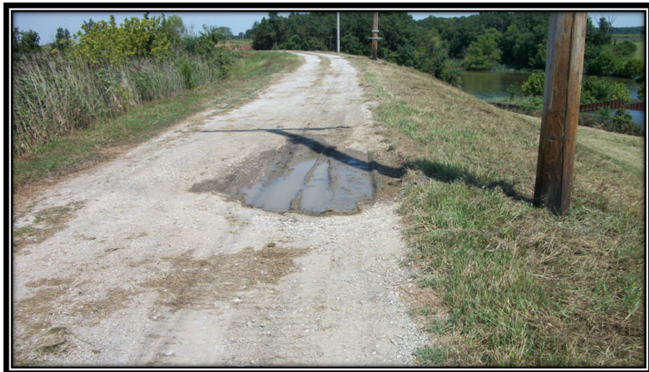
Photo 14 – Rutting on crest
