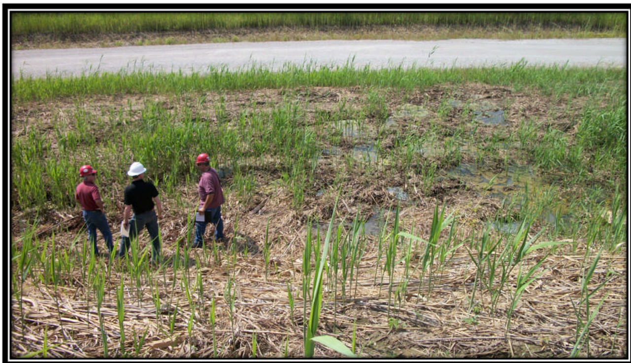
Photo 4 – Ponding at downstream toe of South embankment
