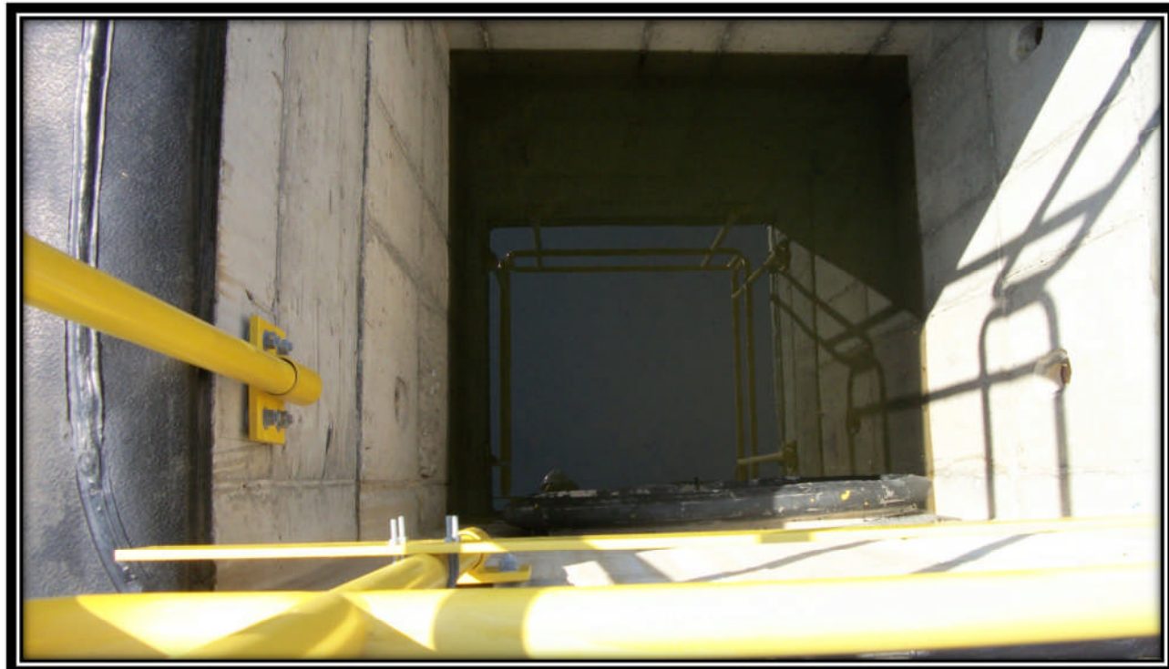
Photo 43 – Outlet box inside
