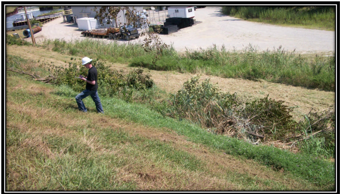
Photo 12 – Debris at downstream toe of East embankment
