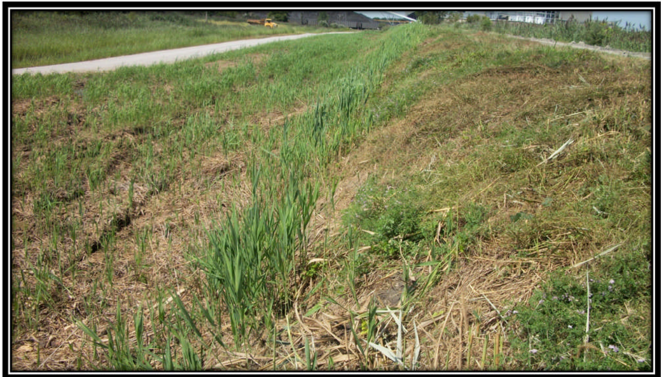
Photo 8 – Shallow sloughing on downstream slope of south embankment
