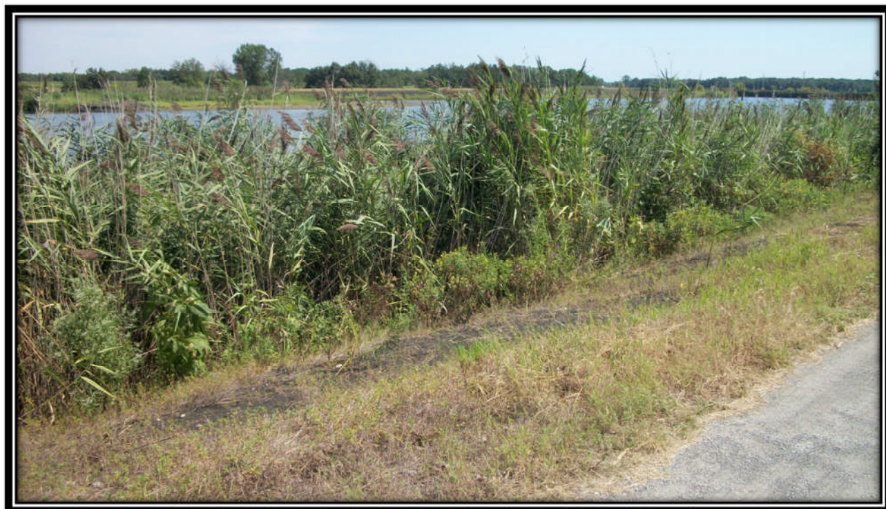
Photo 2 – Vegetation on upstream slope of South embankment
