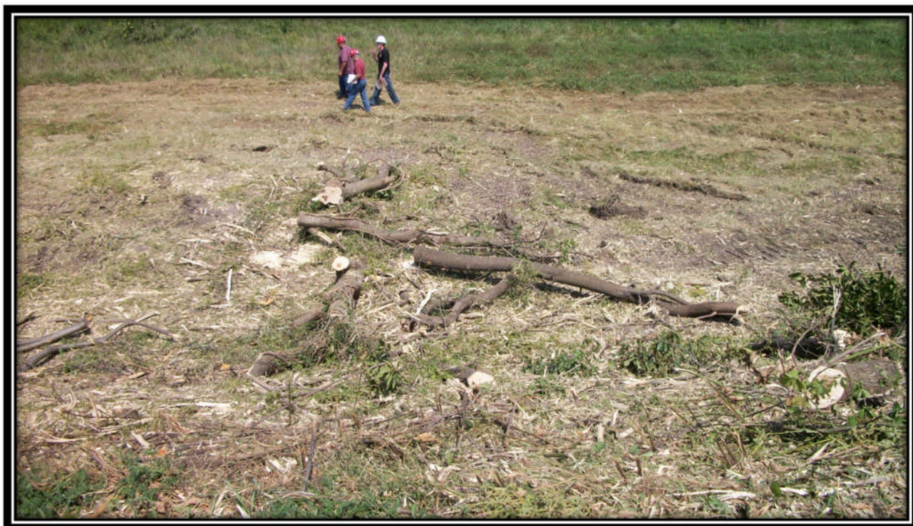
Photo 22 – Debris on downstream slope of North embankment
