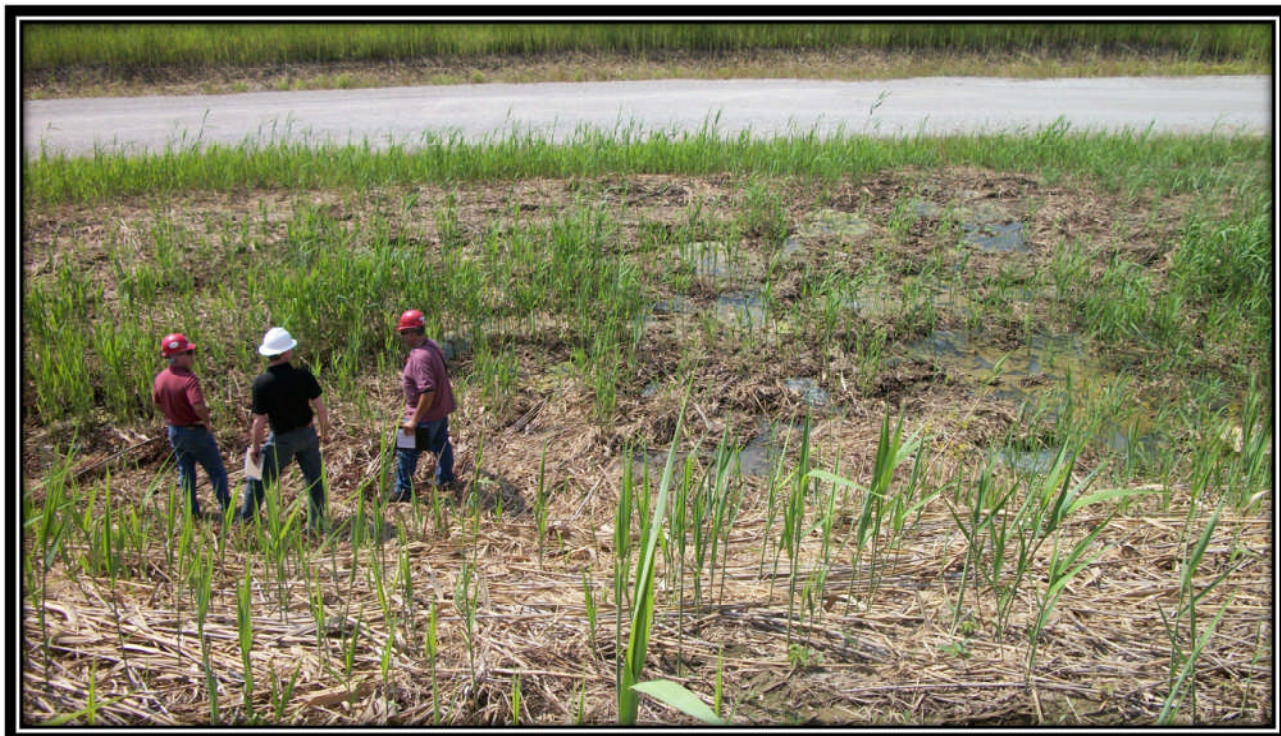
Photo 4 – Ponding at downstream toe of South embankment
