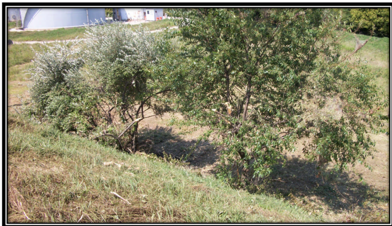
Photo 23 – Trees on downstream slope
