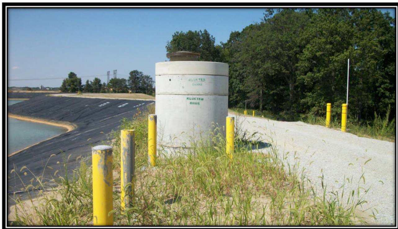
Photo 47 – Inlet of recirculation system
