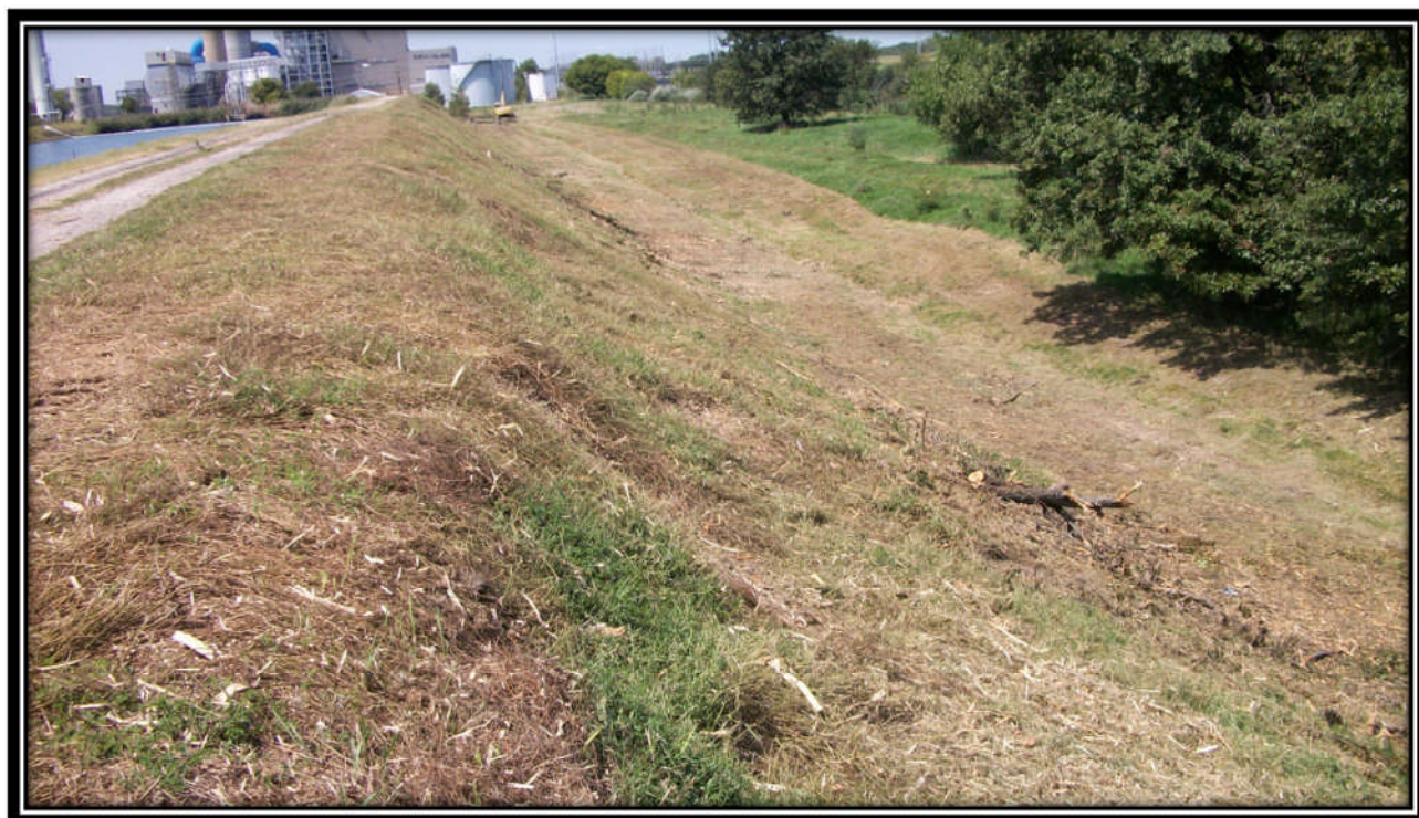
Photo 19 – Slope failure along downstream slope
