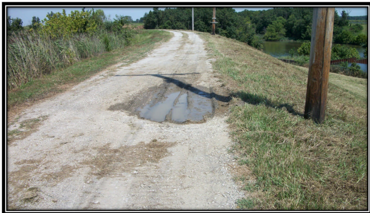
Photo 14 – Rutting on crest
