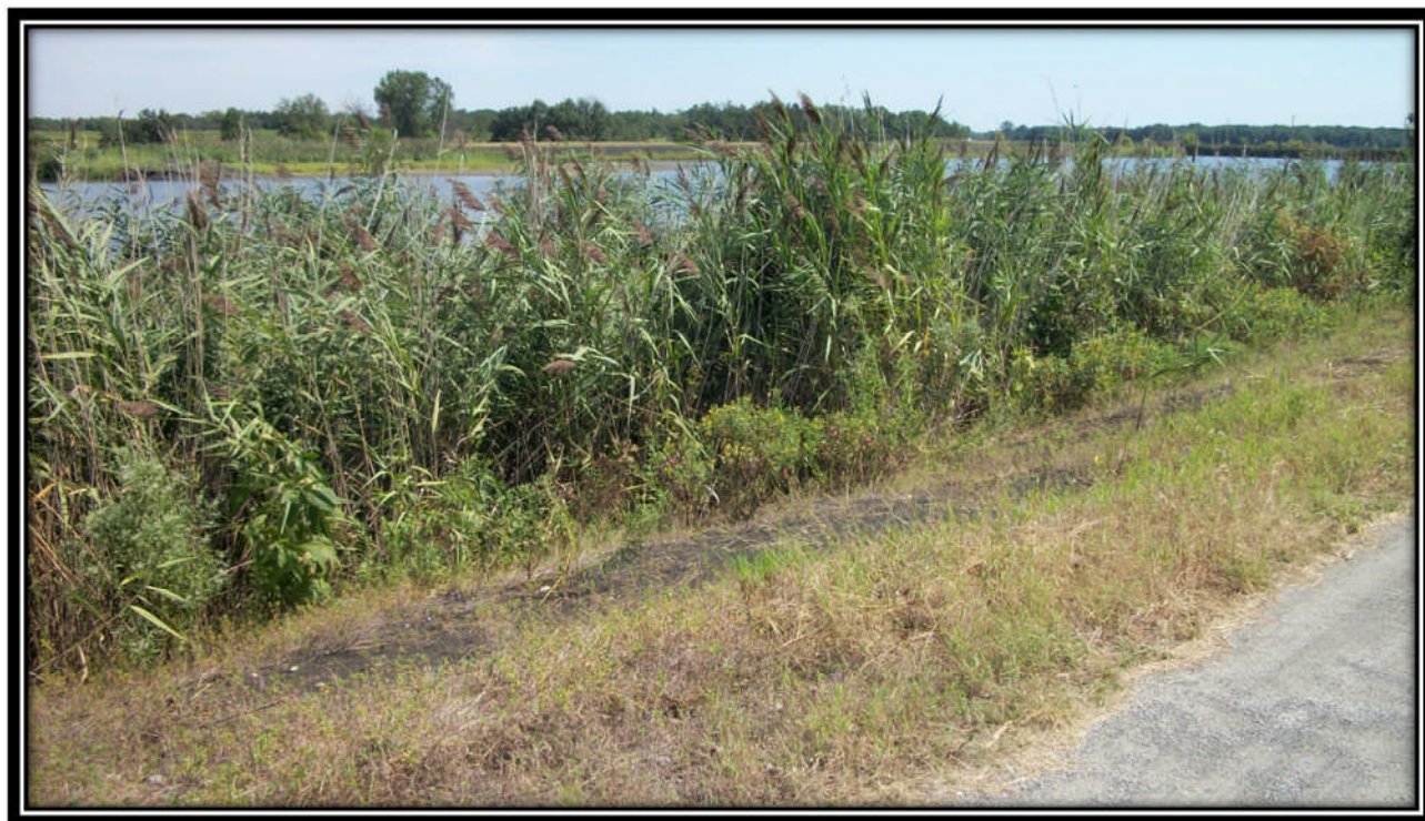
Photo 2 – Vegetation on upstream slope of South embankment
