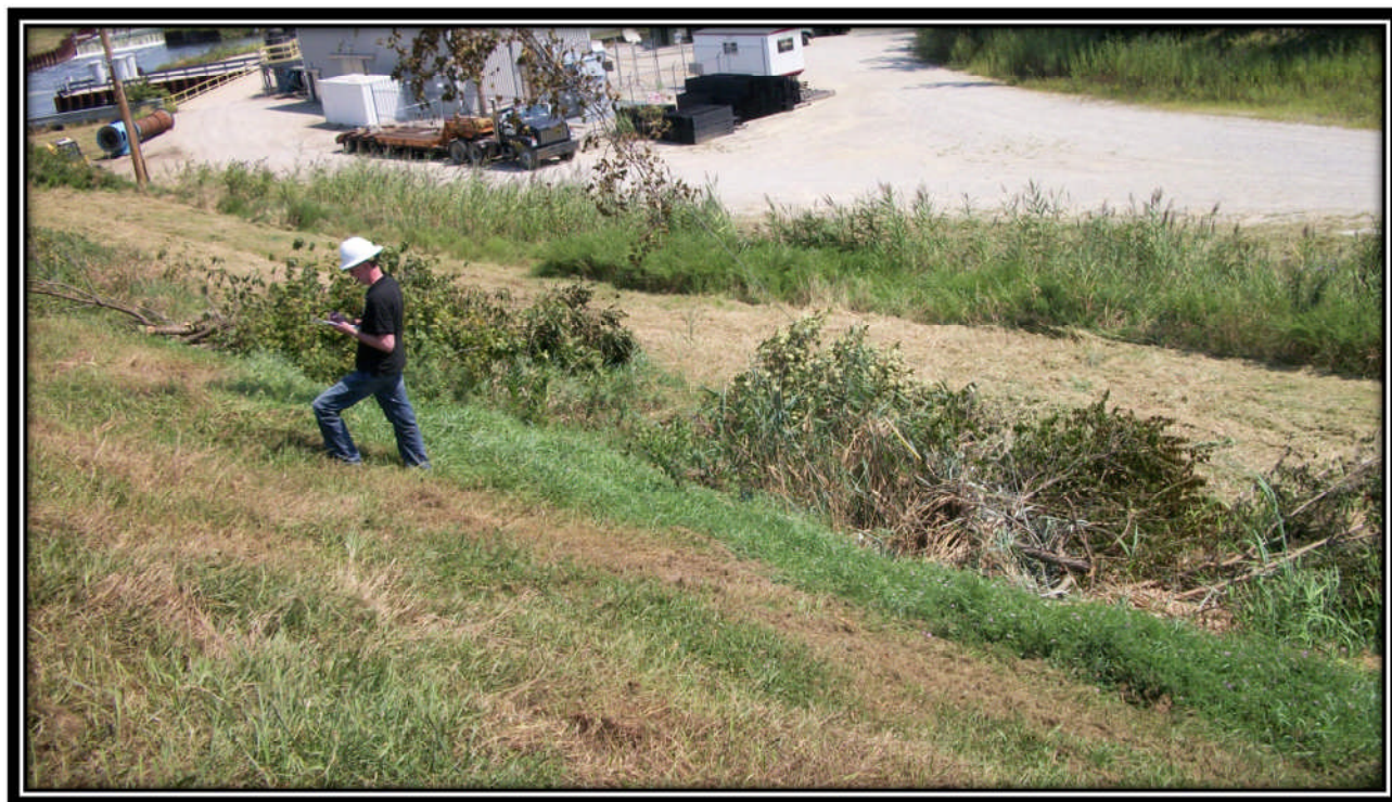
Photo 12 – Debris at downstream toe of East embankment
