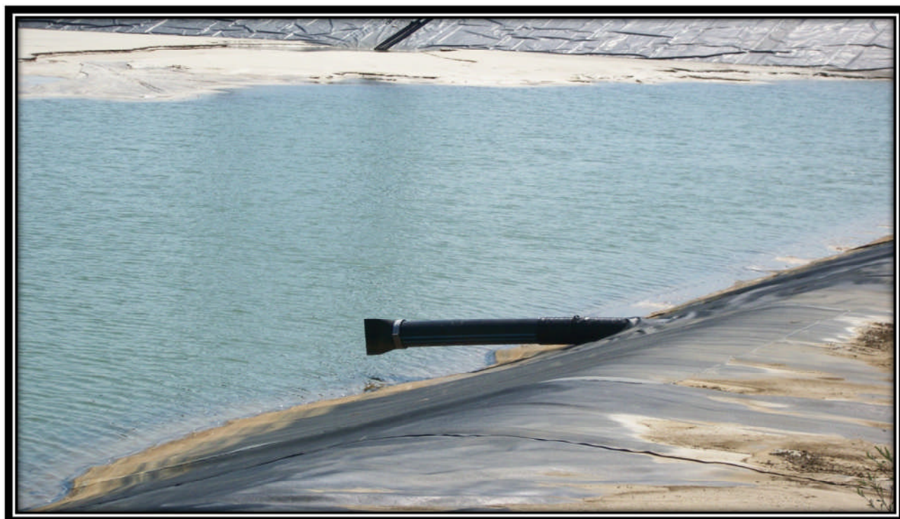
Photo 41 – Pipe between larger and smaller pond
