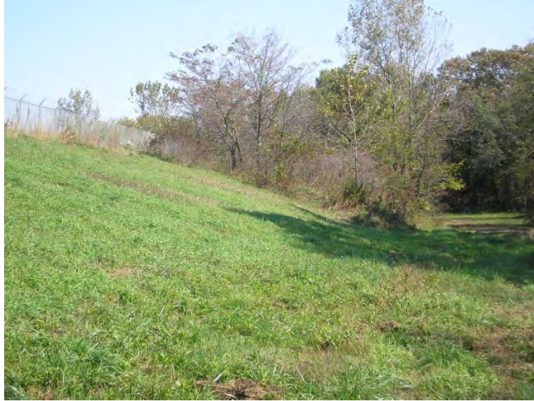
Figure 5.2.3-1: Main Ash Pond South Dike Down-Gradient Slope at Western End of Embankment.
