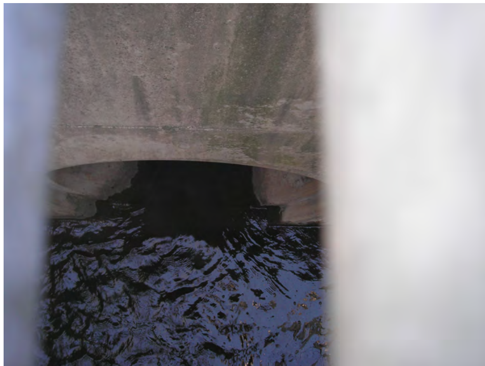
Photograph 5: Decant Water flow into Main Ash Pond Primary Spillway Structure Discharge Conduit (One of Two Parallel 66-inch Concrete Pipes)
