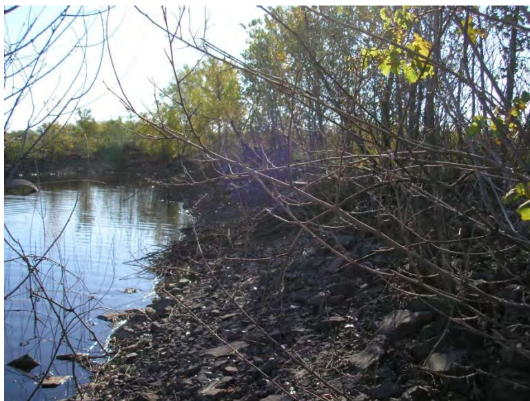
Figure 5.4.4-2: Abutment formed by junction of Main Ash Pond North Dike (Foreground) and Zero Liquid Discharge Pond East Dike
