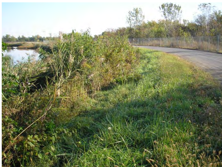
Figure 5.2.2-1: Main Ash Pond South Dike Up-Gradient Slope at Center Section of Dike
