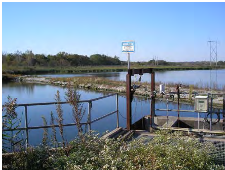
Figure 4.2.1-1: Main Ash Pond Primary Spillway Structure and Low Dike for Stilling Basin
