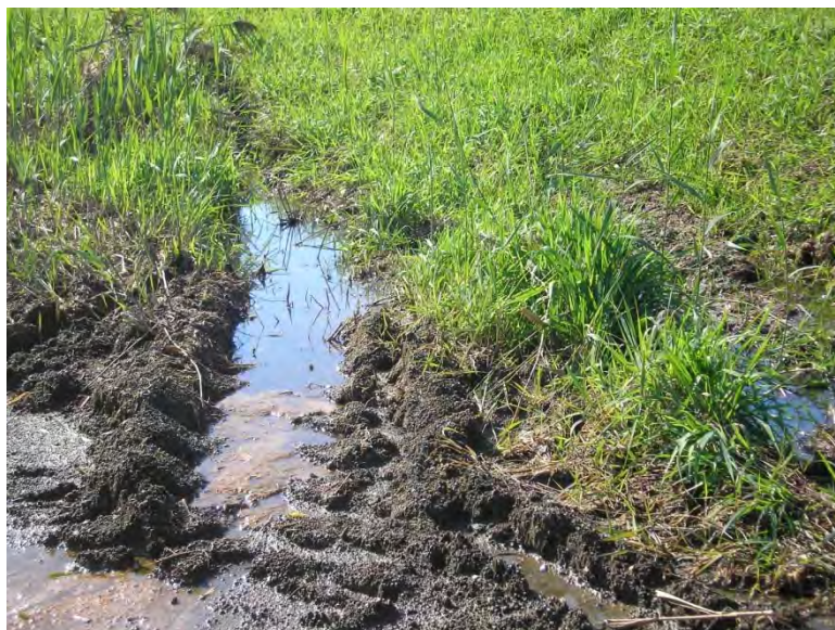
Figure 5.4.3-4: Zero Liquid Discharge Pond East Dike: Soft Wet Area Northern Section of Embankment Toe
