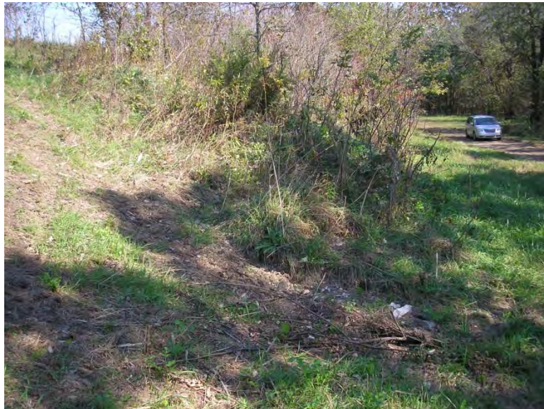
Figure 5.2.3-2: Main Ash Pond South Dike Down-Gradient Erosion at Change from Grass Ground Cover the Woodlands
