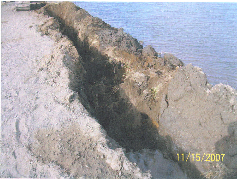
Photograph close-up of bentonite slurry running and filling the trench prior to placement of the soil/bentonite mixture.
