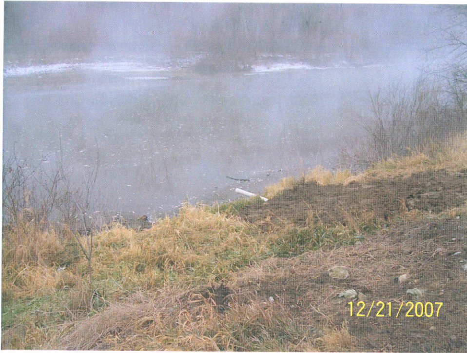
Photograph of drain tile outfall pipe. Old drain tile was determined to be the source of the seep. It was properly plumbed out to daylight so it can be observed in the future.
