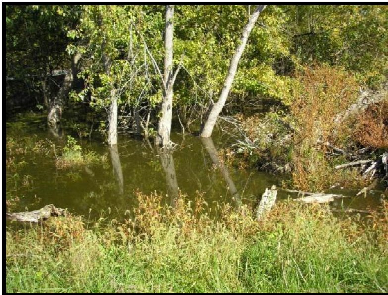
Figure 5.3.3-2: Bottom Ash Pond South Embankment: Discharge Canal Flooding back-up to Downstream Slope Toe
