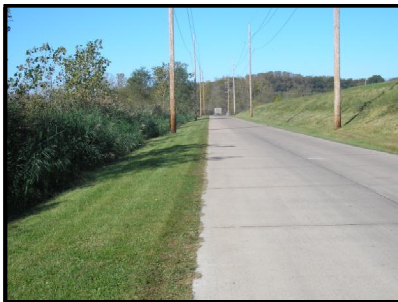
Figure 5.3.2-1: Bottom Ash Pond North Dike - Upstream Slope on Left Side of Photo
