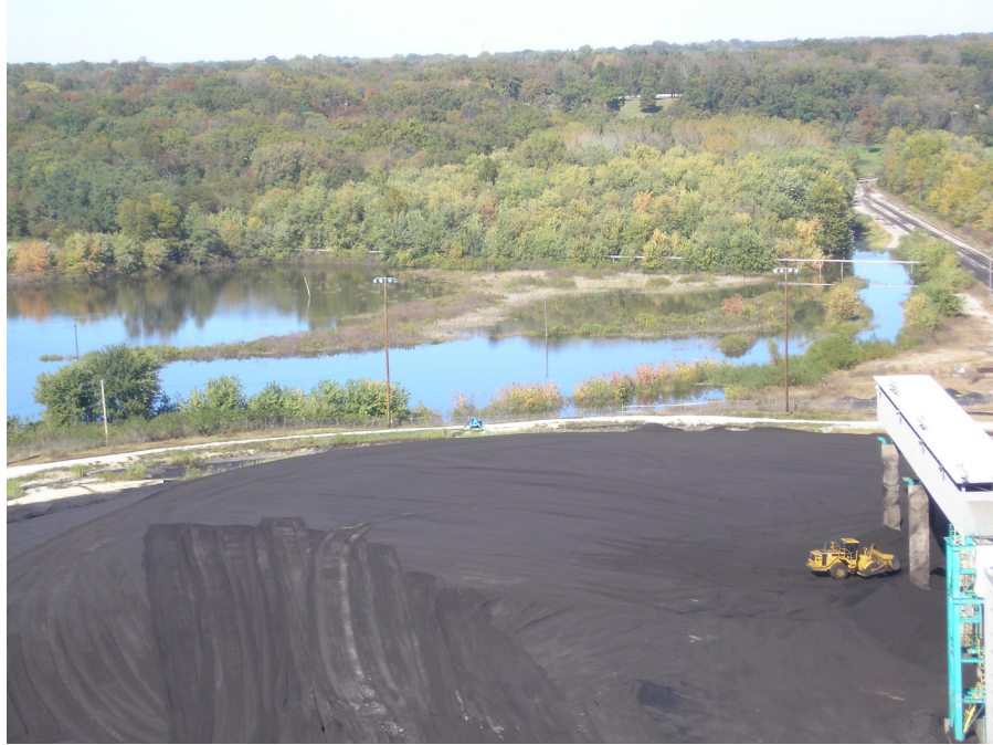
Photograph 7: Rooftop View of Ash Pond 2. Downstream Dike Located beneath Pipe Crossing in Upper Right. Dike Inundated by Flood Water from Mississippi River
