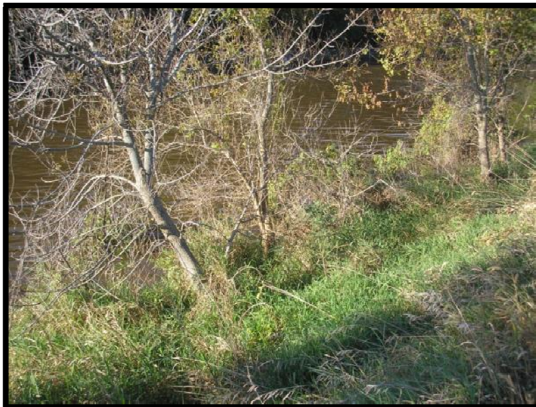
Figure 5.2.3-2: Ash Seal Pond South Dike: Canal High Water against Toe of Outside Slope
