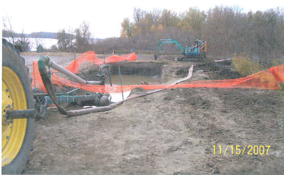
Photograph of bentonite slurry mixing pit. The Mississippi River is at background left and the ash pond is at far right.
