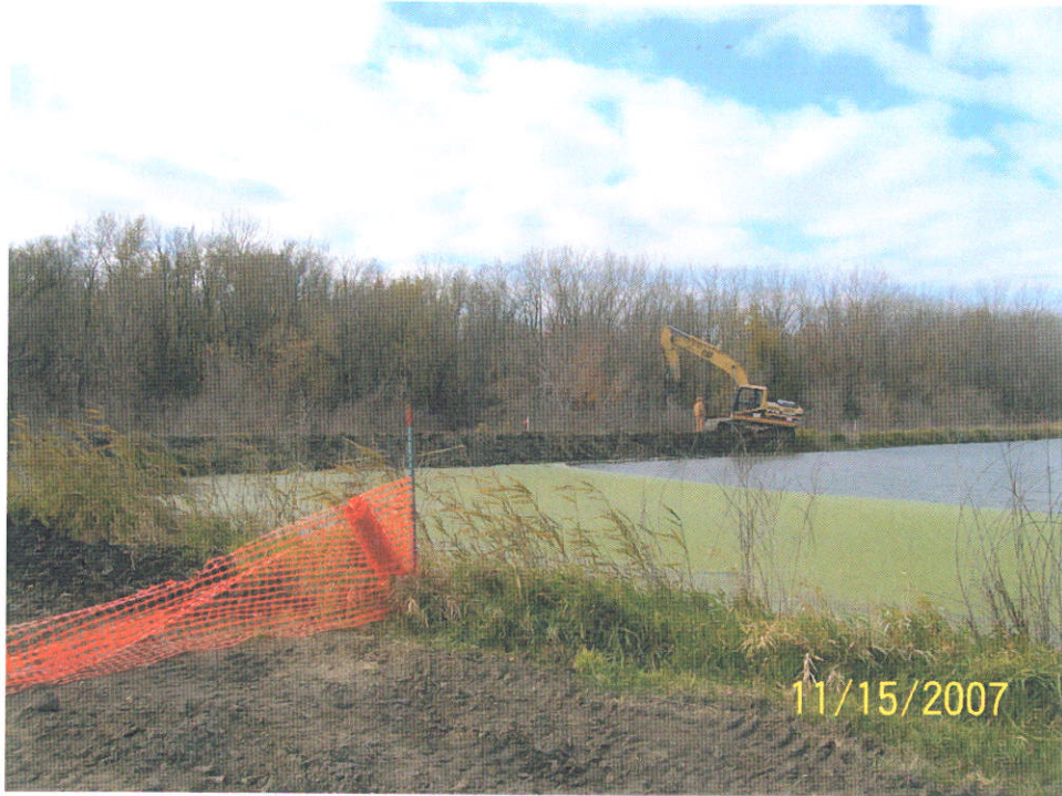
Another photo looking across the ash pond at the excavator digging the slurry trench.
