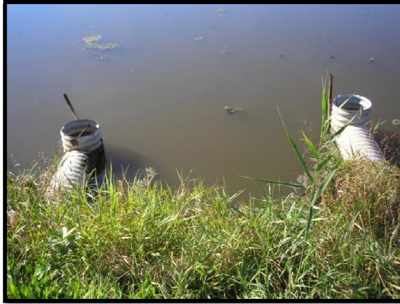
Figure 8.1-2: Bottom Ash Pond Primary Spillway Inlet
