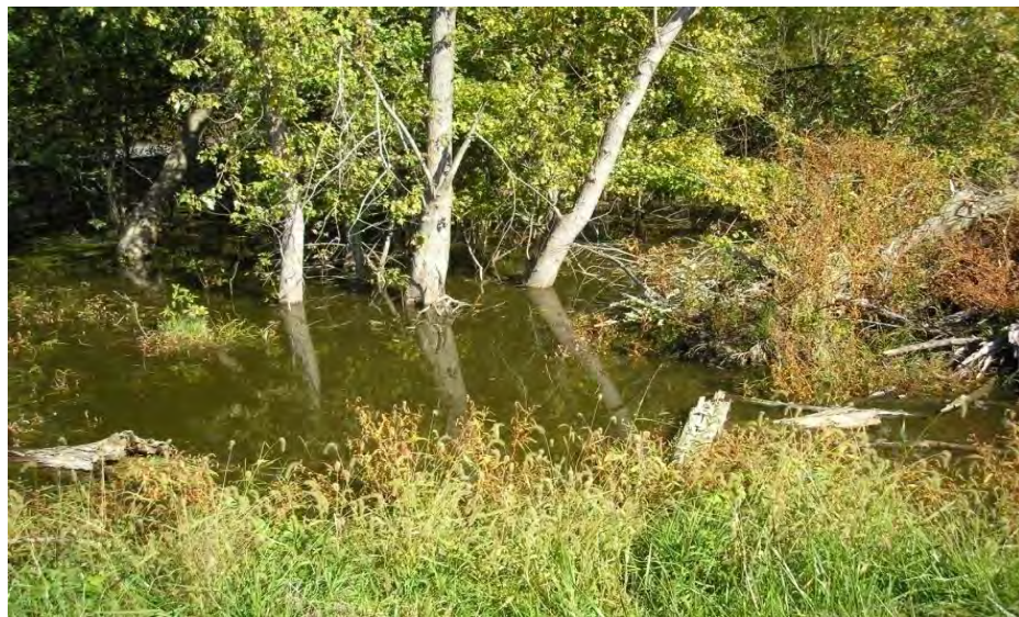
Figure 5.3.3-2: Bottom Ash Pond South Embankment: Discharge Canal Flooding back-up to Downstream Slope Toe
