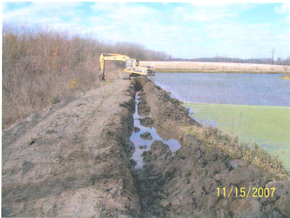
Photograph of slurry trench in berm along ash pond. Standing water is simply the bentonite slurry at the top of the trench.
