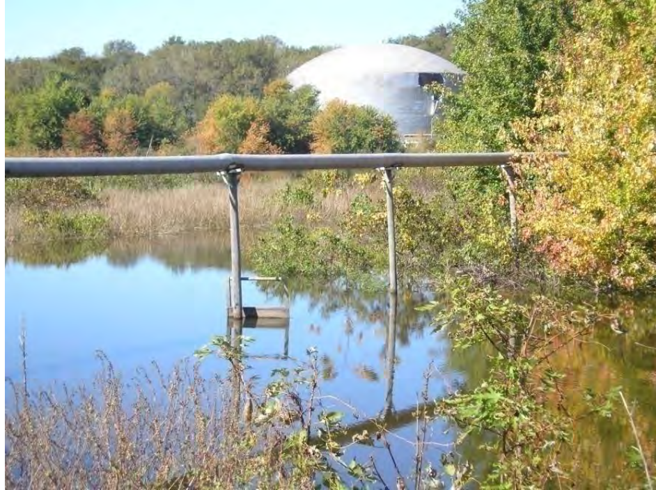
Figure 5.7.1-5: Ash Pond 2 Top of Spillway Stop Log Device
