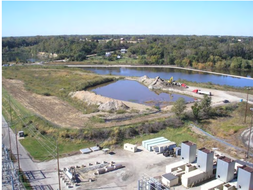
Figure 10.4.1-1” Economizer Ash Pond with Stockpile and Construction Equipment October 7, 2010 (Photo by Dewberry)
