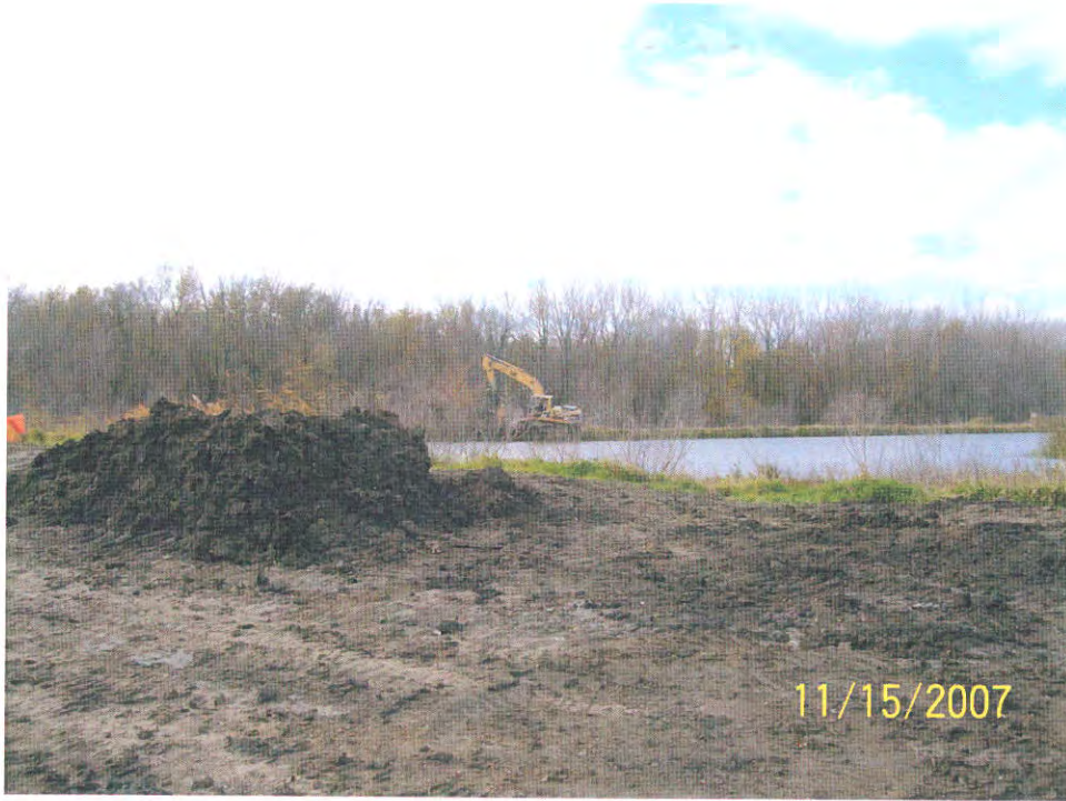
Looking across ash pond at excavator digging slurry trench in ash pond berm.
