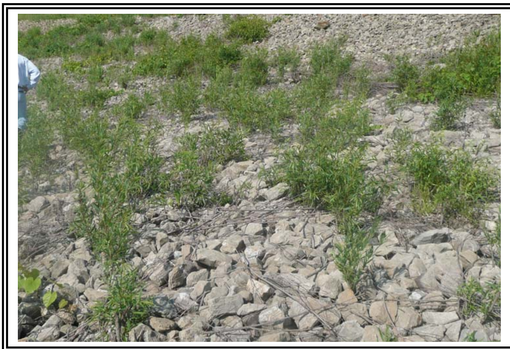
Vegetative growth within toe drain rip rap.
