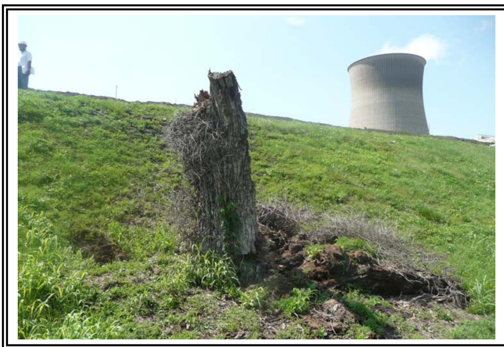
Several tree stumps noted on the downstream slope of the east dike (others except this one were cut flush to ground surface). This is in the benched out area of the east dike.
