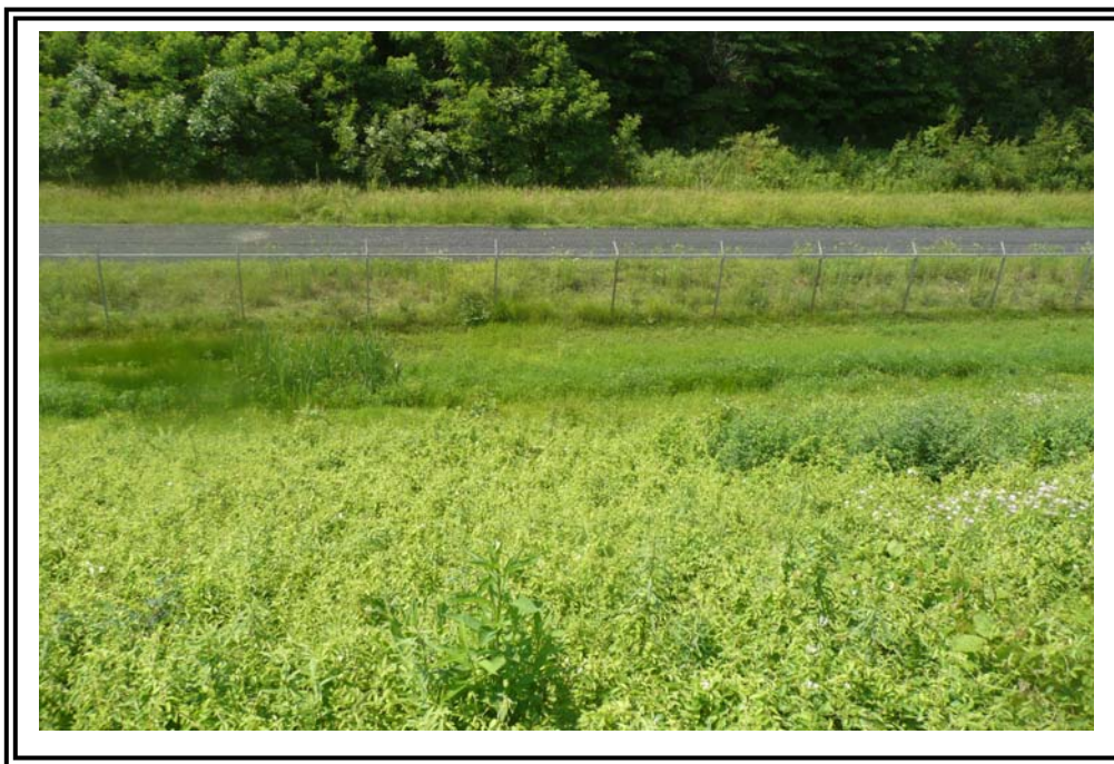
Downstream slope of the south dike about mid-slope. Note cattails growing at the toe of the slope. This area has been reportedly a wet area, but AEP believes it is related to surface drainage and in the fall 2008 reset culverts crossing the adjacent access road to pitch away from the wet area and the conditions appears to be improving. Recent spring rains have resulted in standing water in this area.
