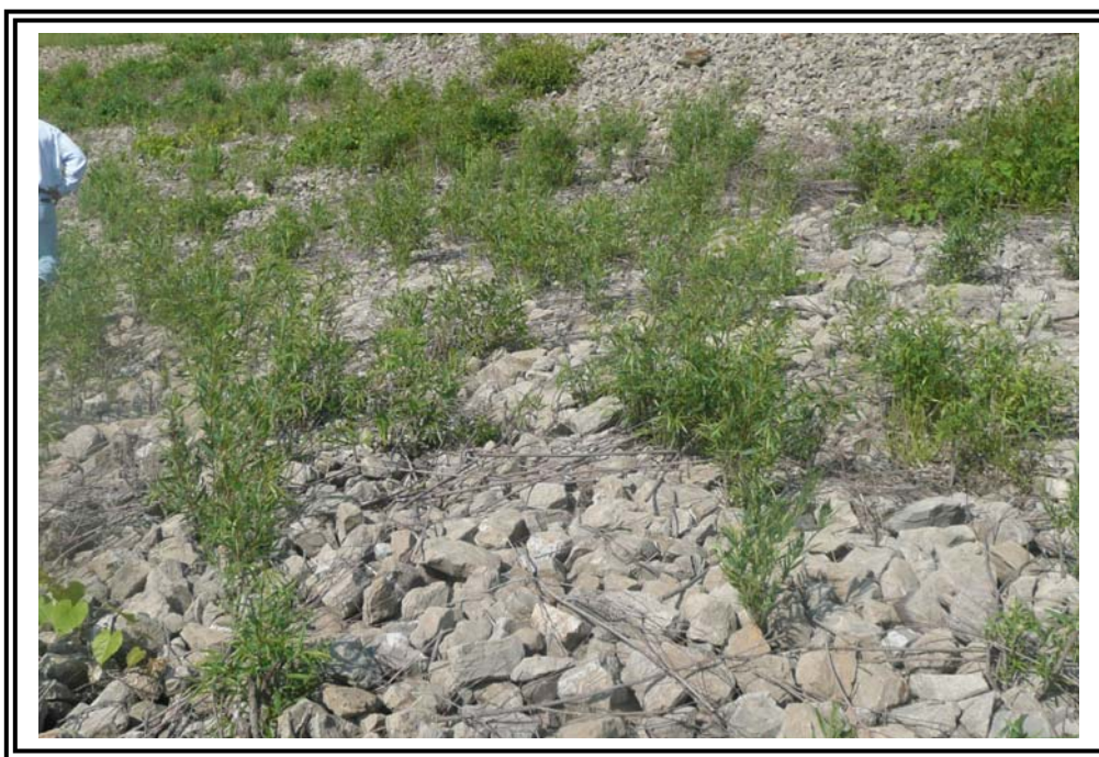
Vegetative growth within toe drain rip rap.
