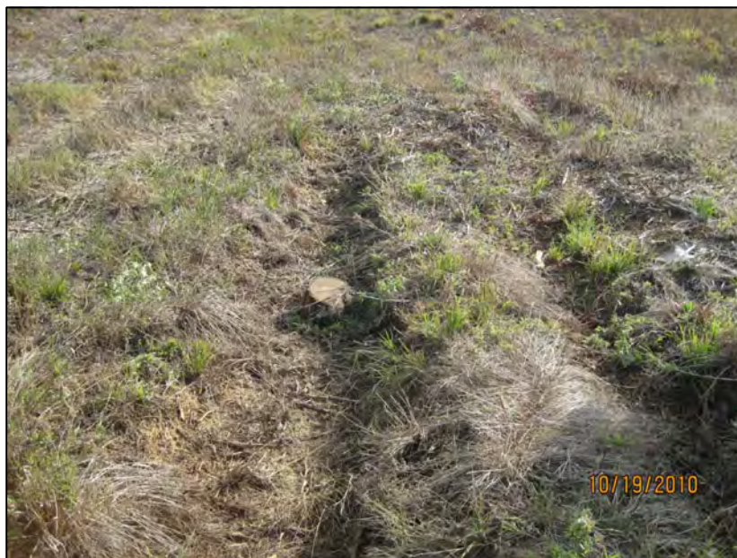
WAP-8 RUTS AND STUMP ON SOUTH EMBANKMENT
