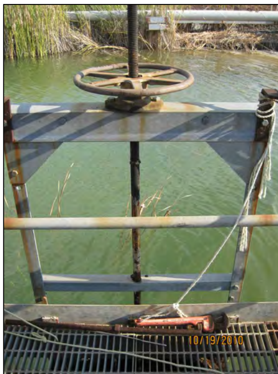
WAP-3 DISCHARGE PIPE VALVE OPERATOR
