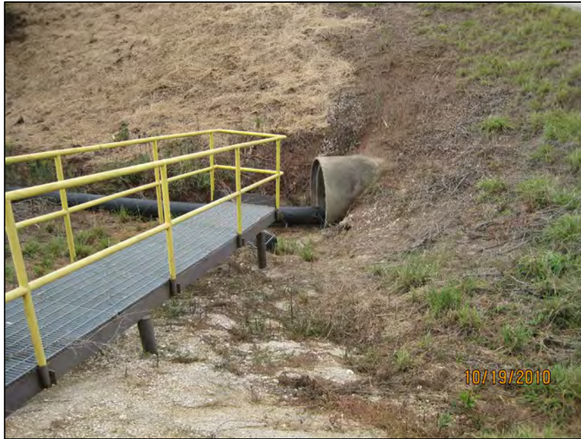
SAP-4 TRANSFER PIPE CARRYING REUSE FLOW TO ADJADENT LIGNITE MINE
