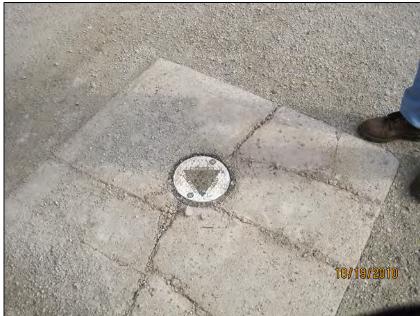
EAP-3 PIEZOMETER ON CREST OF NORTHERN EMBANKMENT
