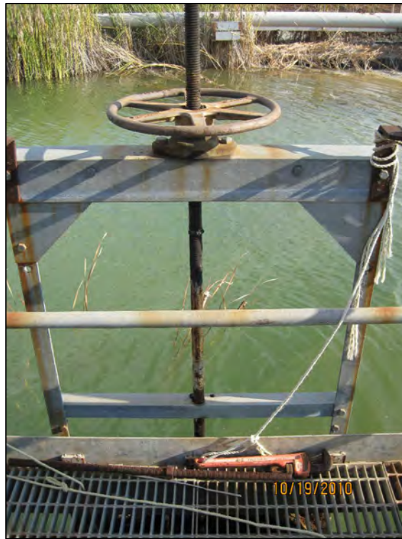
WAP-3 DISCHARGE PIPE VALVE OPERATOR
