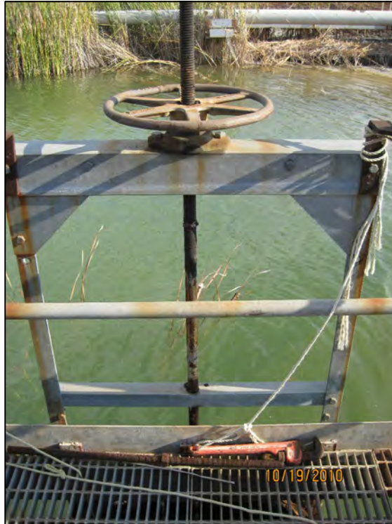
WAP-3 DISCHARGE PIPE VALVE OPERATOR
