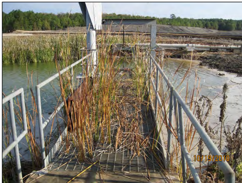
WAP-2 TOP OF DISCHARGE STRUCTURE
