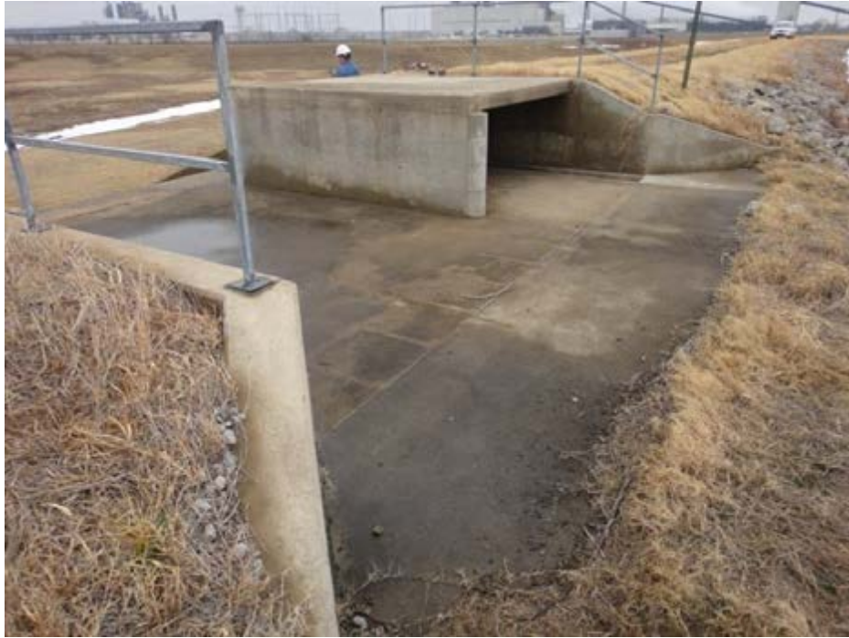
Figure 5.5.1-1. Inlet end of the Overflow Structure.
