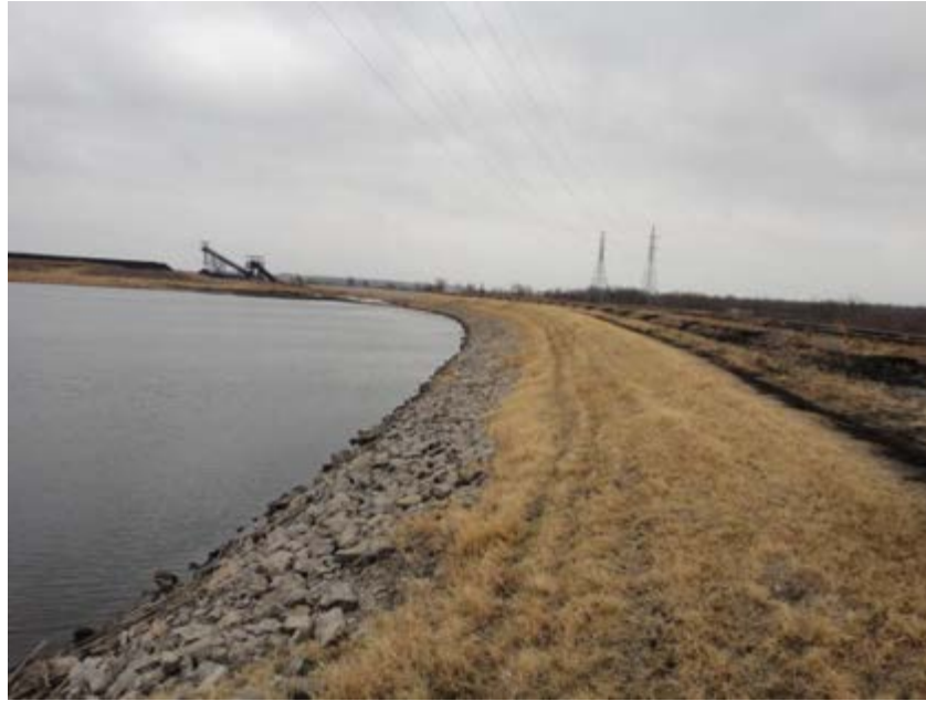
Figure 5.4.2-1. Conditions of inside slope of North Embankment.
