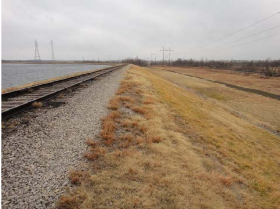
Figure 5.2.3-1. West Embankment outside slope condition.
