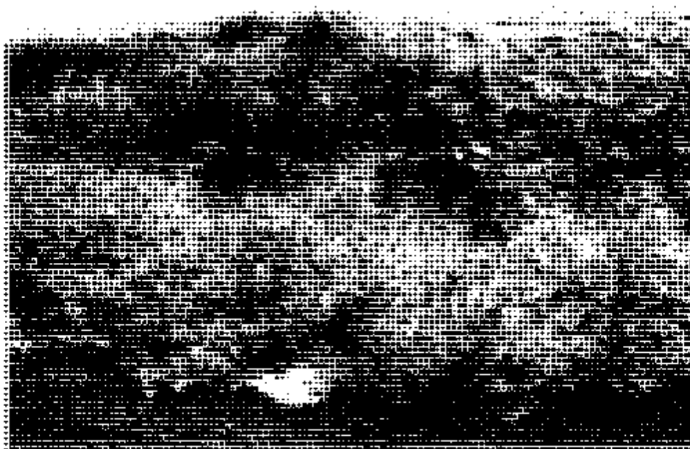
Photo 4. Outflow of the culvert that conveys emergency spillway discharge flow off site was partially blocked with minor vegetation.
