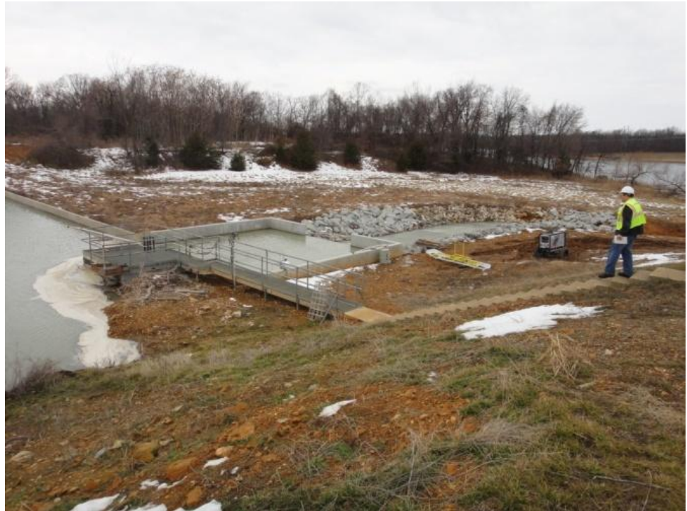
Figure 5.4.1-1. Main outlet structure
