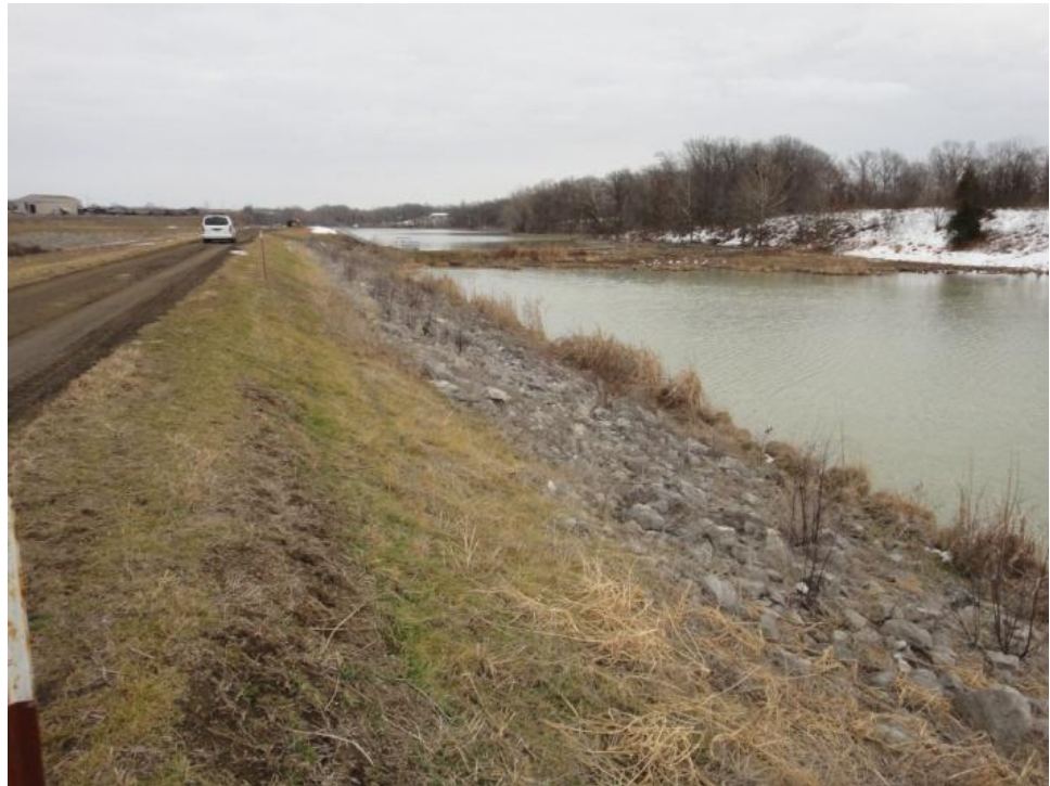
Figure 5.2.2-1: General condition of the inside slope, west dike
