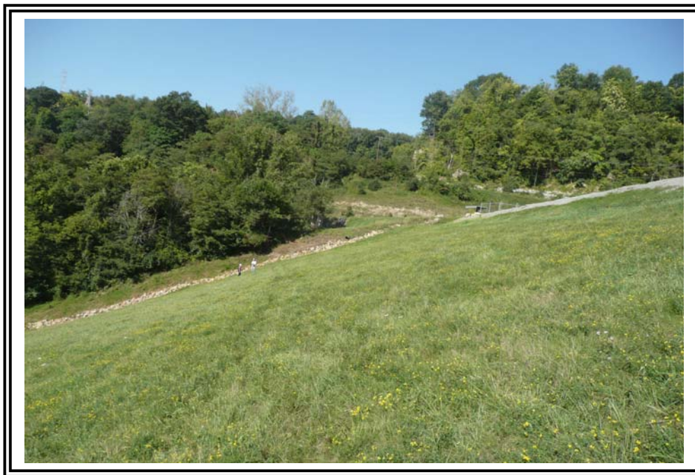
Downstream slope below crest, looking west towards right abutment. Note rock groin at abutment contact.
