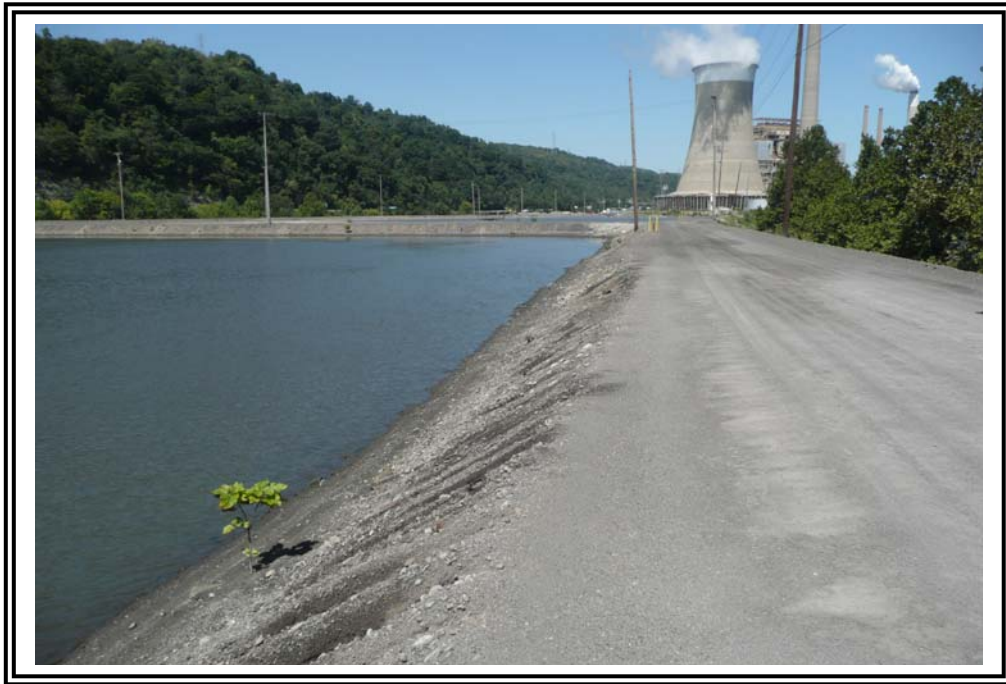
Crest and upstream slope of east dike at vinyl wall, looking north. Note typical erosion and sparse vegetation.
