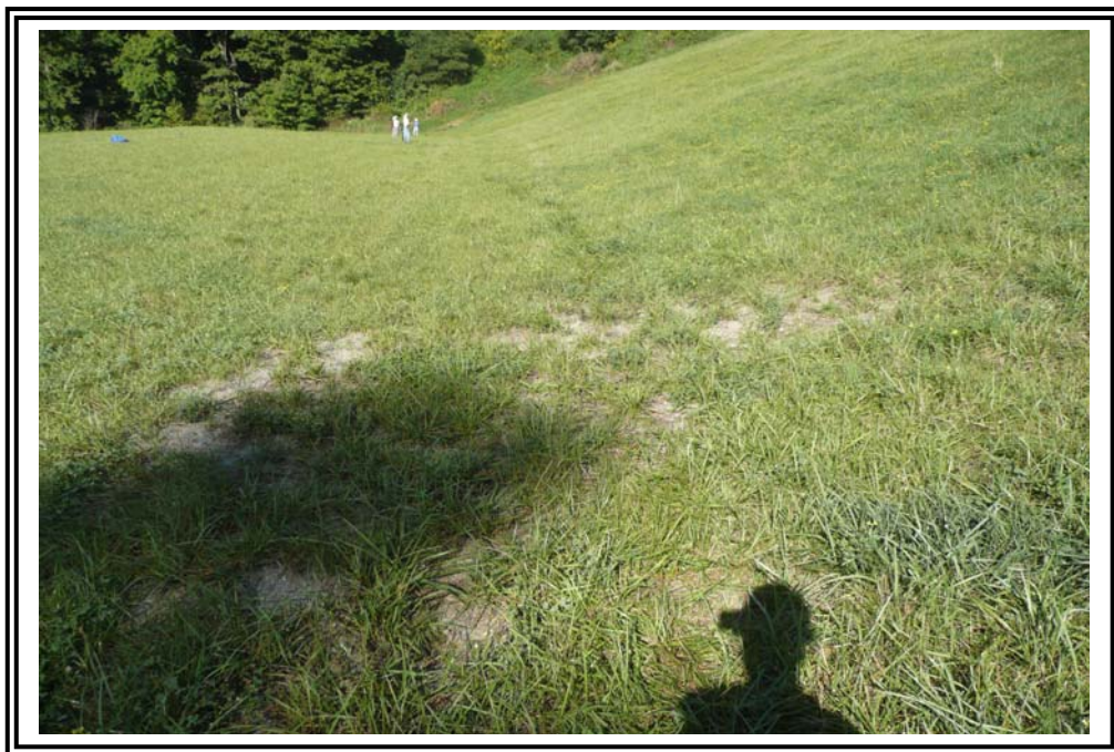
Sporadic loss of grass cover on upper bench adjacent to left (east) abutment.
