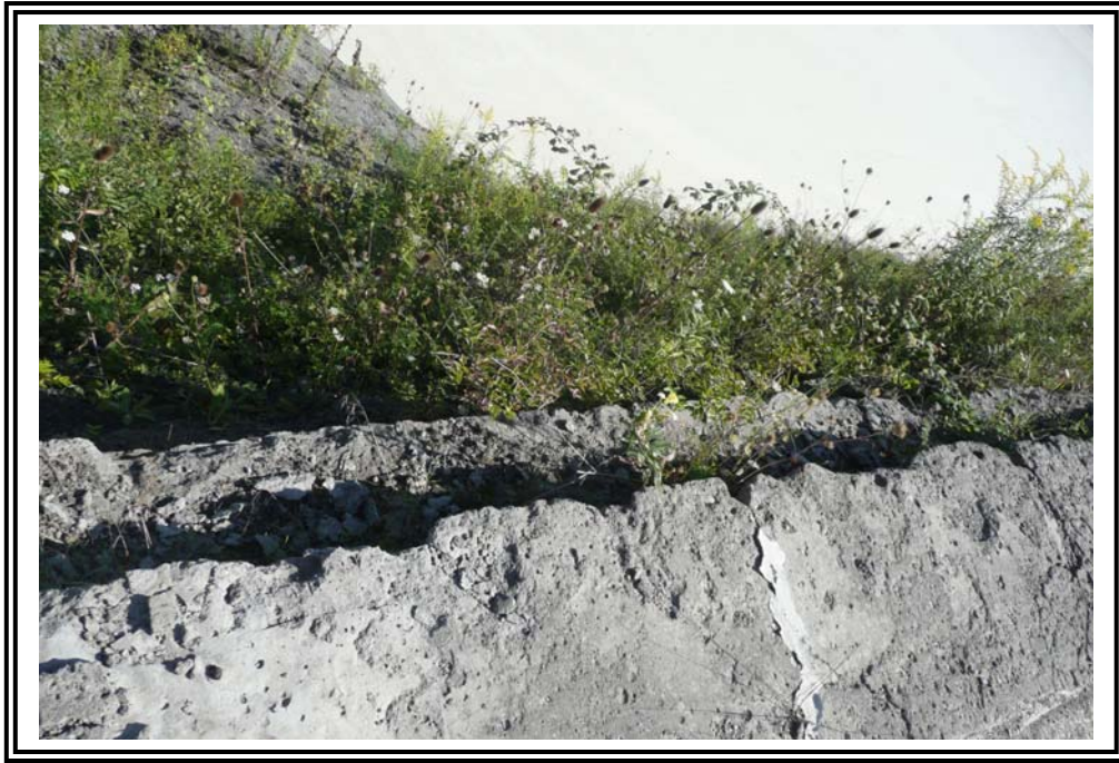
Close-up at weathered roller compacted concrete (RCC) surface and sealed crack on crest at upstream face. Note vegetation below crest level.
