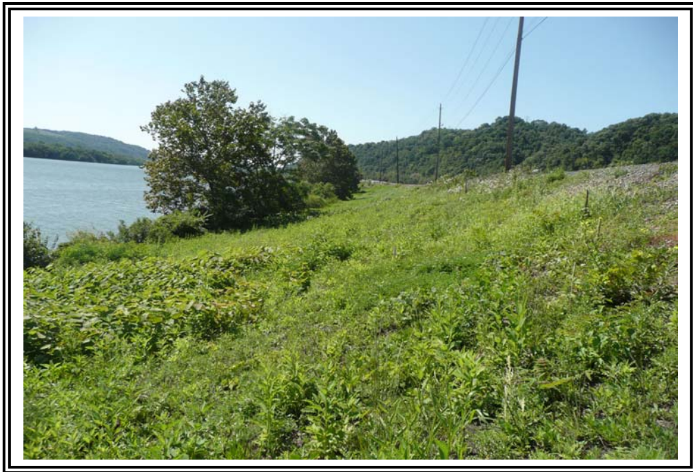
Downstream slope of east dike, looking south. Typical loss of vegetation shown at crest and change in vegetation shown adjacent to river bank.
