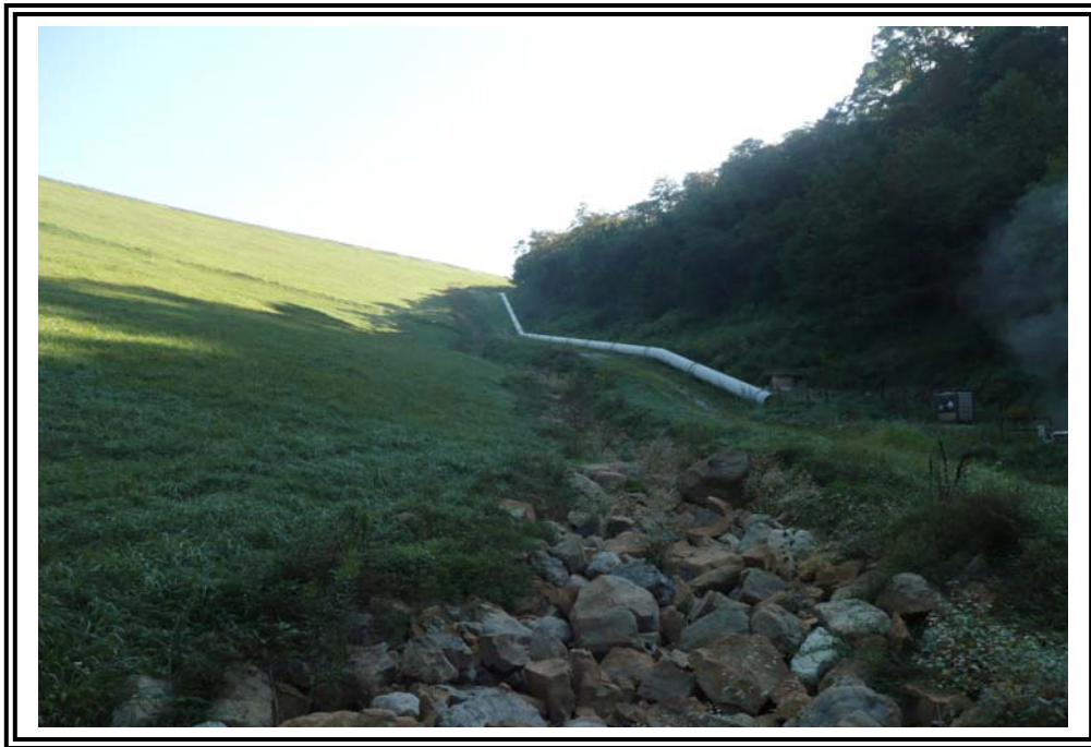
Looking upslope at left (east) rock groin and 42" diameter spillway outlet from toe drain.
