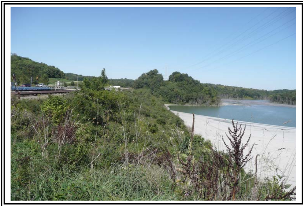
Downstream slope from right (south) abutment near crest. Note heavy wooded vegetation.
