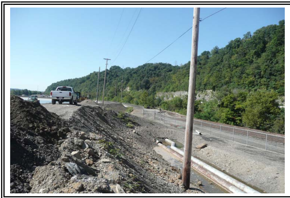
Downstream slope of the west dike looking south. Note water collecting around pipes in swale at slope toe which drains to the stormwater/wastewater and drainage sump in Photo # 9.
