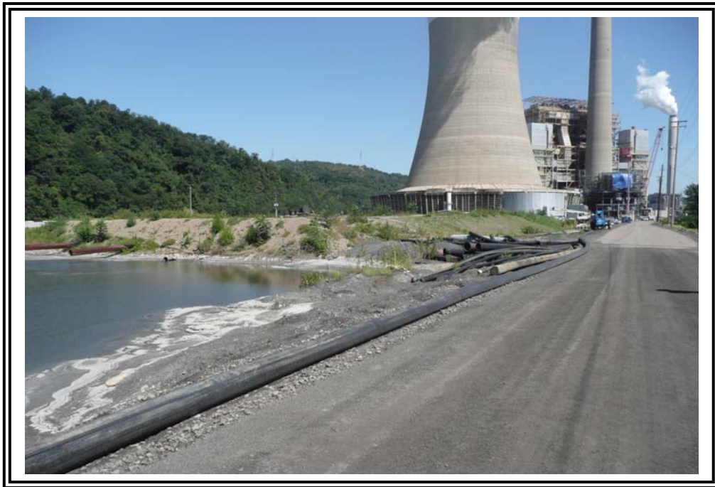
East dike crest alignment, pond surface, interior dike, chemical tank (in background) looking north.
