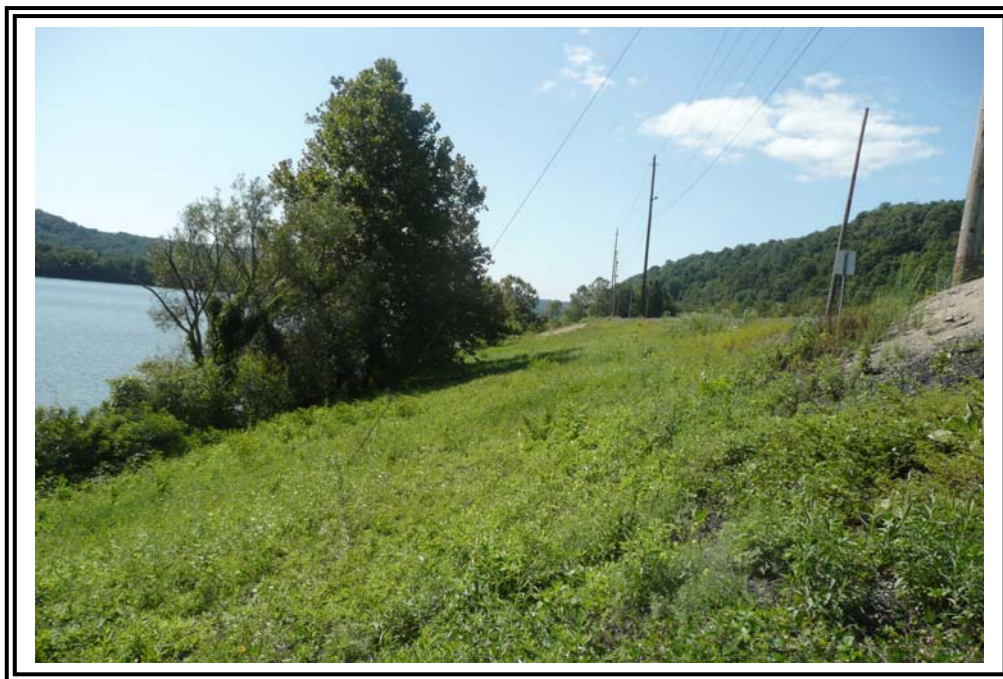
Downstream slope on east dike, looking south showing typical moderate, weedy vegetation cover on the slope face and larger brush with isolated trees at river bank.
