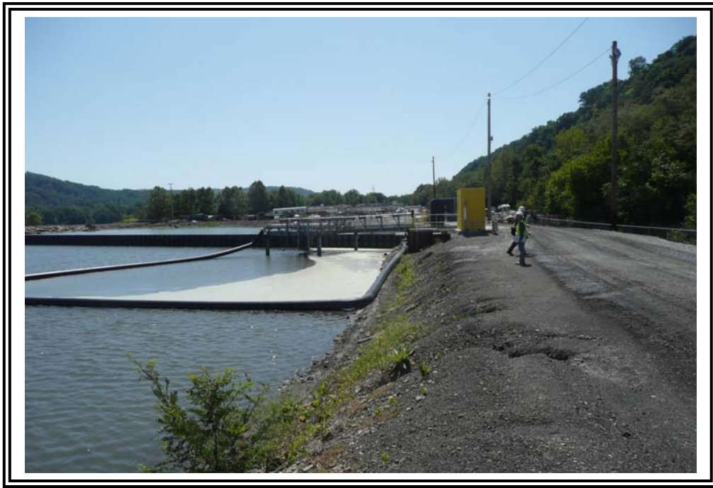
Upstream slope and crest of west dike, looking south. Note erosion feature and isolated brush. Vinyl sheet pile wall is in background.
