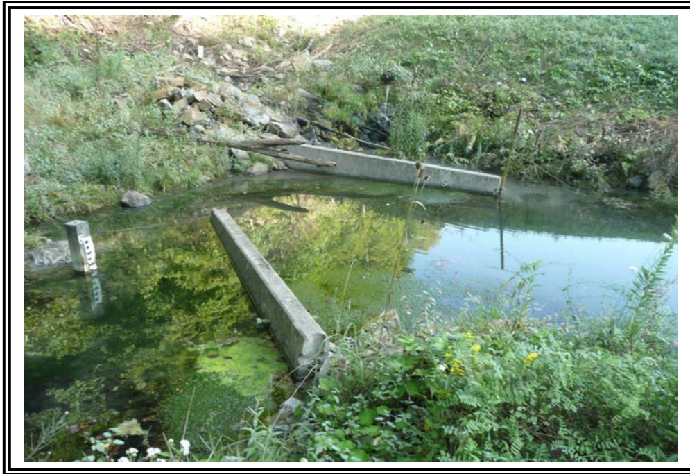
View of active toe drain discharge, seepage collection pool, and concrete baffles.
