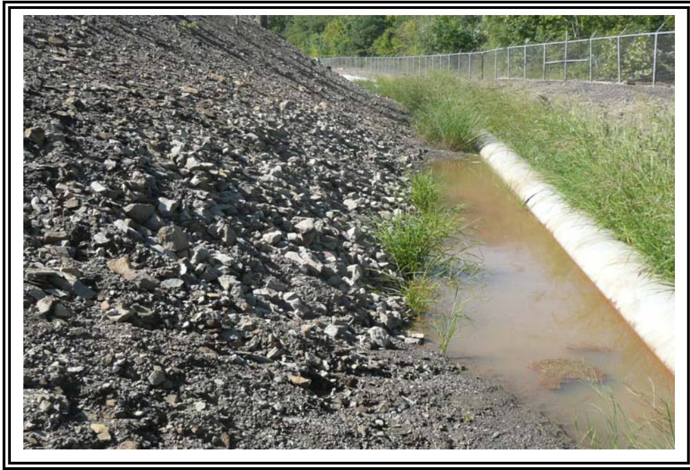
Toe of west dike where drainage has collected in pipe swale, looking south. Soil difficult to probe more than a few inches.
