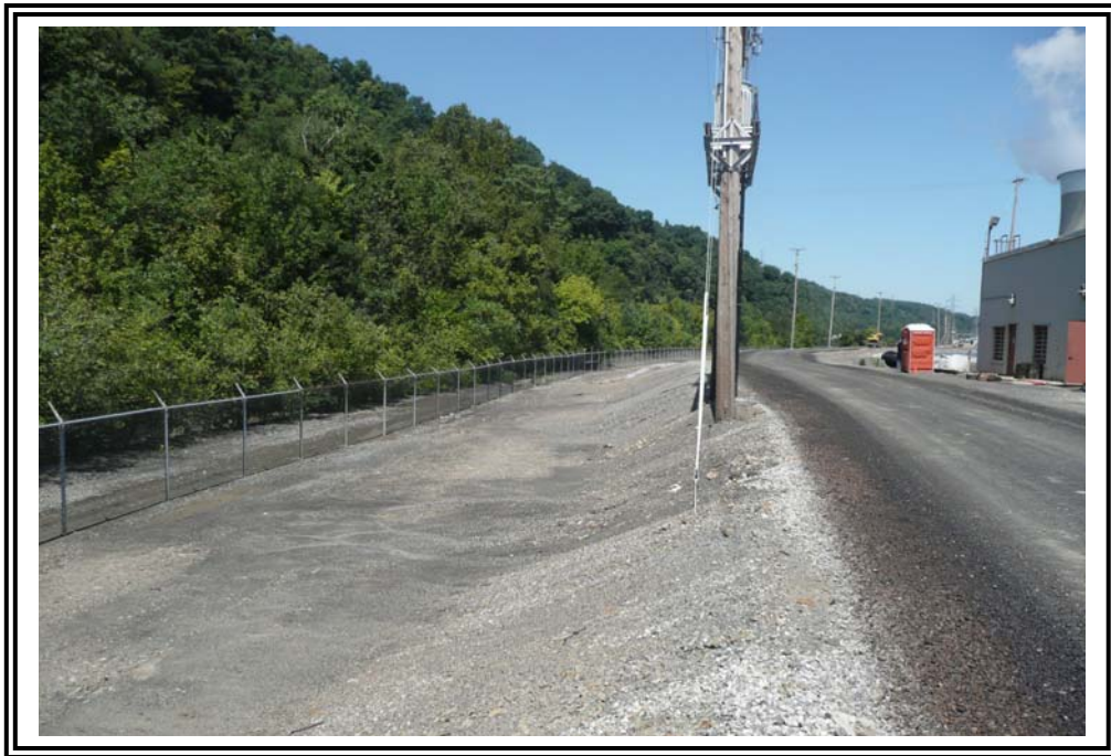
Downstream slope of west dike, looking north. Note fairly low height (about 5 feet tall) at this point.
