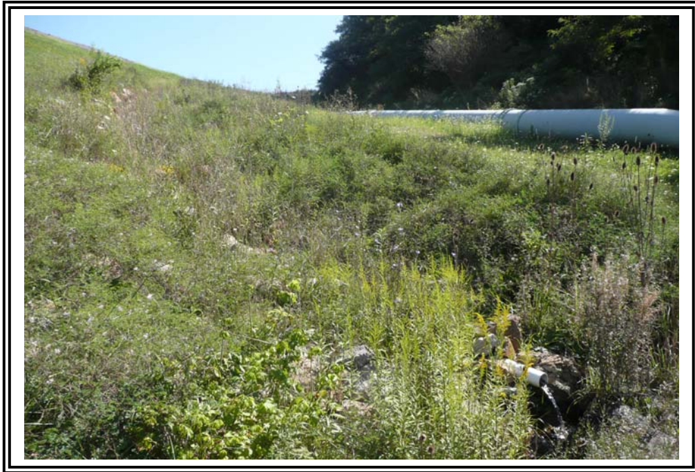
Active seepage outlet in left (east) rock groin. Water flowed clear.
