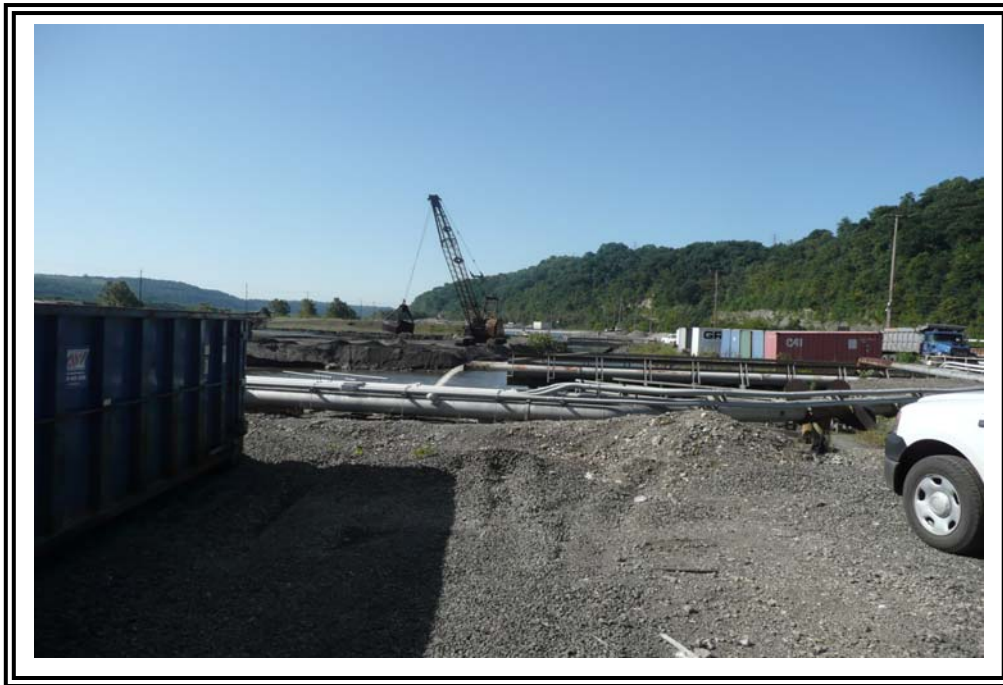
North rim of bottom ash pond at ash lines looking south. Note crane on ash delta platform.
