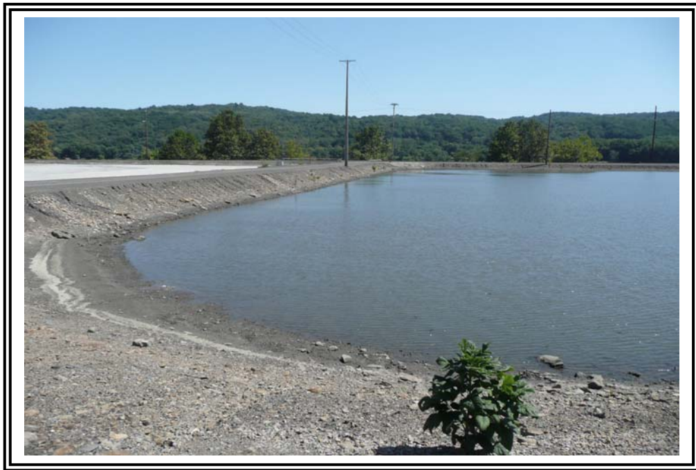
Downstream slope of the separator dike on the north side of the pond. Erosion features noted in separator dike slope.
