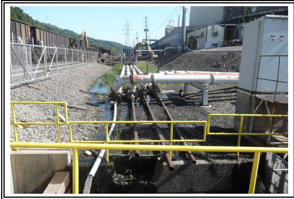
Looking north from the yard sump at the drainage swale along the downstream toe of the west dike.
