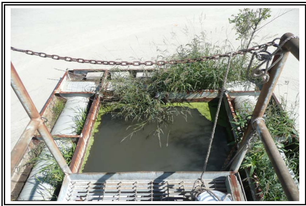
Closer view of skimmer at spillway tower and vegetation beginning to establish itself.
