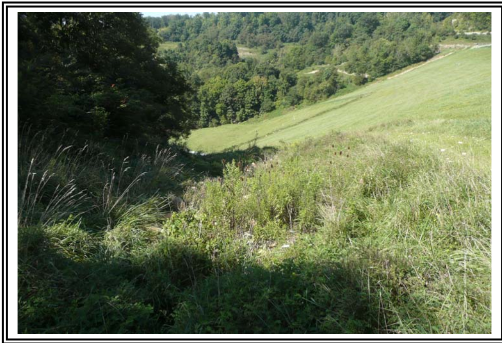
Left (east) rock groin at abutment contact. Note moderate to heavy vegetation.
