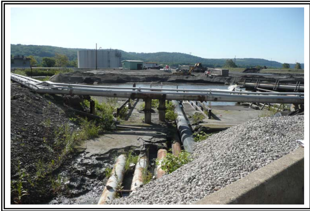
View of ash delta working platform from north dike. Note dredge spoil dike in background.
