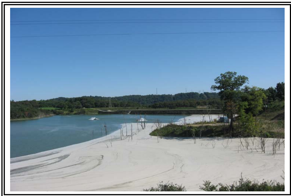
Looking east from crest across Fly Ash Reservoir No. 2 at Fly Ash Dam No. 2.
