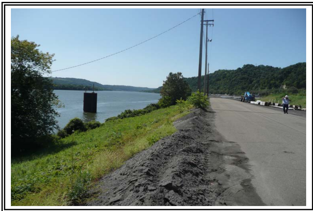
East dike crest alignment, looking south, showing ash build up at road edge due to grading activities.
