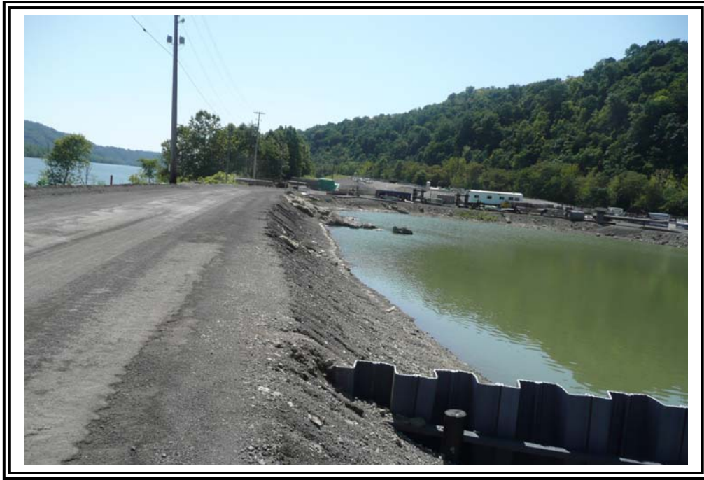
Crest and upstream slope of east dike at vinyl wall, looking south.
