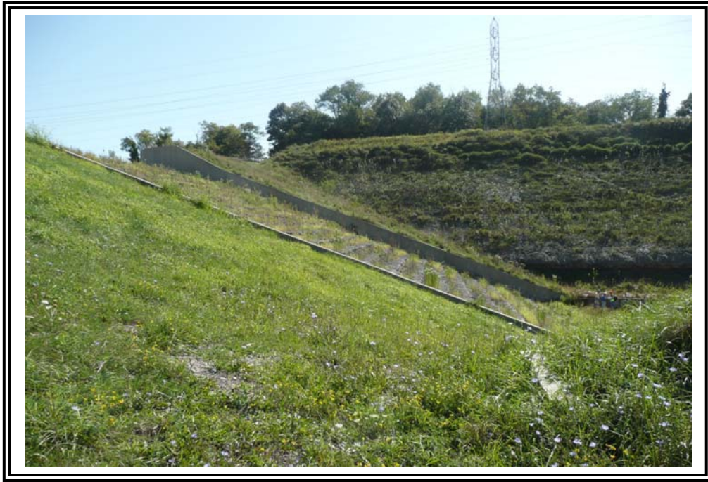
Downstream slope on RCC portion looking toward emergency spillway and left (east) abutment. Bedrock is exposed in far slope.
