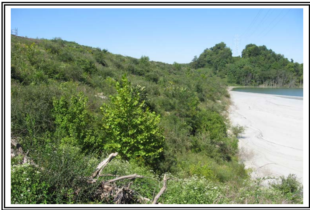
Downstream slope from right (south) abutment, closer to Fly Ash Reservoir No. 2 water surface.
