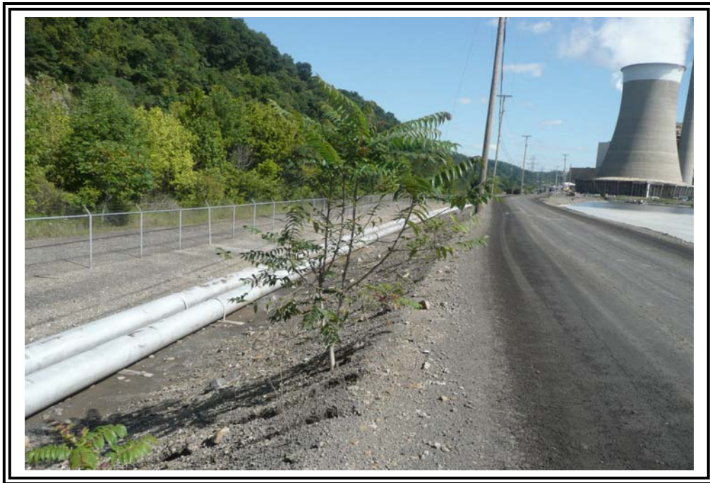
Wooded vegetation becoming established on downstream slope of west dike, looking north.
