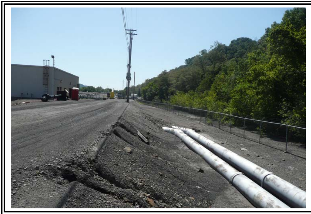
Crest and downstream slope at west dike, looking south where recirculation pipes exit slope. Typical erosion features evident at crest.
