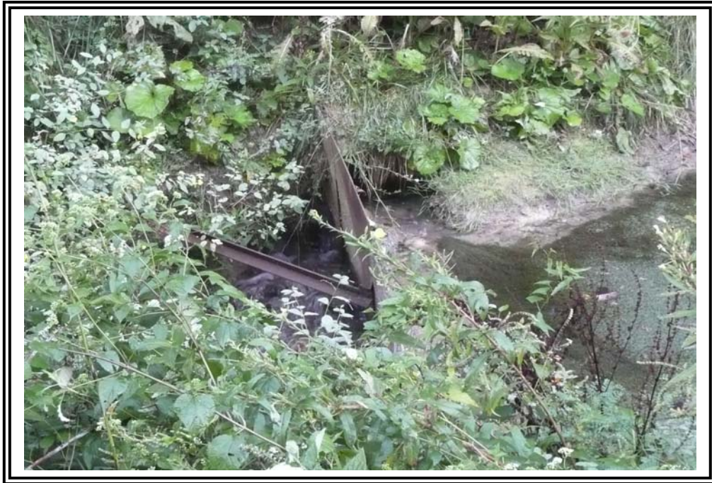
Ineffective steel V-notch weir where water flows along seepage path around weir.
