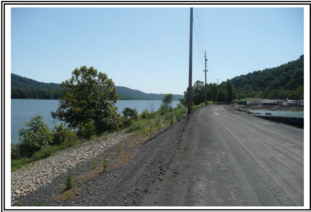
Crest and downstream slope of east dike, looking south. Note vertical limit of stone facing.
