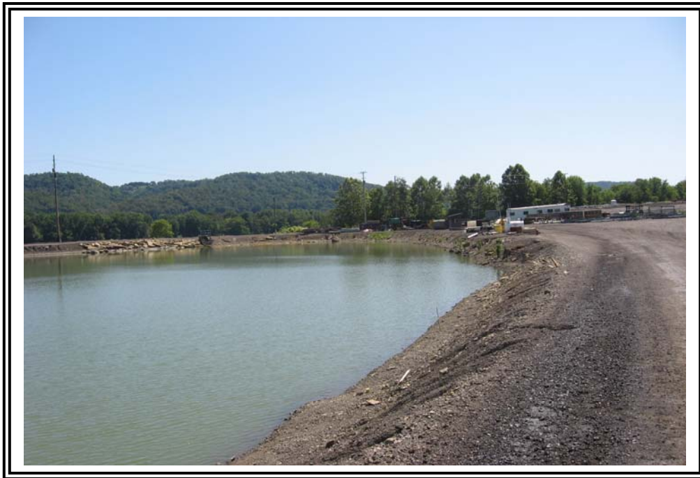
Inboard face at south wall, looking east. Pond is essentially incised in this location.
