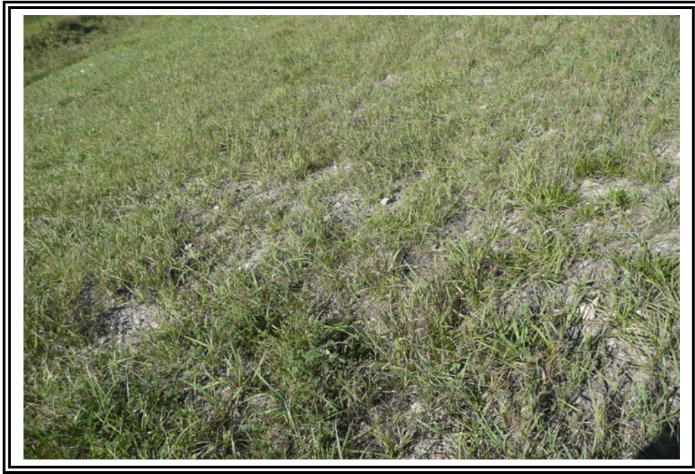
Isolated loss of grass cover and possible erosion on upper portion of downstream slope above slope groin.
