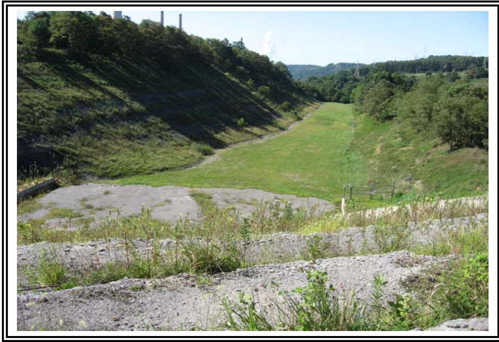
Emergency spillway, looking south from crest. Note that this spillway is excavated through hillside.
