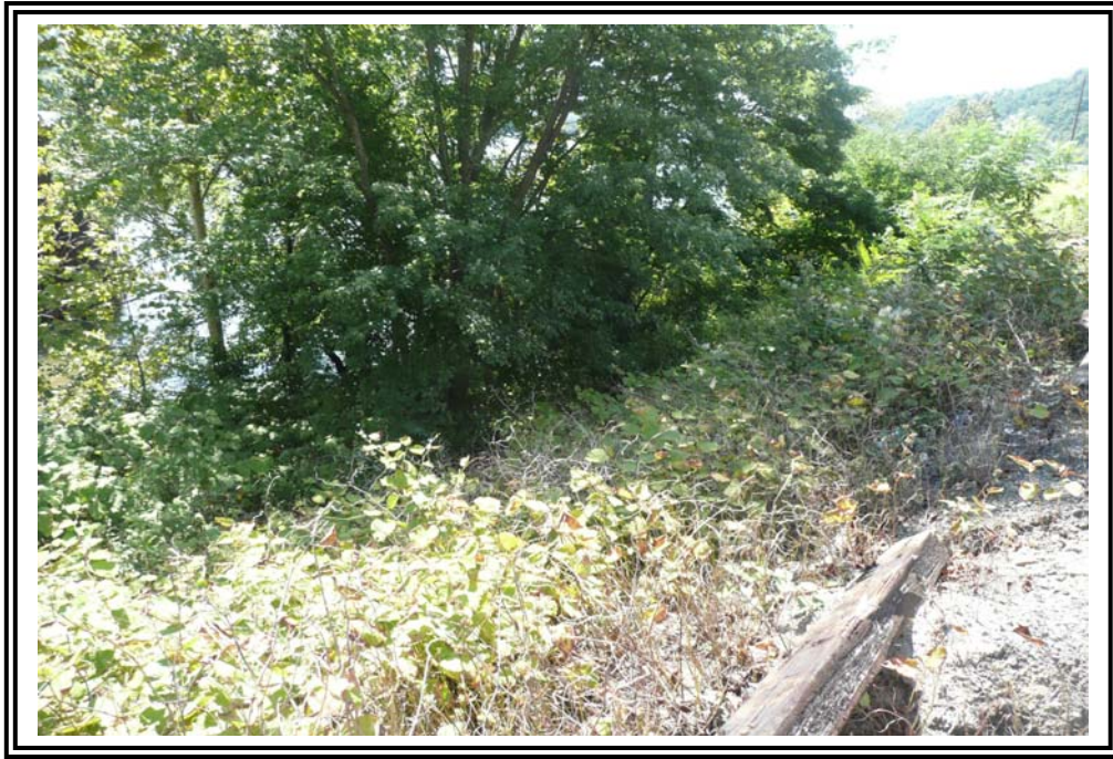
Downstream slope of east dike at northern extent of pond showing heavy vegetation and debris.
