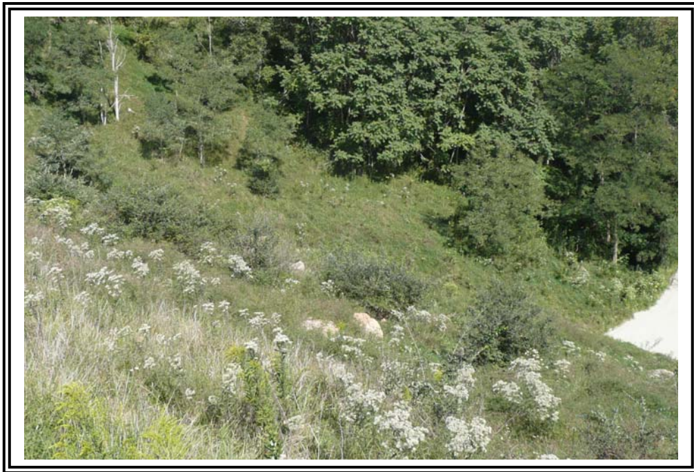
Downstream slope showing sporadic rip-rap (boulders).
