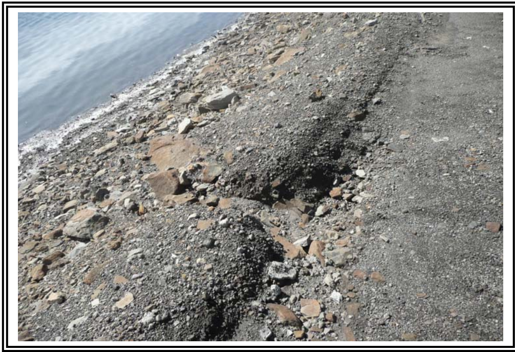
Up-close view of erosion noted in Photo #11 showing large rock fragments in dike material.
