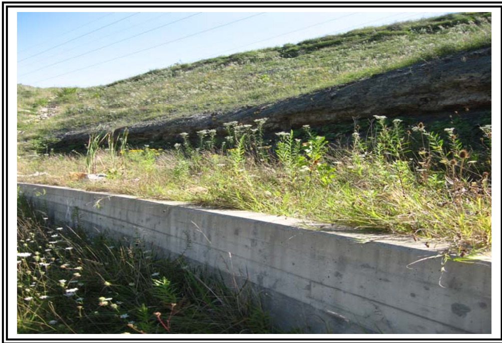
Left (east) concrete training wall at emergency spillway outfall channel. Note exposed bedrock.
