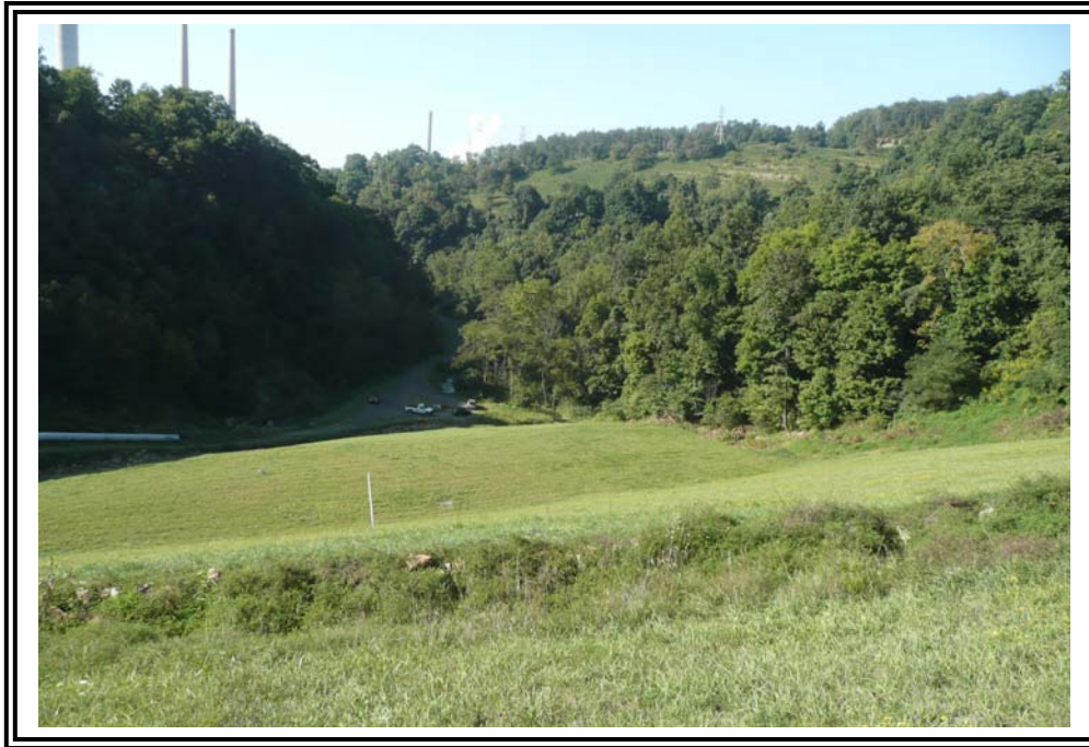
Another view of slope groin and general slope grass cover, looking downstream.
