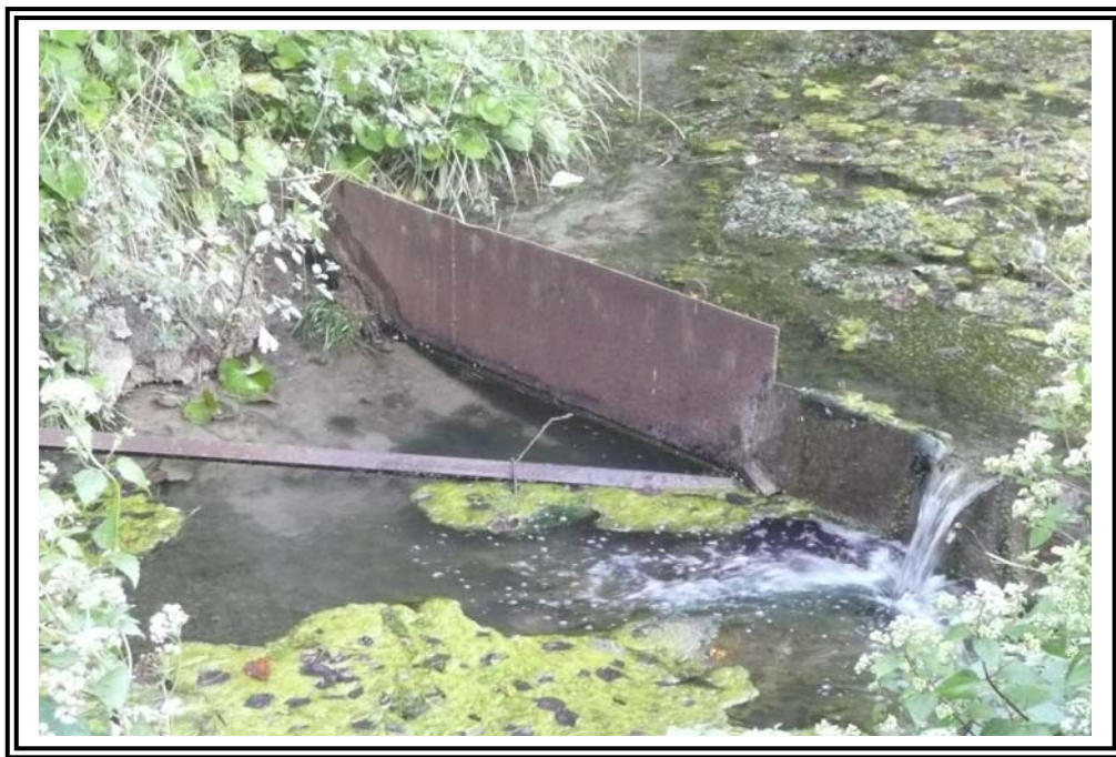
Steel V-Notch weir (typical) noted downstream of concrete weir shown in Photo #93.
