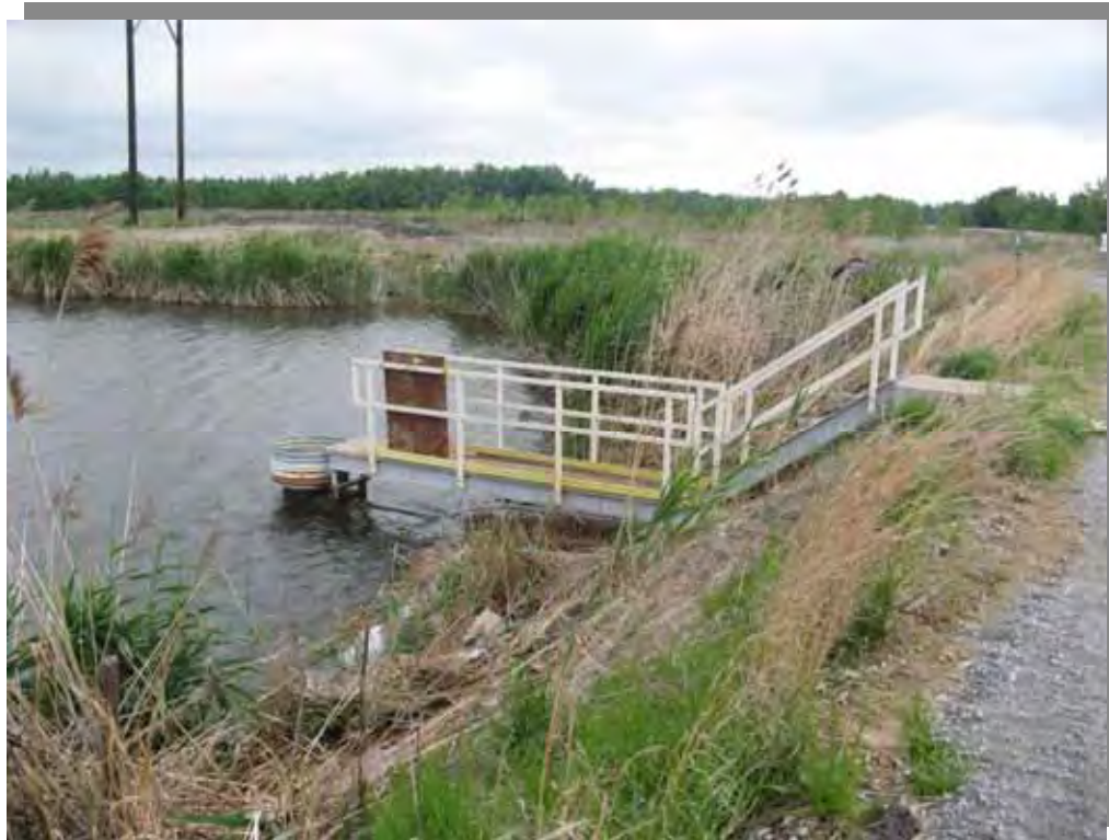
Photo 15 – Southern Pond primary outlet structure.
