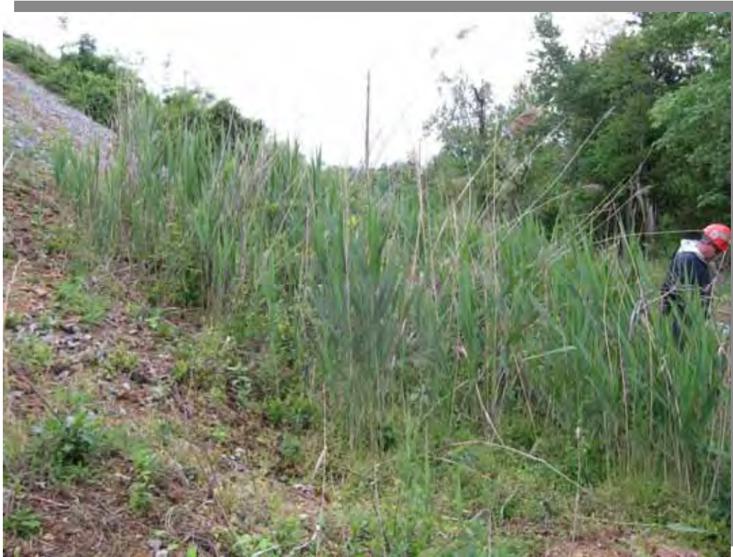
Photo 23 – Outboard toe of Southern Pond eastern embankment approximately 500 feet north of power lines. Note reedy grasses indicating moist conditions, signs of seepage.
