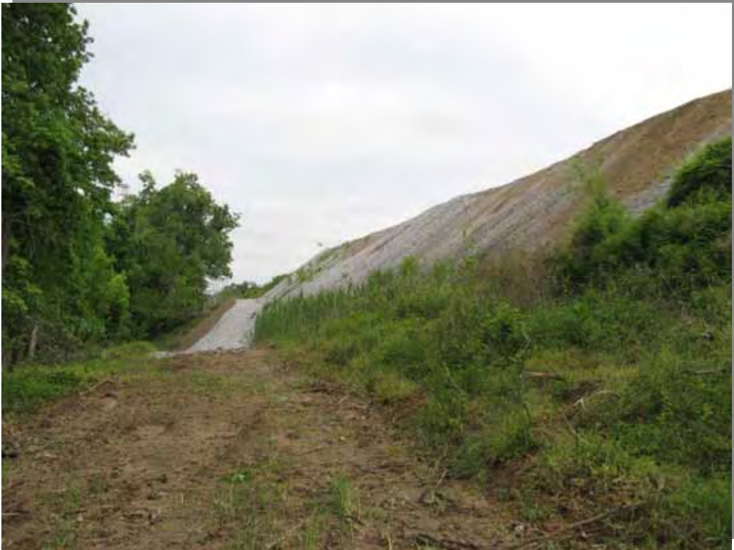
Photo 19 – Outboard slope of eastern embankment of Southern Pond. Note repairs near crest and partially completed access road along toe.
