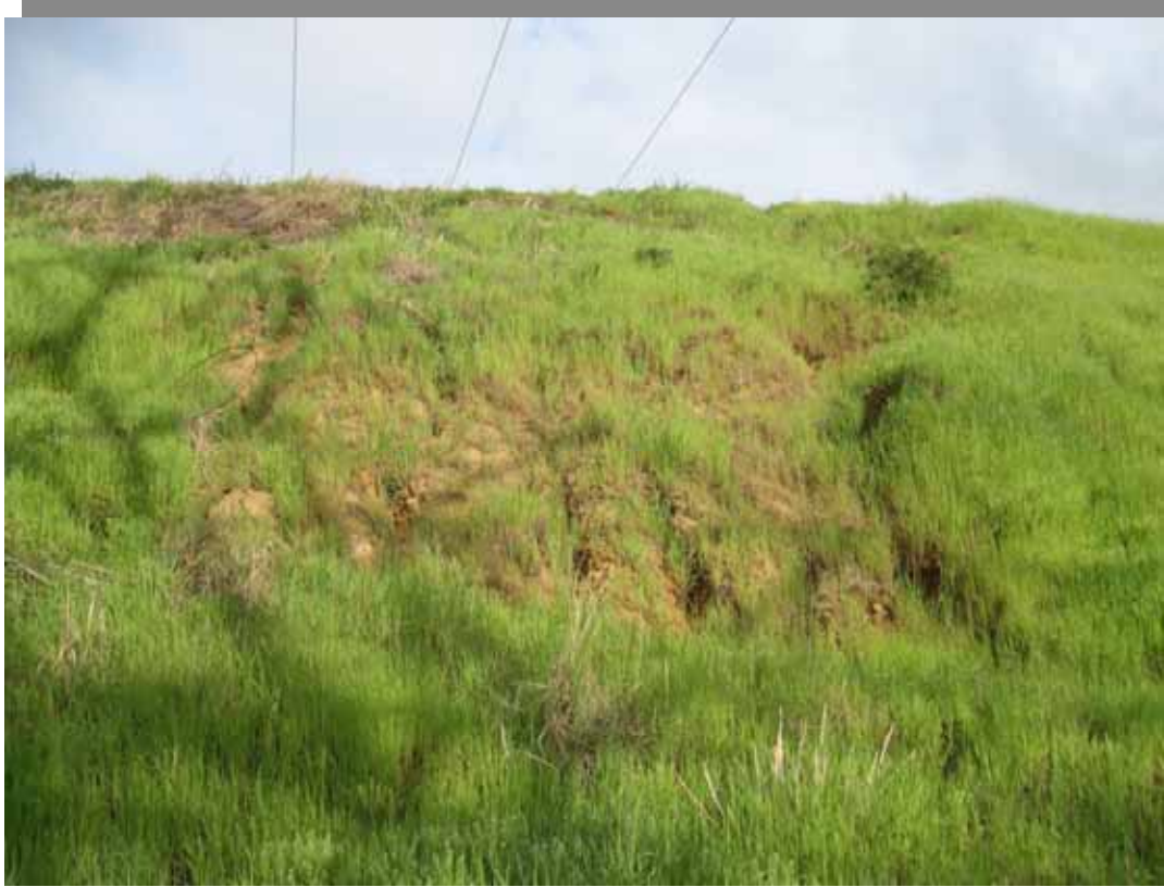
Photo 21 – Erosion on east embankment of Southern Pond below the power lines.
