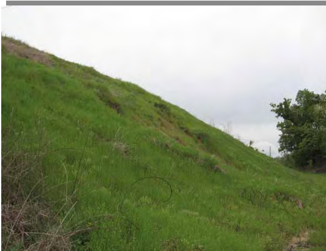
Photo 22 – Slides and sloughs on east embankment of Southern Pond, approximately 200 feet south of power lines.
