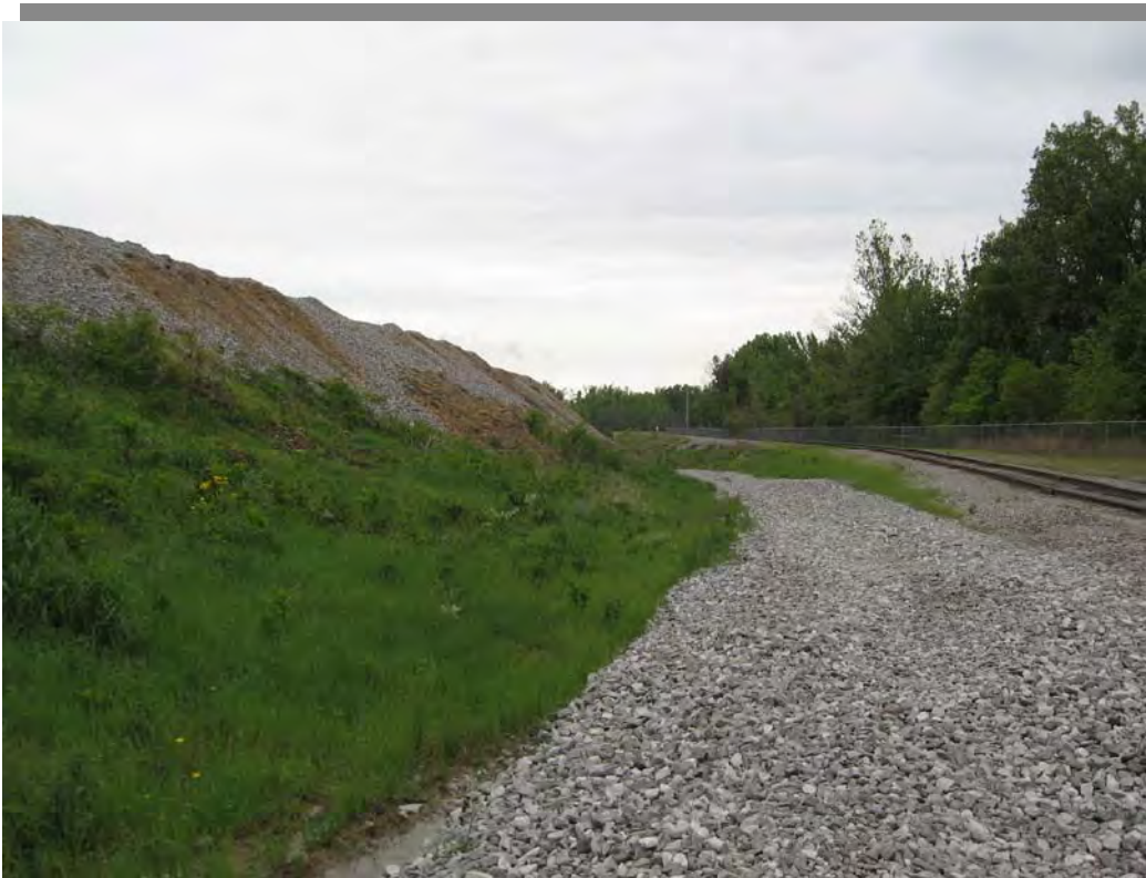
Photo 7 – Outboard slope of Northern Pond near the northern end. Note repairs near the crest.
