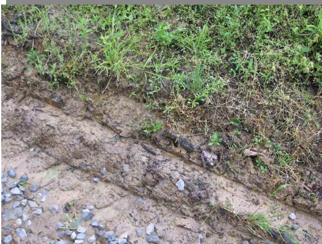
Photo 24 – Seepage at toe of east embankment of Southern Pond, near location indicated in Photo 23 above.
