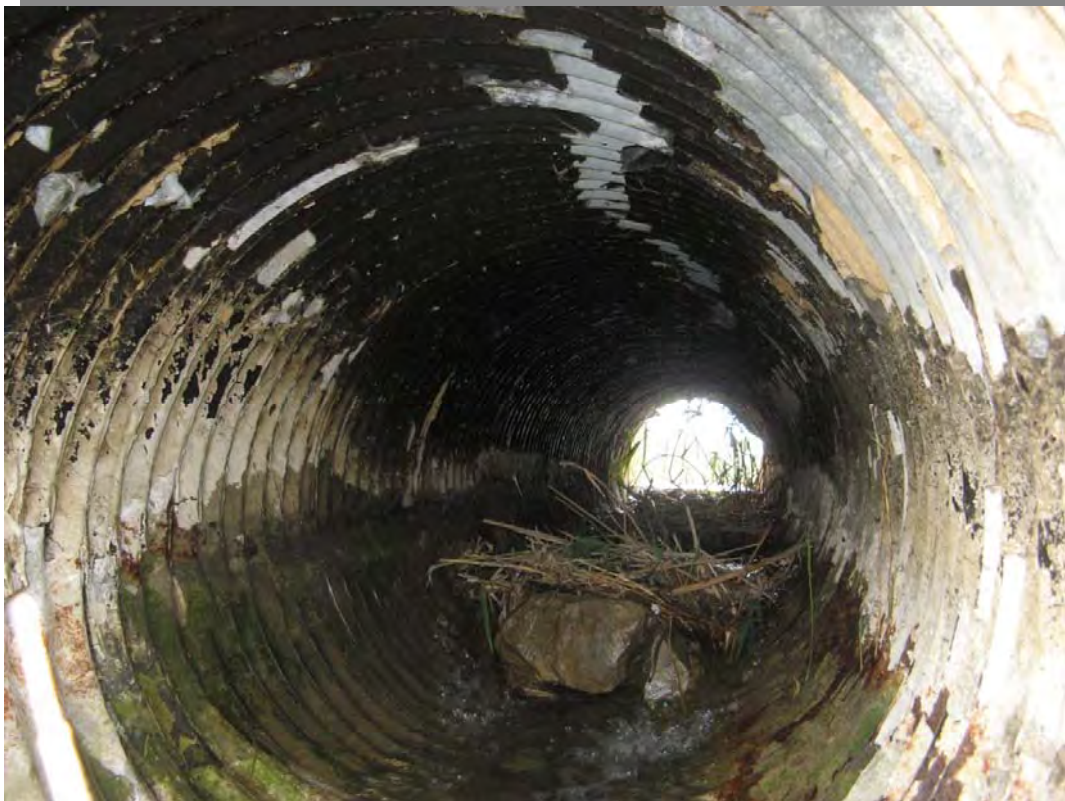
Photo 3 – Interior of Central Dike Culvert. Note riprap “dam” limiting pipe’s capacity.
