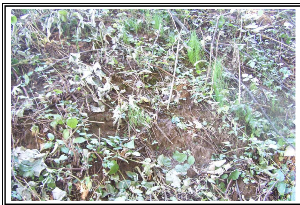
Erosion/surficial sloughing on east dike at Pond #4. Surface soil soft.
