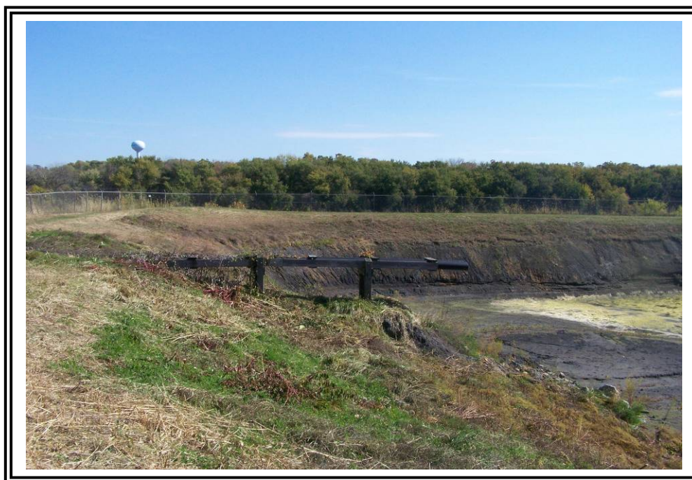
Upstream slope of north dike at Pond #3, looking east. Irregularity of slope related to remaining ash from recent dredging operations.
