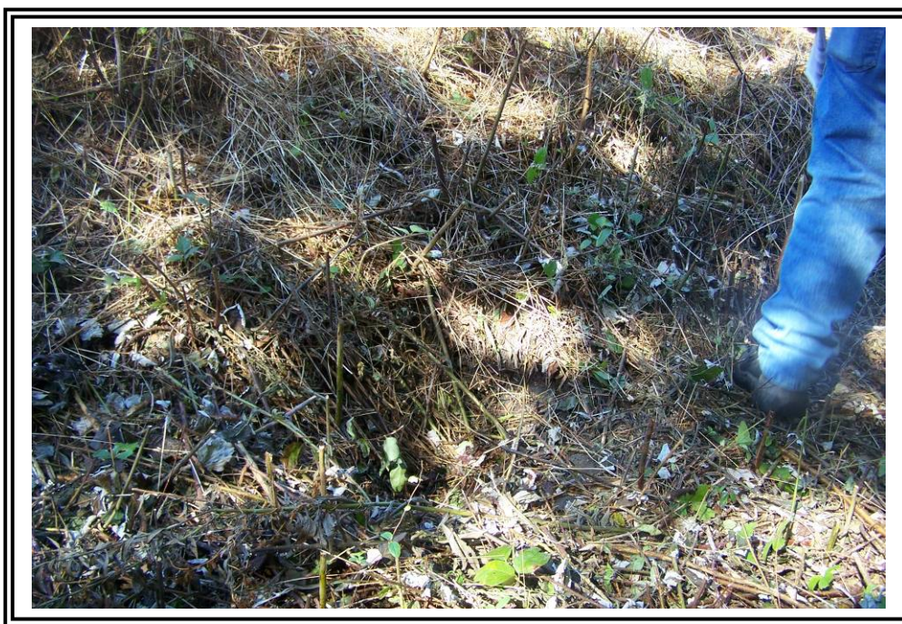
Filled in rodent holes on east dike at Pond #4. Rodent control is performed each spring and observed holes are filled as part of routine maintenance of the dikes.
