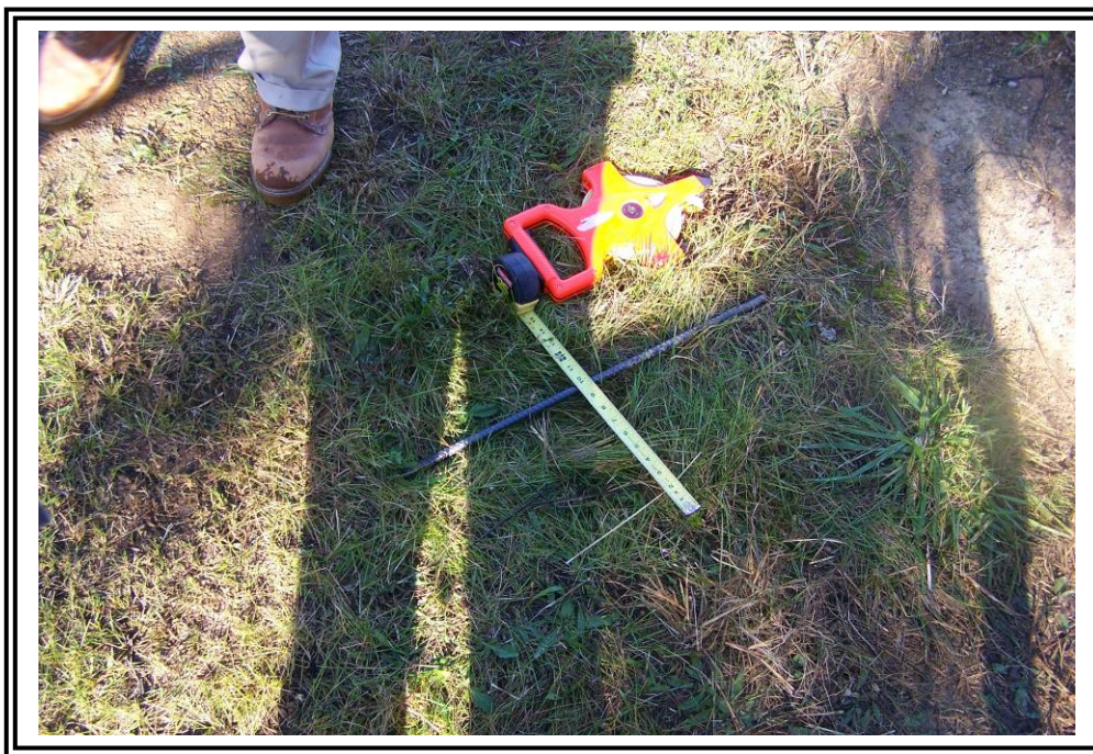
Depression about 2 inches deep and 18 inches in diameter on crest of east dike in approximate area of outlet pipe.
