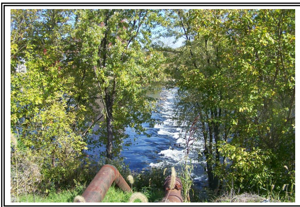
Slice lines from R Paul Smith Station traverse the Potomac River are hardened steel and protected with rip rap. The sluice lines are replaced approximately every 15 years as routine maintenance.
