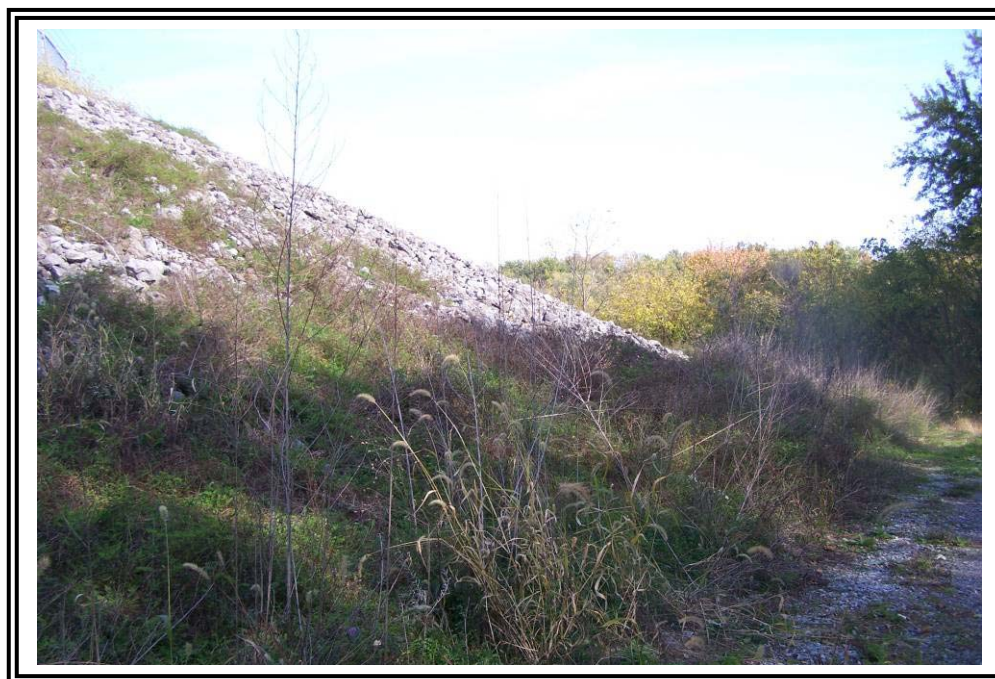
Typical patchy vegetation on rip rap armor of downstream slopes of Pond #3. Mostly grasses, occasional saplings.
