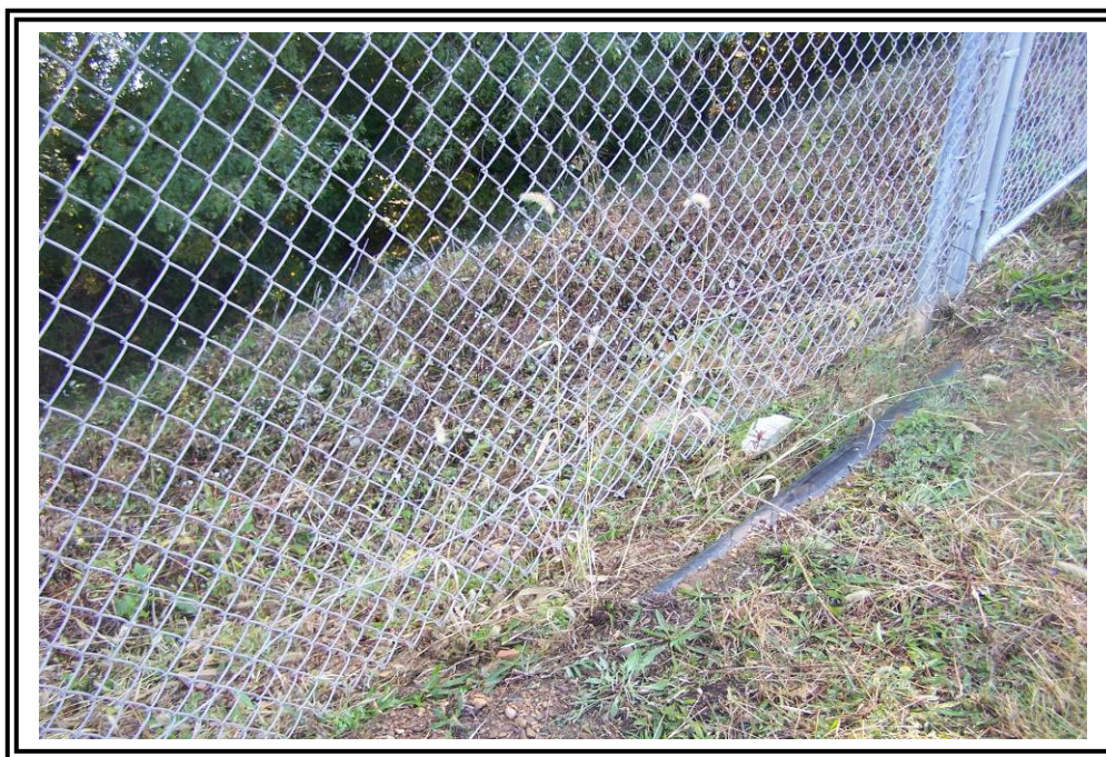
Surface erosion at downstream slope/crest on east dike at Pond #4. This erosion has been noted in previous inspection reports and has not changed in many years.
