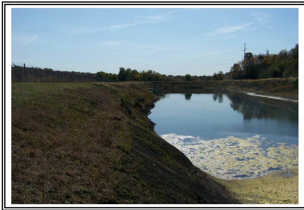
Upstream slope of east dike at Pond #3, looking south. Irregularity in slope related to over excavation during recent dredging operations.
