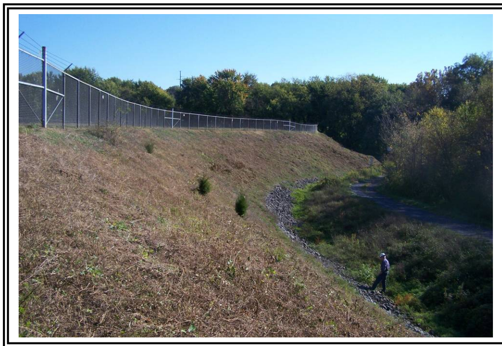
Small trees on downstream slope on south dike at Pond #4, looking east.
