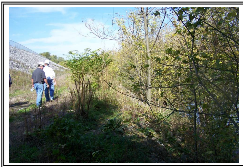
Trees growing in stone buttress on east dike of Pond #3, looking north.
