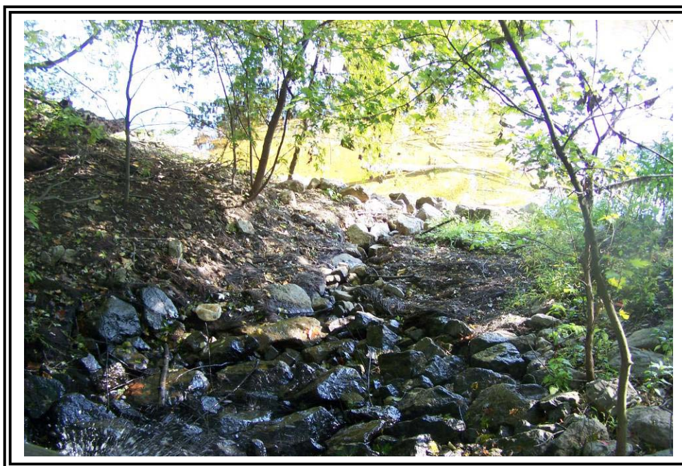
Rip rap channel from the Pond #4 outlet to the Potomac River.
