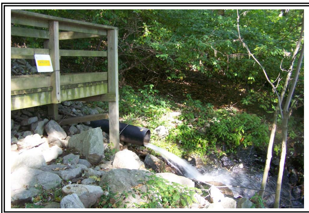
Discharge pipe from Pond #4.
