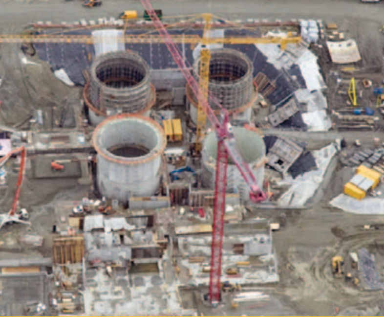
Construction of Three Digesters and a Mixing Tank for the Brightwater Treatment System
