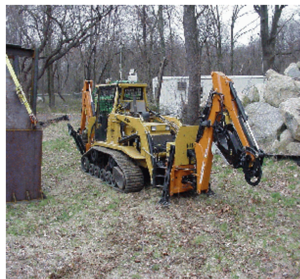
Figure 2 Remote Control Equipment
