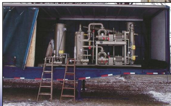
Multi-phase extraction trailer
