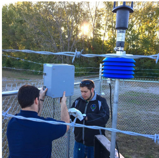
Tim McArthur (left) and Alex Korff of Science Systems and Applications, Inc. make final adjustments during the installation of the portable, low-cost air monitors (P-pods) in Kansas City, Kansas, on October 18, 2017, for a year-long air monitoring study. Photo credit: EPA Region 7 Digital Team.
