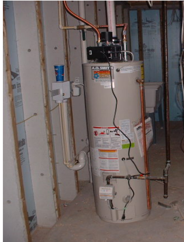
POWER VENTED WATER HEATER
