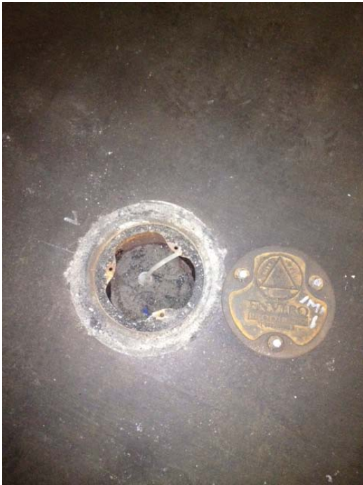
Vapor monitoring point; typical of VMP-1, 2, 3 and 10
