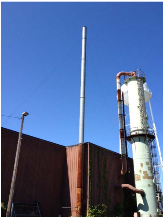
Air discharge stack and groundwater air stripper
