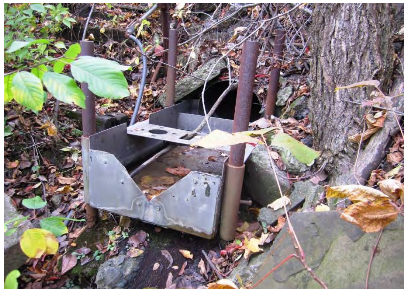
This is one of two outfall pipes that were discharging polluted waters into the Cuyahoga River from the BASF site. BASF obeyed a U.S. EPA order to stop the discharges that contained heavy metals and uranium.
