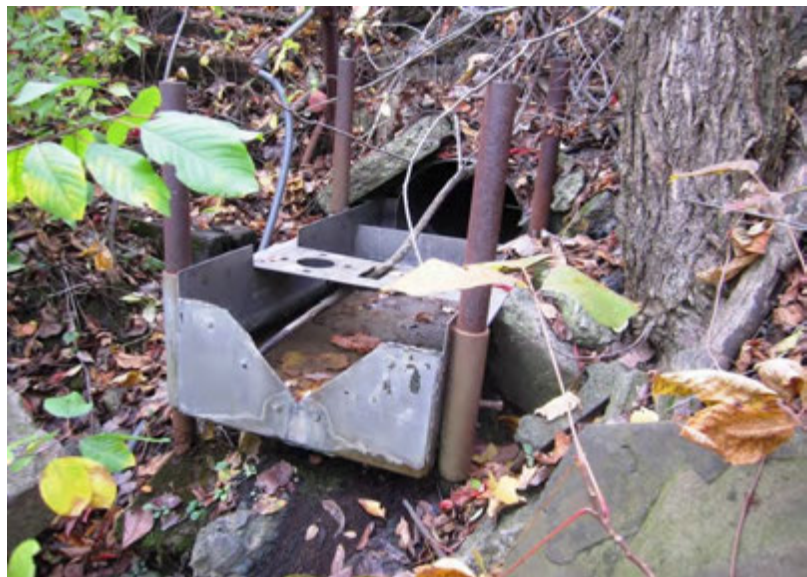
This is one of two outfall pipes that were discharging polluted waters into the Cuyahoga River from the BASF site. BASF obeyed a U.S. EPA order to stop the discharges that contained heavy metals and uranium.
