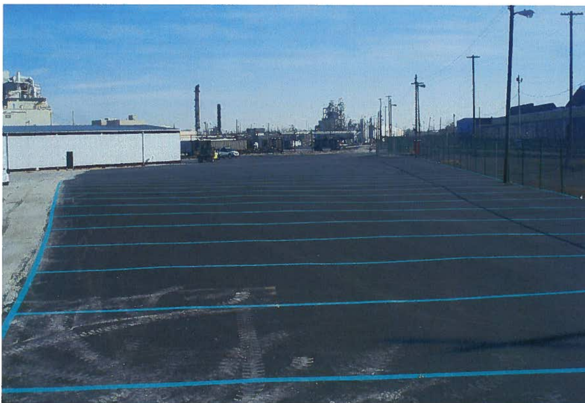
Photo # 45 Looking northeast from southwest corner of Plant at S0609 paving area.
