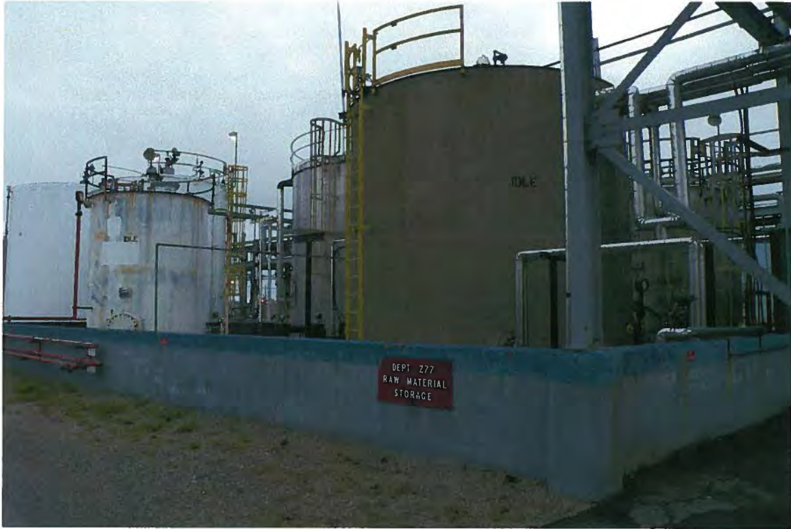
Photo # 1 Looking northeast at North Tank Farm. Samples B-39 and B-40 were collected inside concrete containment area.
