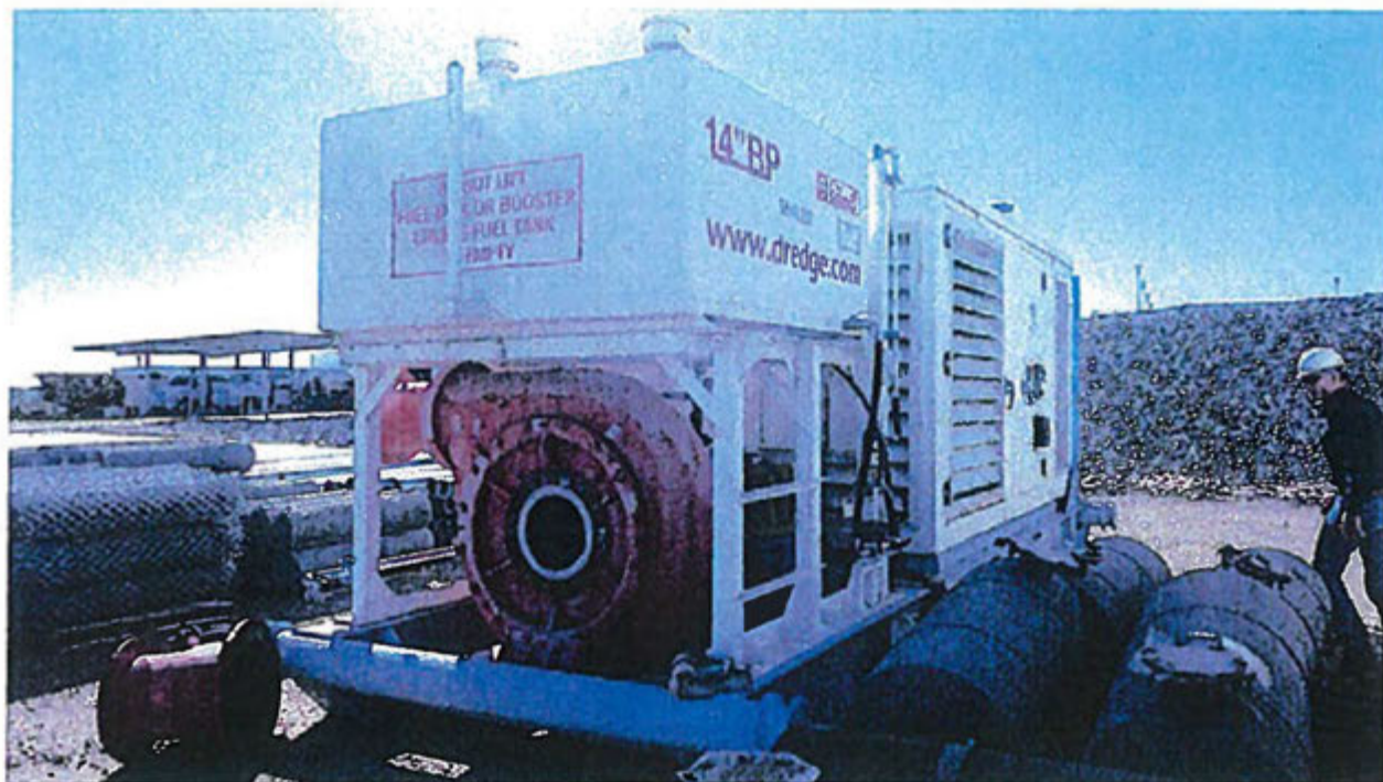
Photo 1 - Primary Ellicott 860 Booster Pump System with Diesel Engine
