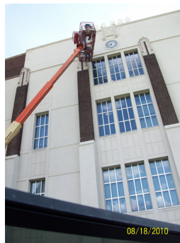
Sealing up West High School, former home to hundreds of Mexican free-tailed bats.
