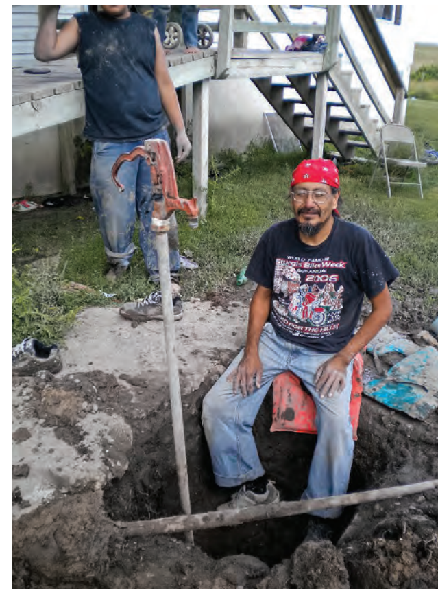
A local Pine River Reservation resident works on a pump to provide a house with well water.
