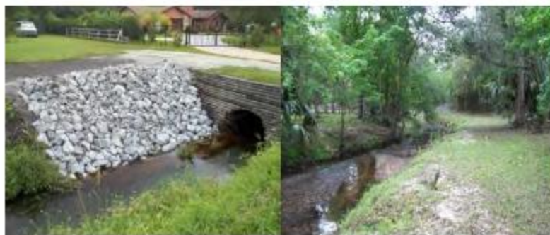
Tomoka Farms Roadside Ditch
