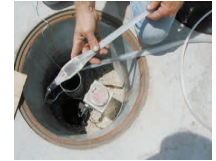
Interstitial monitoring sensor
