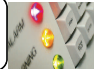
Control panel indicator lights
