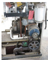
Suction piping system
