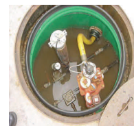
Tank top sump full of liquid
