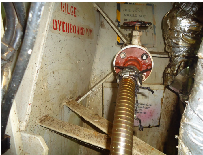
Bilge sent overboard with flexible hose.
