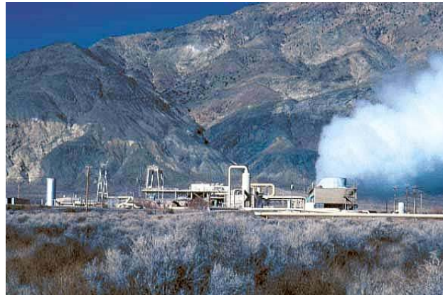
Figure B-8. Caithness Geothermal Power Plant in Dixie Valley, Nevada (source: BLM).
