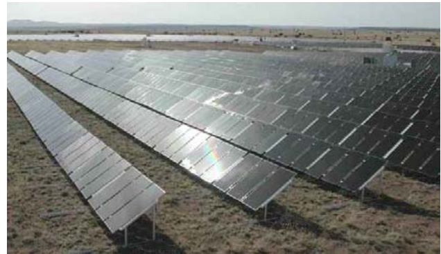
Figure B-6. 3.8 MW Springerville Solar Plant (source: First Solar).
