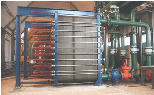
Figure C-5. Geothermal District Heating Equipment.
