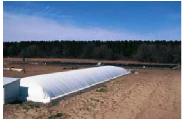
Figure C-9. 135 kW Dairy Manure Digester. 5
